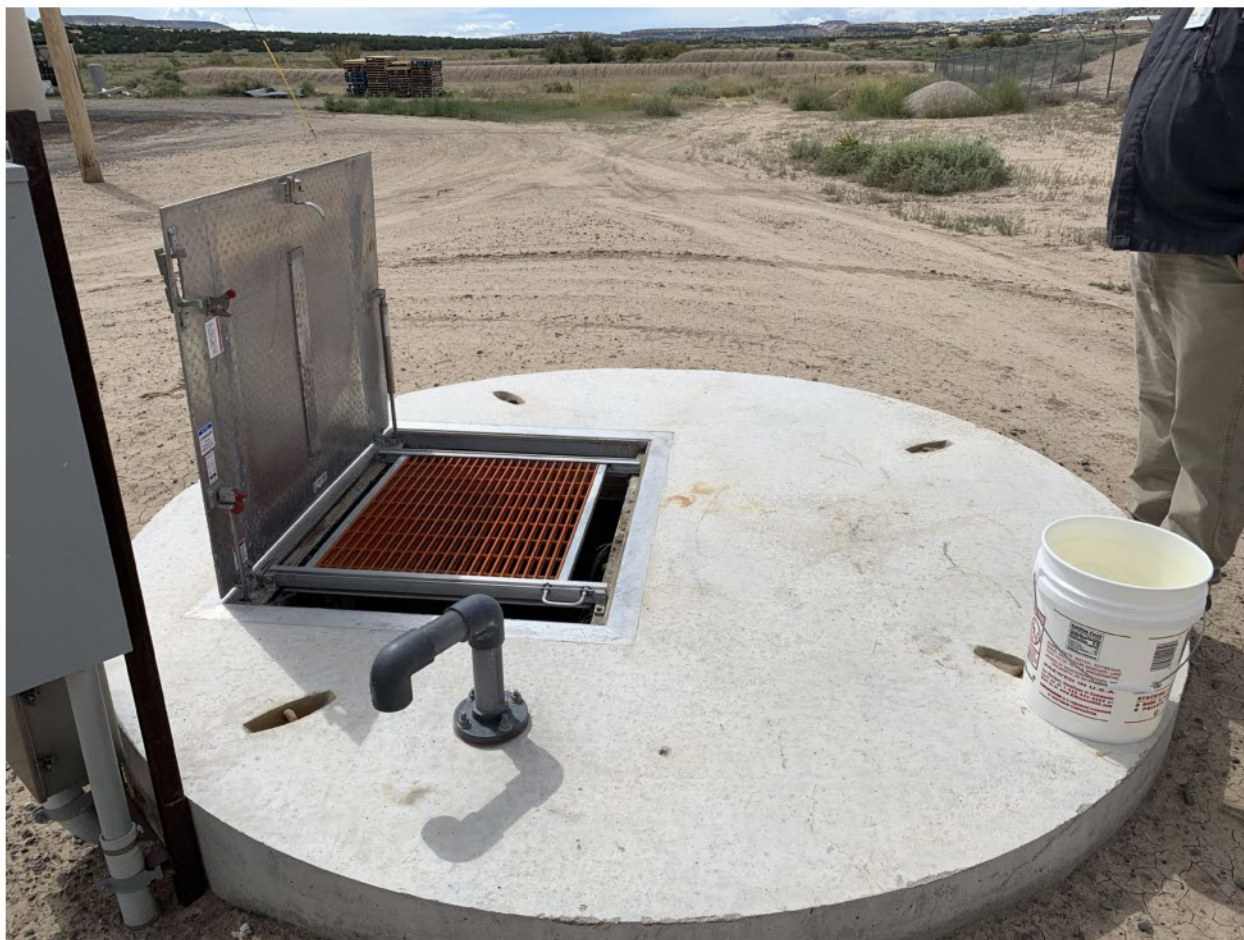
View of LS WWTP#1 with hatchway open and safety gate in-place. (IMG0138). September 13, 2022. Photographed by D. Esparza
