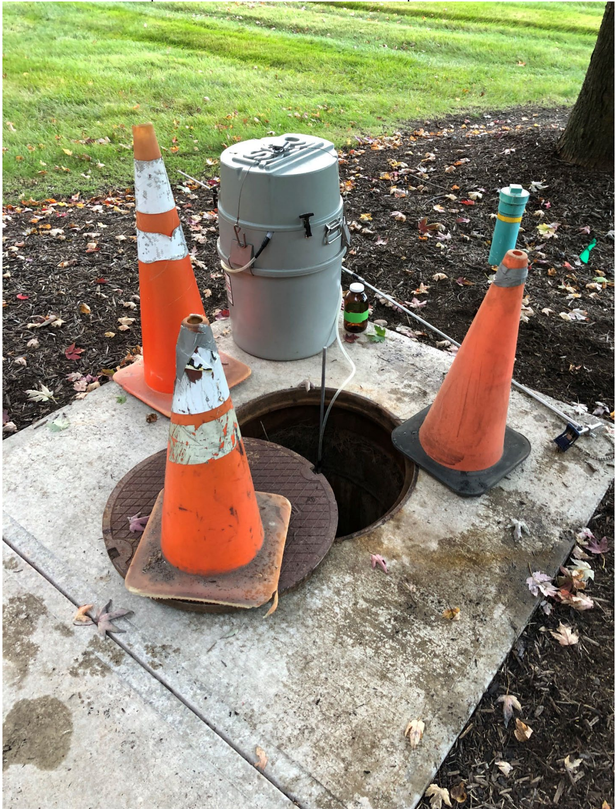
Photo #1: View of the pretreatment effluent location where samples were collected.
