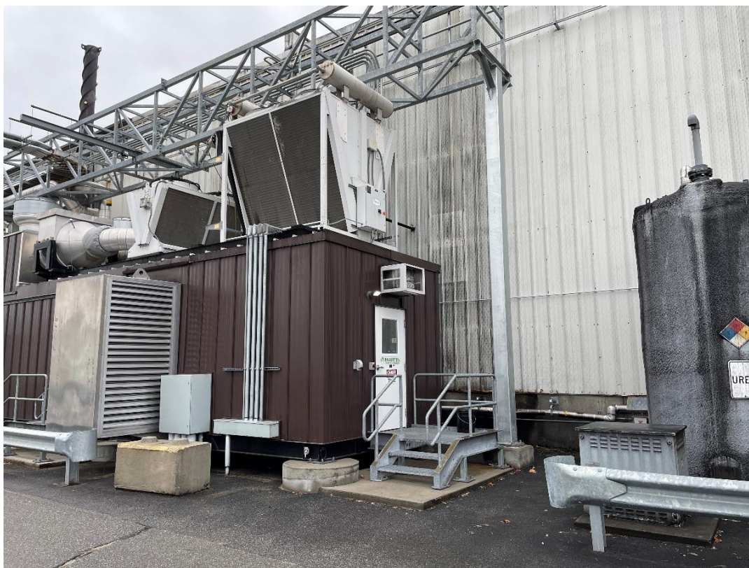
Photograph 1: Trailer housing the CHP.
