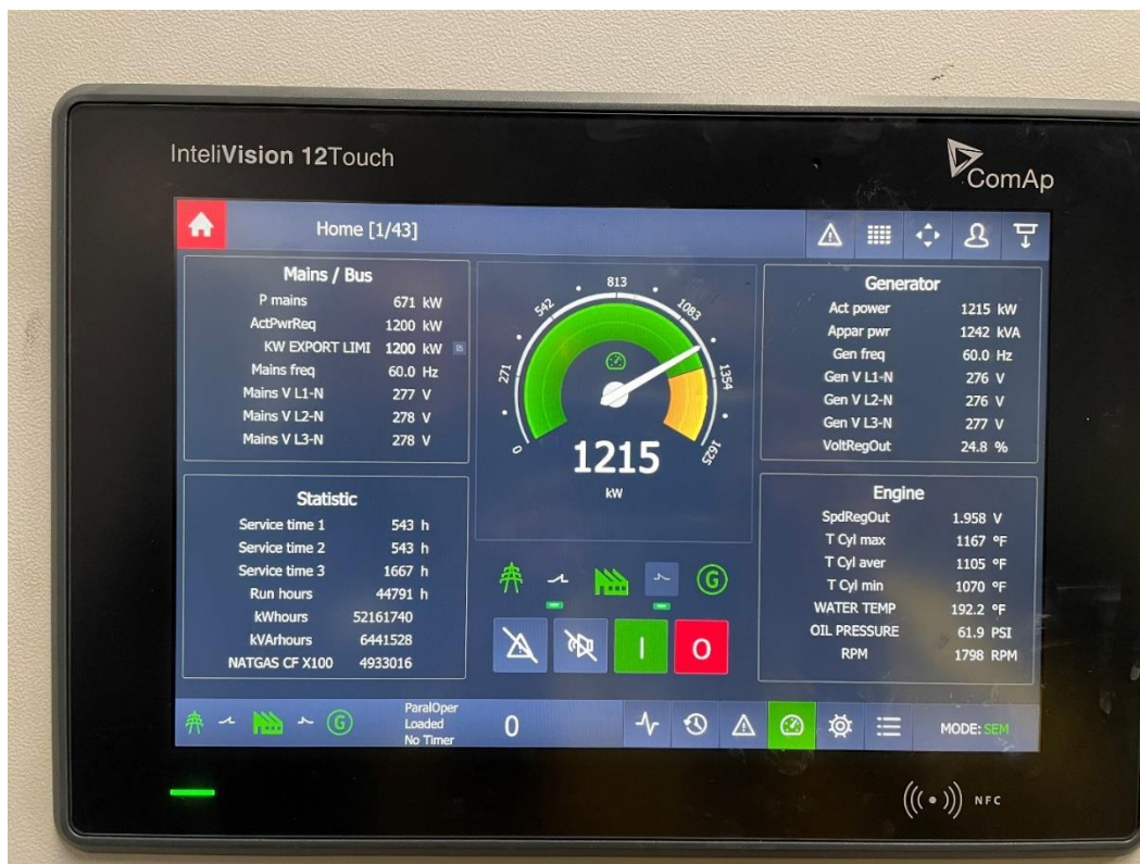
Photograph 3: Control system screen displaying the CHP engine operating parameters.
