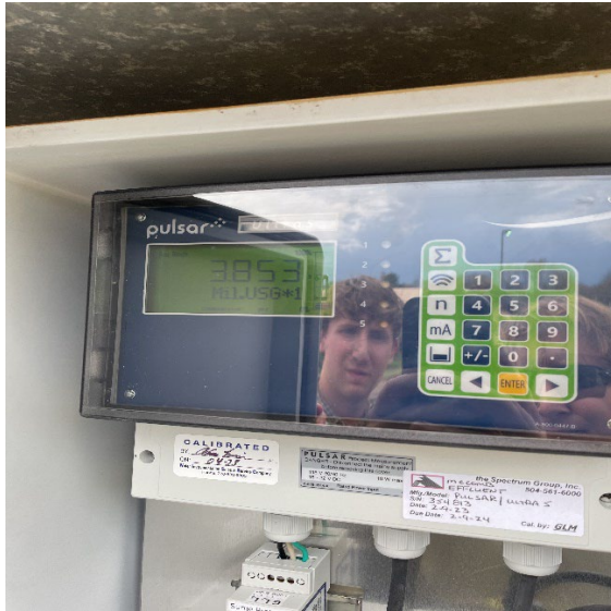
Figure 3 – Effluent Flow Meter
