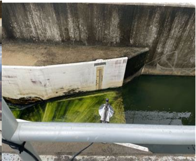
Figure 4 – Effluent Parshall Flume
