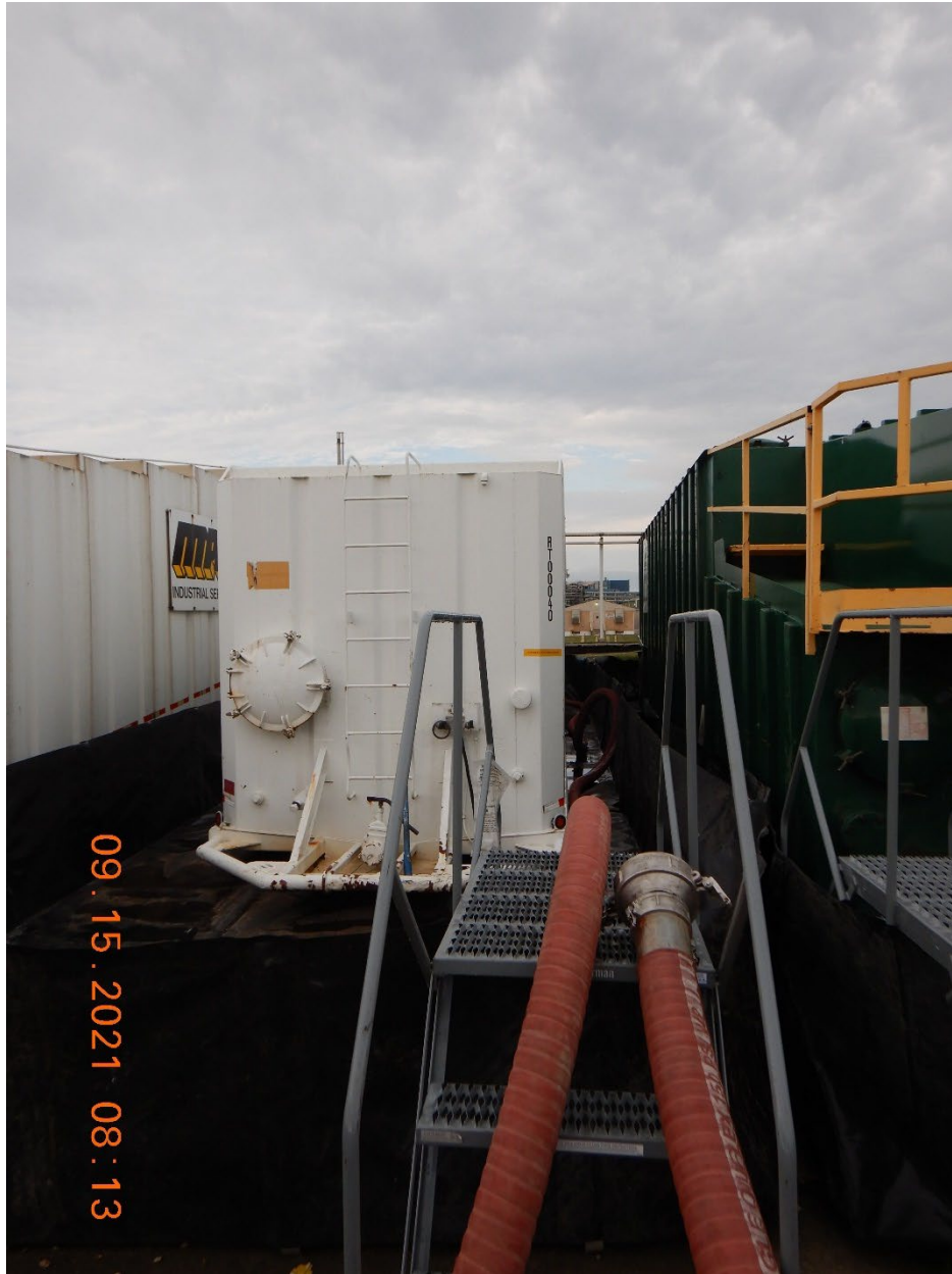
RCRA Photo 23. A view of frac tank RT00040 that was labeled with “Hazardous Waste – Pending Analysis” on the side of the tank.
