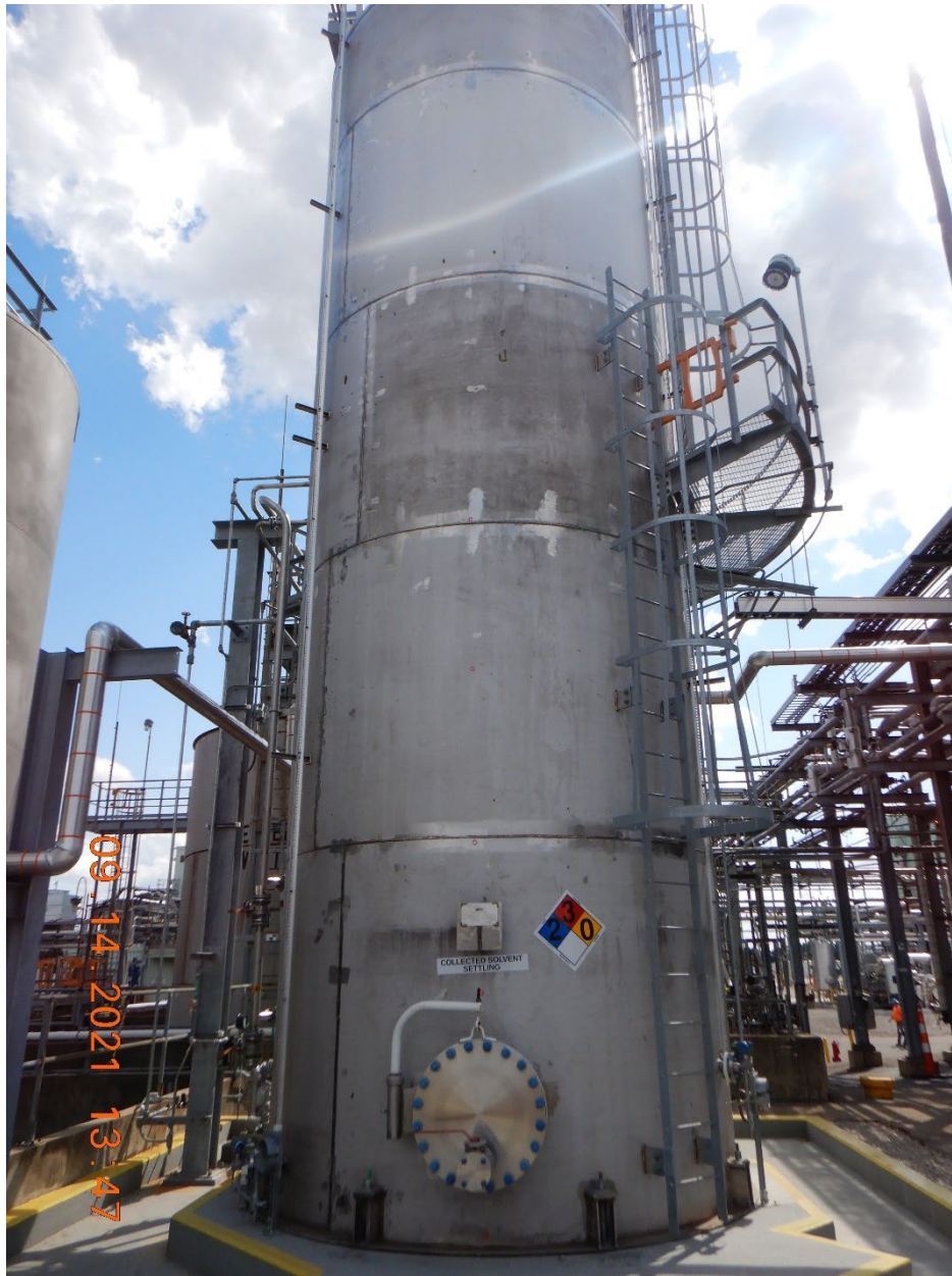
RCRA Photo 11. A view of the collected solvent settling tank located next to the Kapton solvent recovery process. The tank is used to hold material that is sent through the solvent recovery process.
