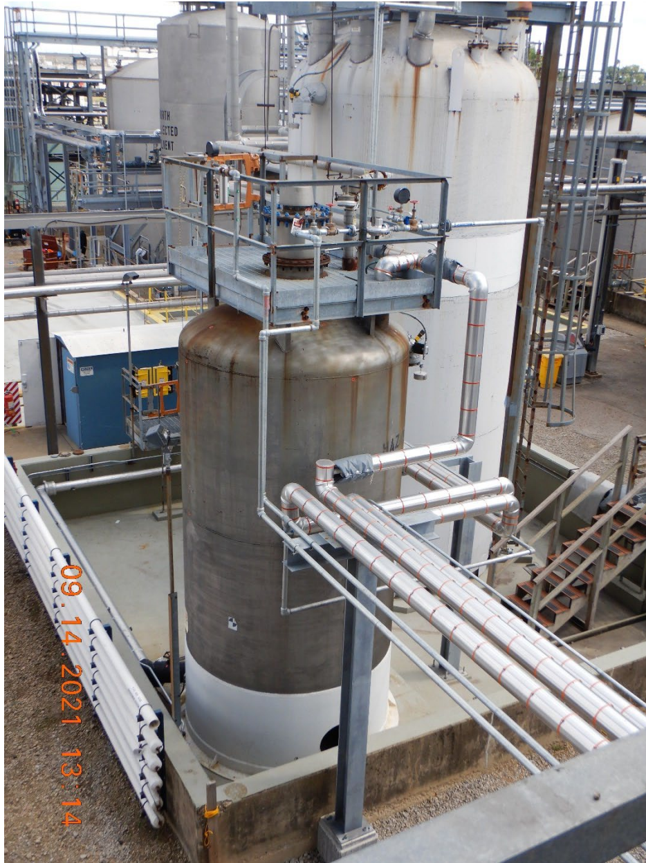
RCRA Photo 8. An overview of the facility's 5,000-gallon hazardous waste tank. This view of the hazardous waste tank is shown from the Kapton solvent recovery area.
