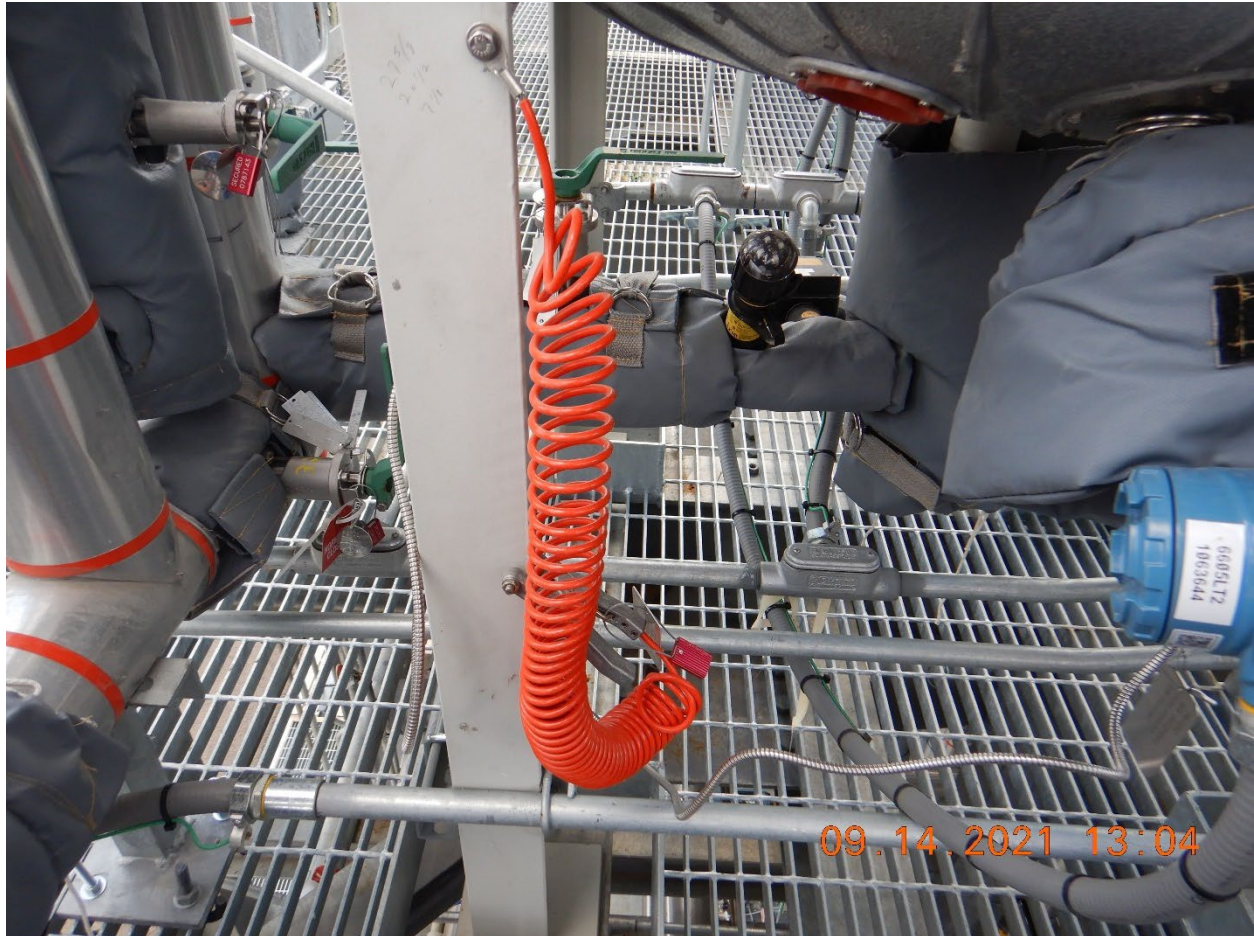
RCRA Photo 6. View of the lines underneath the P-12 decanter tank.
