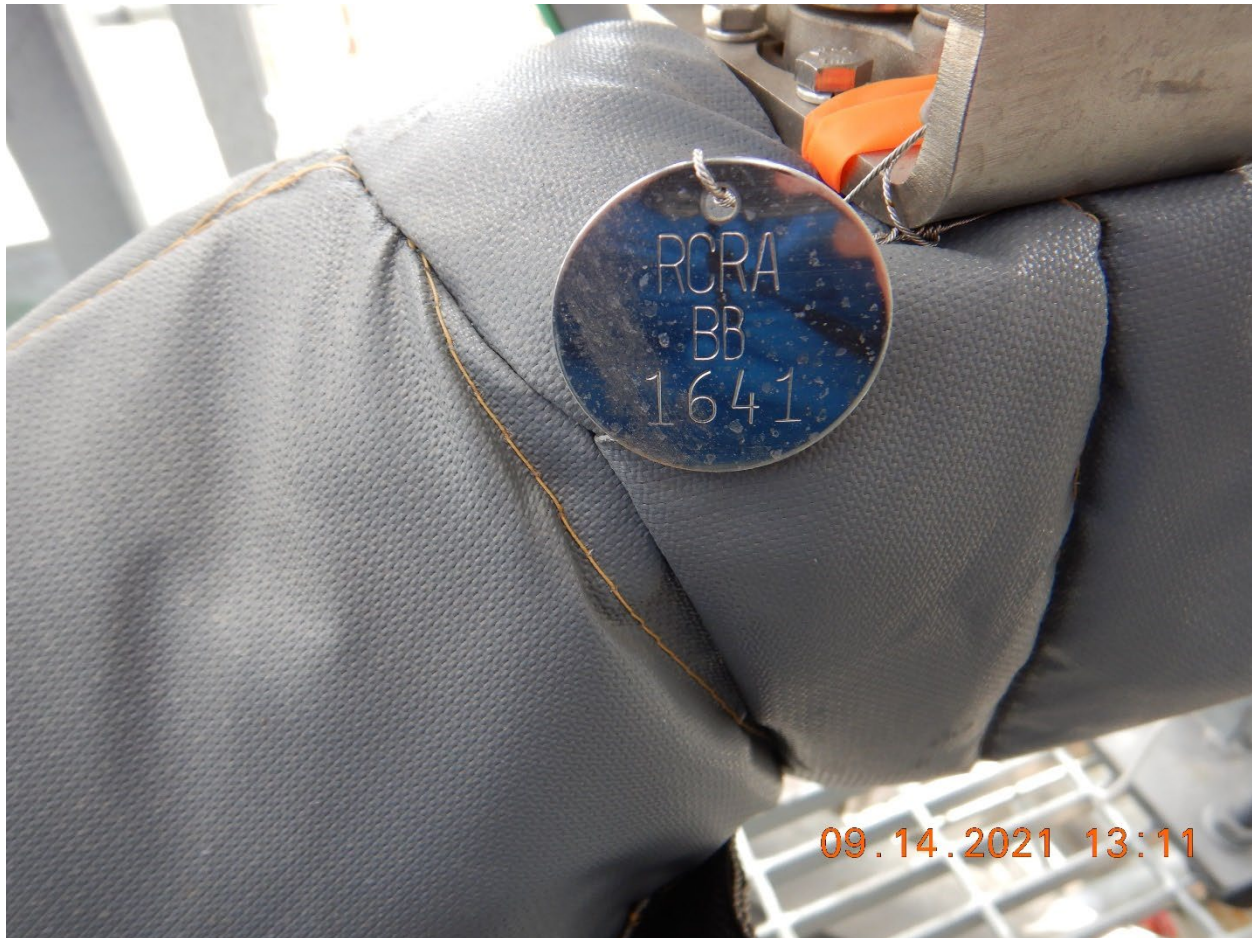
RCRA Photo 7. Close-up view of the lines underneath the P-12 decanter tank shown in Photo 6. This photo was taken to show an example of the facility's RCRA subpart BB tagging system.
