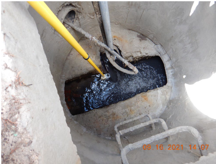
CWA Photo 35. View of sampling from the K2 process sewer.
