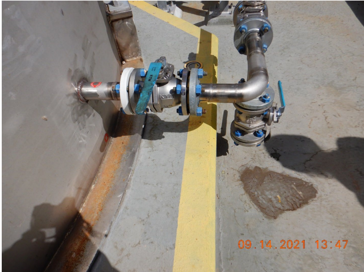
RCRA Photo 12. A view of the discharge port of the collected solvent settling tank. The tank is cleaned out approximately once per year and the material is put into a tanker trailer which attaches directly to the port photographed above.
