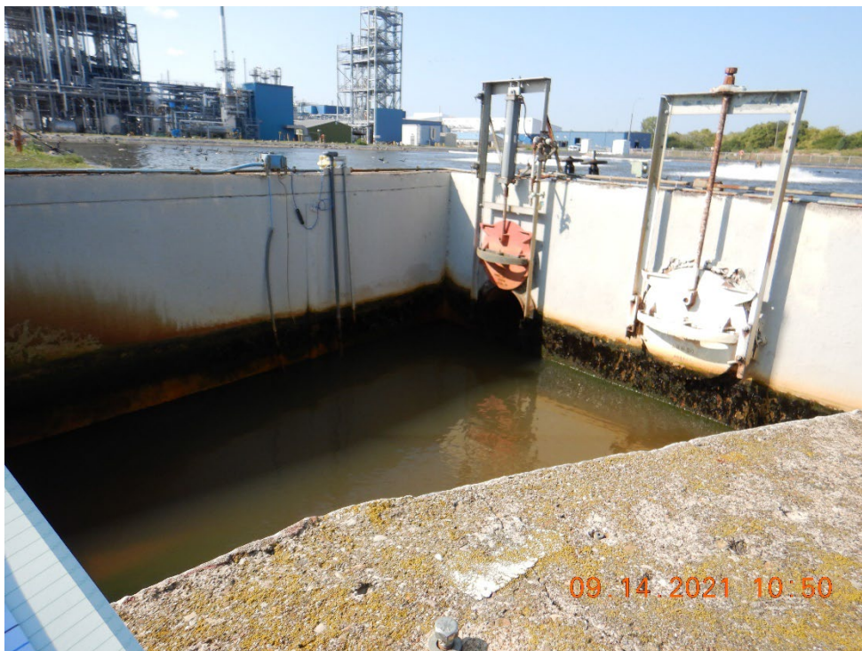
CWA Photo 14. View of the diversion box through which wastewater flows to the aerated lagoons. Wastewater was flowing through the left pipe at the time of the inspection, corresponding to the South Lagoon.
