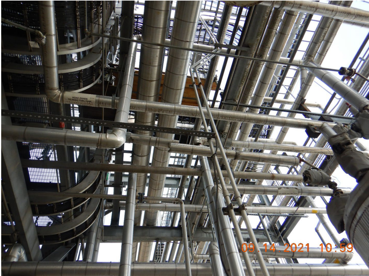
RCRA Photo 2. View of the lines that feed into the 2,200-gallon liquid fuel tank shown in Photo 1.
