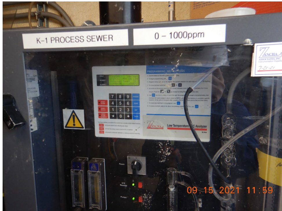
CWA Photo 3. View of the K1 TOC analyzer, which read 106 mg/l (ppm) at the time of the inspection on 9/15/2021.
