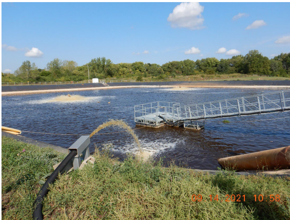
CWA Photo 12. View of the North Lagoon, which was not discharging to the South Lagoon at the time of the inspection. The hose viewed in the photo is a recirculation line.
