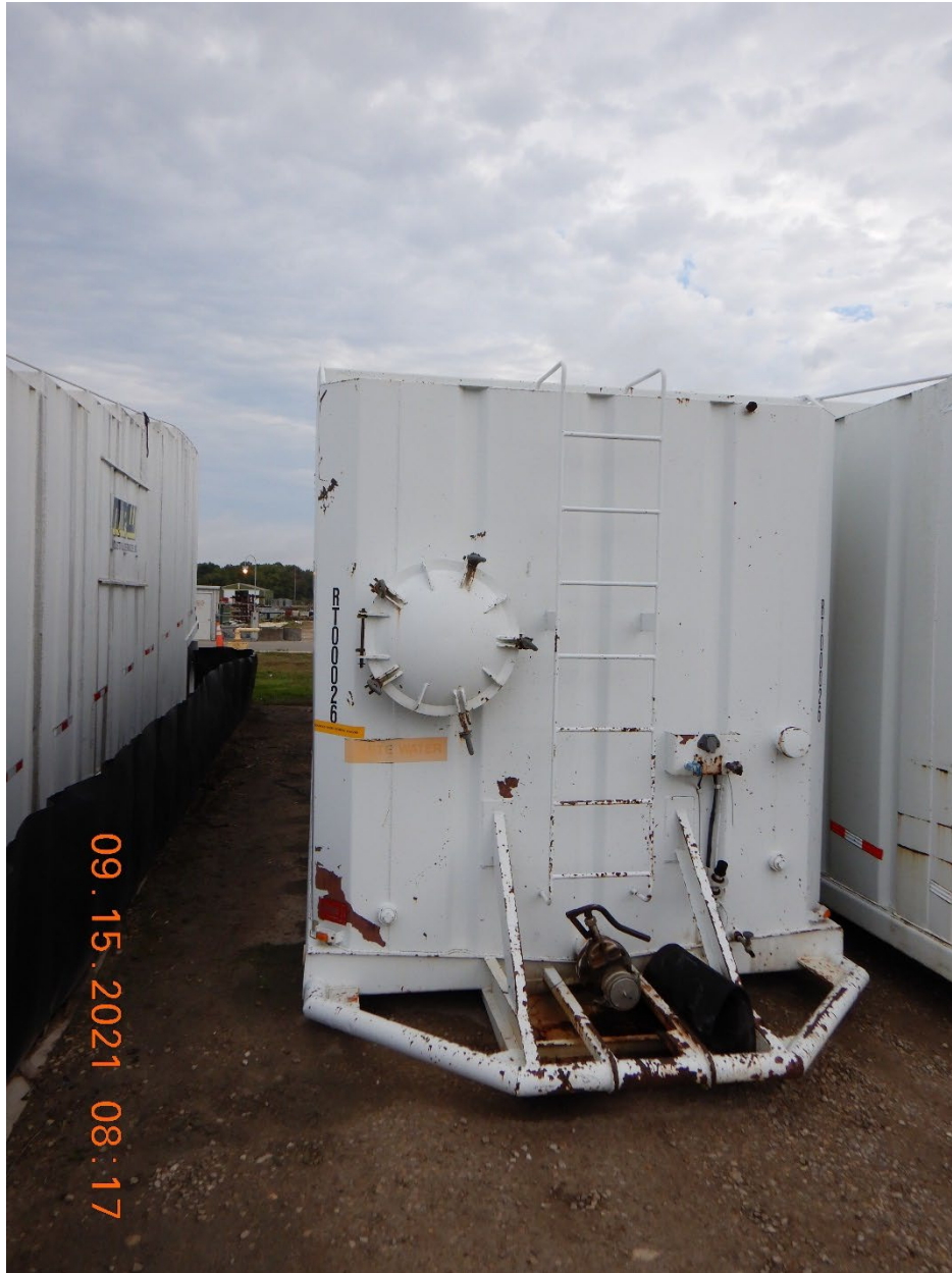
RCRA Photo 26. A view of frac tank RT00026 that was also labeled with “Hazardous Waste – Pending Analysis” on the side of the tank as seen on frac tank RT00040 in Photo 25.
