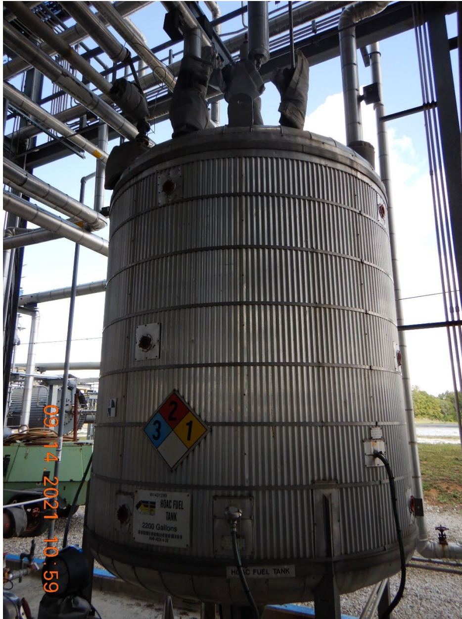
RCRA Photo 1. View of the 2,200-gallon liquid fuel tank located in the Kapton solvent recovery area.
