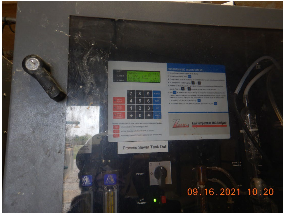
CWA Photo 7. View of the Tedlar process sewer tank TOC analyzer, which read 26 mg/l (ppm) at the time of the inspection on 9/16/2021.
