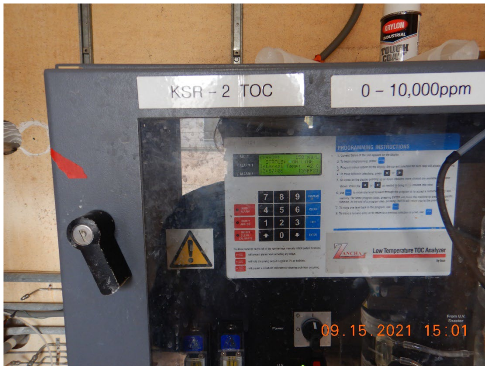
CWA Photo 2. View of the KSR2 TOC analyzer, which read 150 mg/l (ppm) at the time of the inspection. The time reading on this analyzer was off by approximately one hour.
