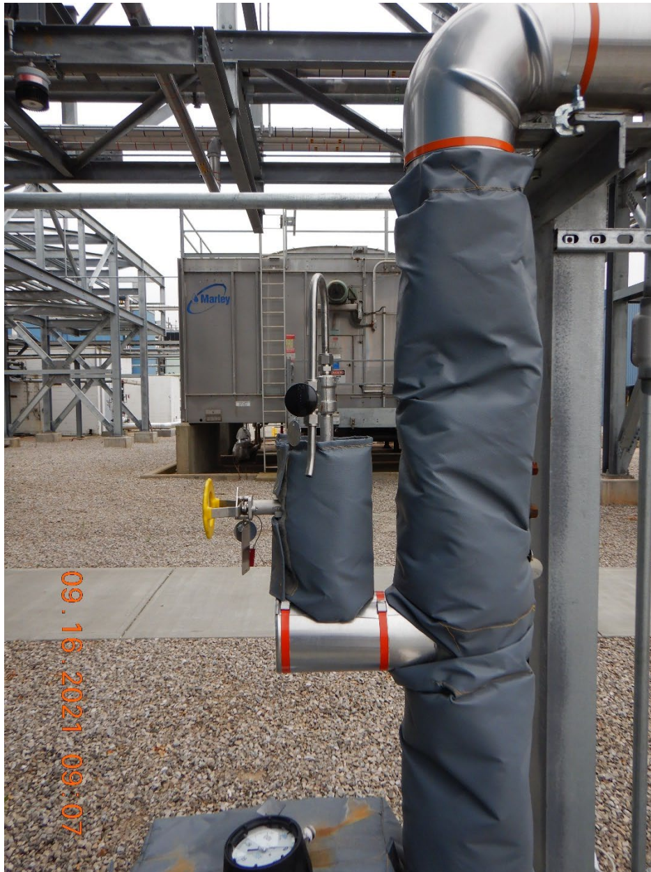
RCRA Photo 32. A view of the tap used to sample the basement tank located in the Vespel solvent recovery area. This sample tap was used to fill all SP-2 and SP-3 containers.
