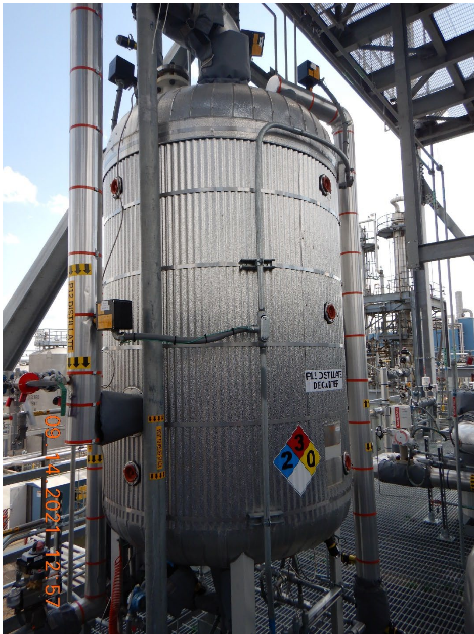
RCRA Photo 3. View of the P12 distillate decanter tank located in the Kapton solvent recovery area. The P12 decanter tank feeds the facility's 5,000-gallon hazardous waste tank shown in Photo 8.
