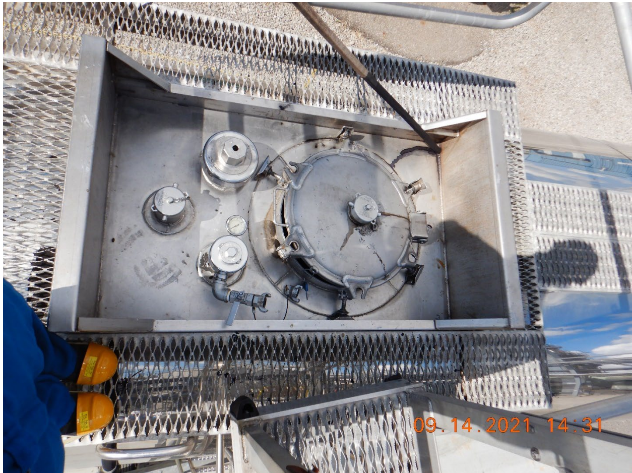
RCRA Photo 15. A view of the manway cover on the tanker trailer LT-1087 accumulating hazardous waste photographed in Photo 16. The manway cover was unlatched and venting to the atmosphere.
