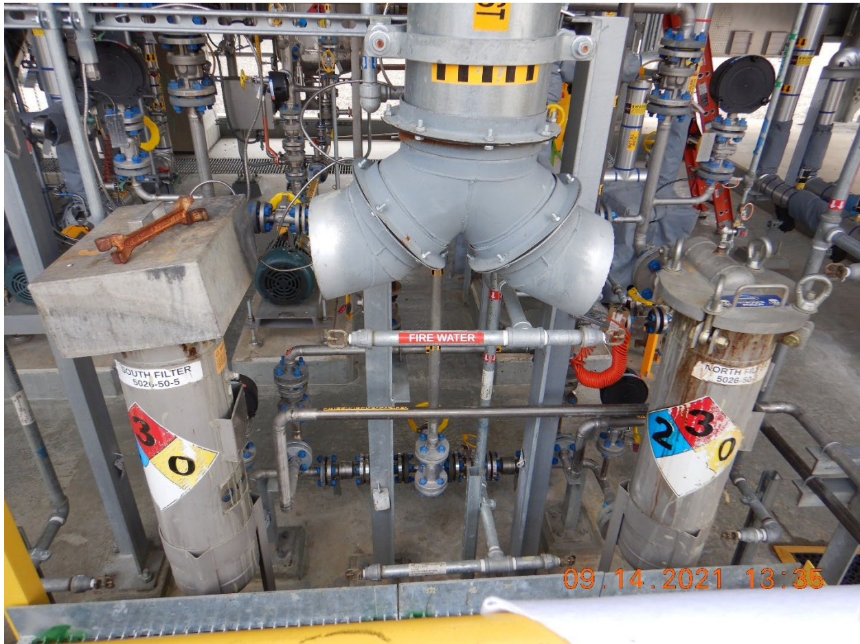
RCRA Photo 9. A view of both filters used in the Kapton solvent recovery process.
