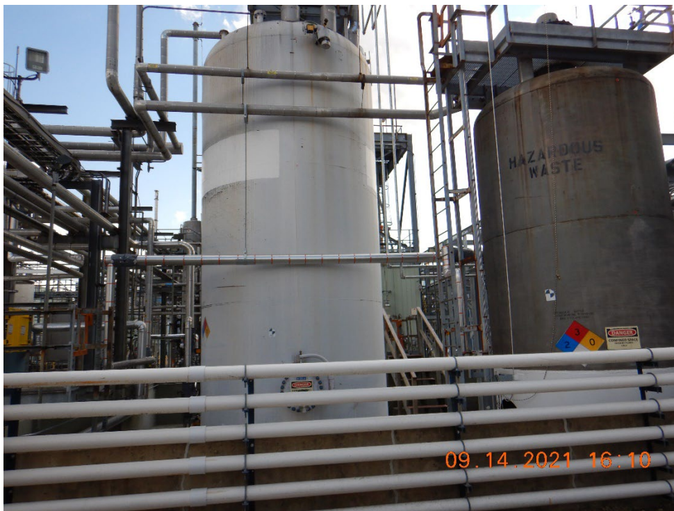
CWA Photo 10. View of the 20,000-gal wastewater tank that feeds the Vespel SBRs (white tank).
