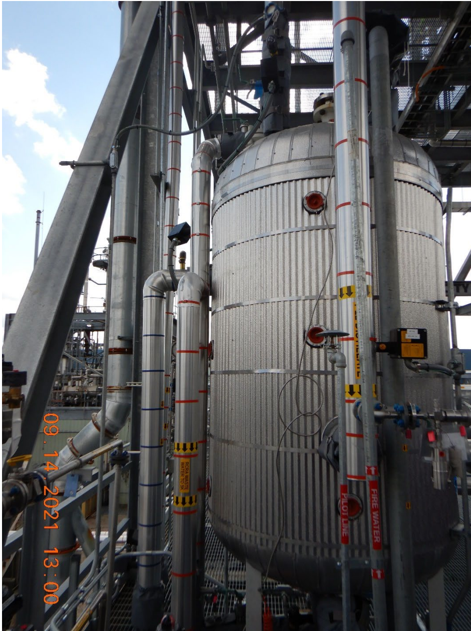
RCRA Photo 4. View of hazardous waste feeding lines coming off the P-12 decanter tank shown in Photo 3.
