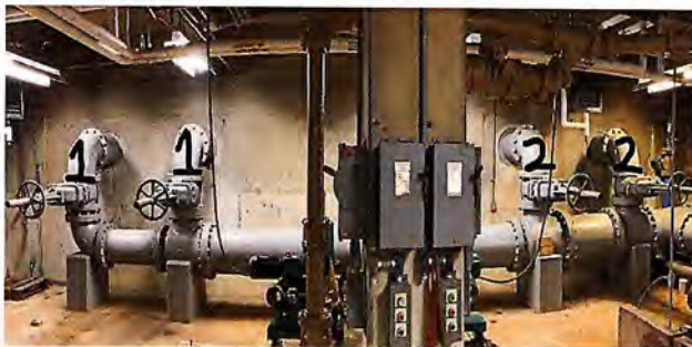
Primary Settling Tank #1 & #2 Influent Valves
