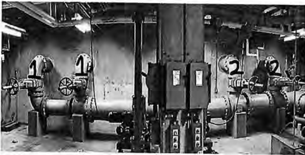
Primary Settling Tank #1 & #2 Influent Valves
