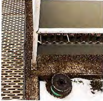
Primary Settling Tank #1 Drain Valve
