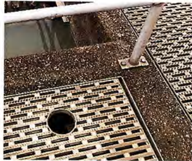
Primary Settling Tank #2 Drain Valve
