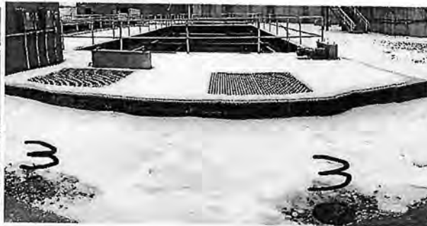
Primary Settling Tank #3 Influent Valves
