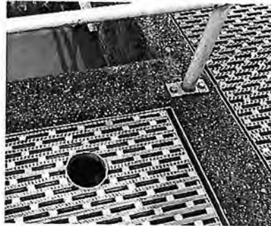
Primary Settling Tank #2 Drain Valve
