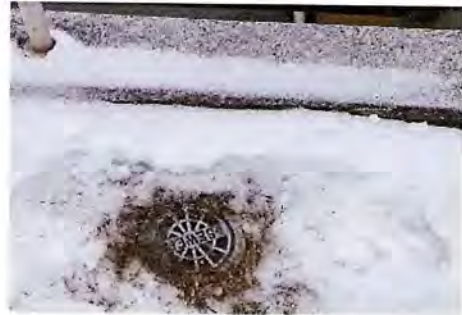
Primary Settling Tank #3 Drain Valve
