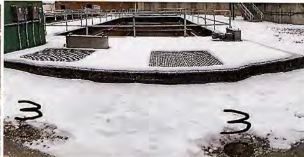
Primary Settling Tank #3 Influent Valves
