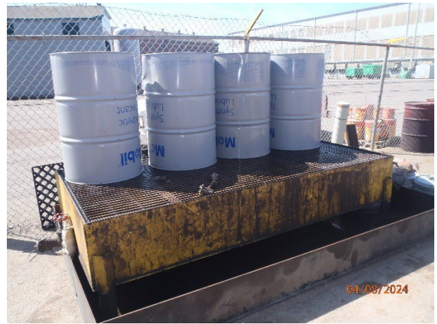
Picture 21 – Dry Dock 5 Pier F 90-Day CAA used oil drain station
