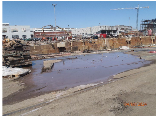
Picture 46 – Behind Condos paint slurry on the ground
