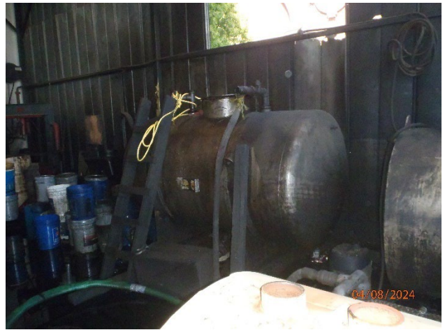
Picture 67 – Building 177 Maintenance Department used oil tank
