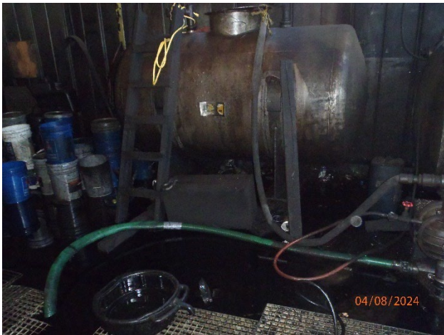
Picture 65 – Building 177 Maintenance Department used oil release to ground
