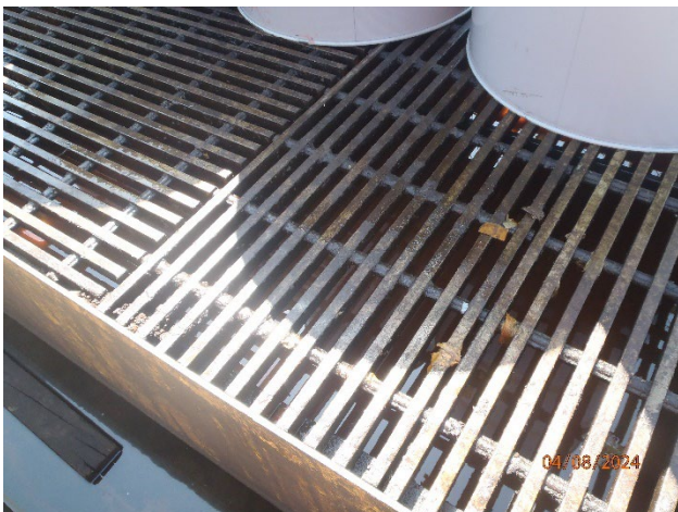
Picture 26 – Dry Dock 5 Pier F 90-Day CAA used oil drain station grate full
