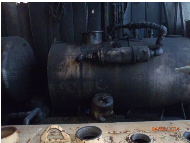
Picture 66 – Building 177 Maintenance Department used oil tank
