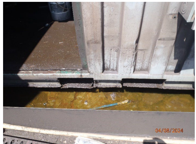
Picture 47 – Behind Condos compressor used oil
