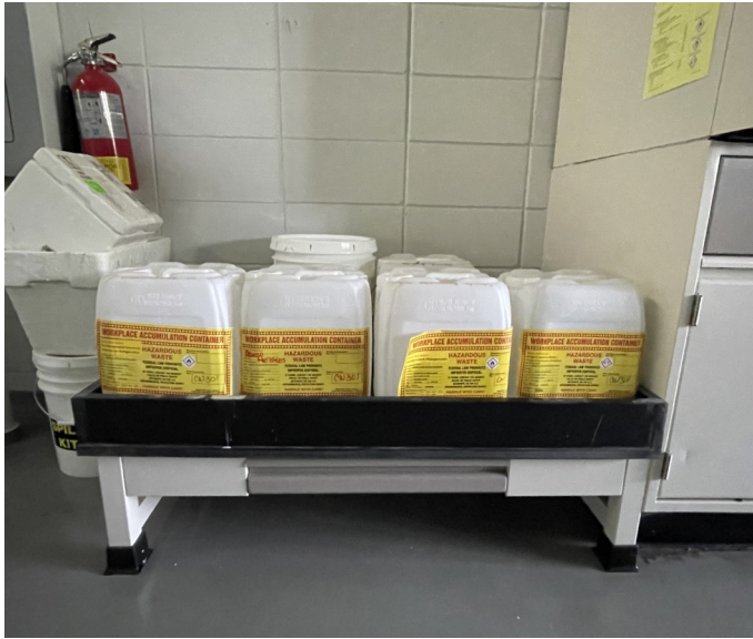
Picture 21 - UPR NATURAL SCIENCES - At the Lab CN-301, EPA Inspector noted that containers were in good conditions and sealed to secure of any potential releases of waste content, however, some containers were not properly identified nor posted with their hazardous communication pictograms.
