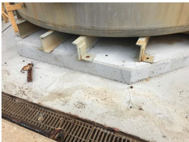
Photo 55: Cracks in secondary containment near Slurry Tank TK-5210.
