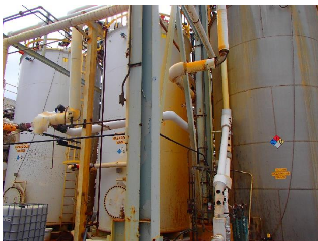
Photo 50: Three Slurry Tanks.
