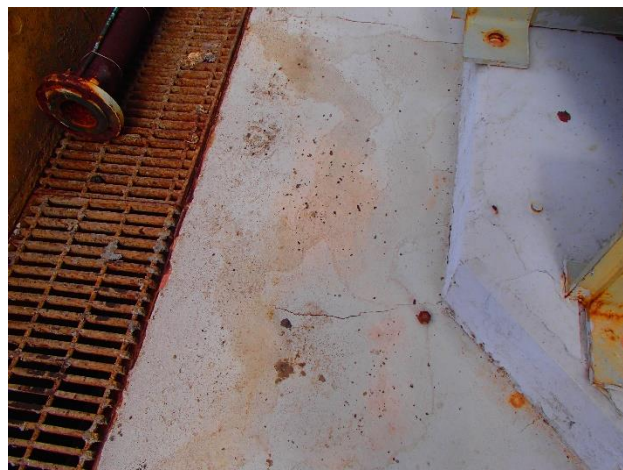
Photo 57: Cracks in secondary containment near Slurry Tank TK-5210.
