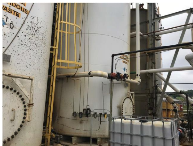
Photo 52: Slurry Tanks TK-5209B.
