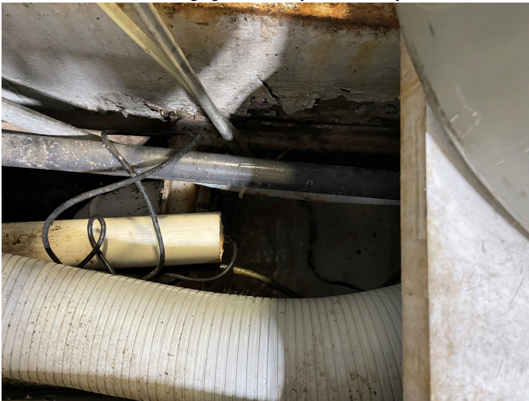
Photo #2. RO backwash was discharging continuously into the Sample Box.
