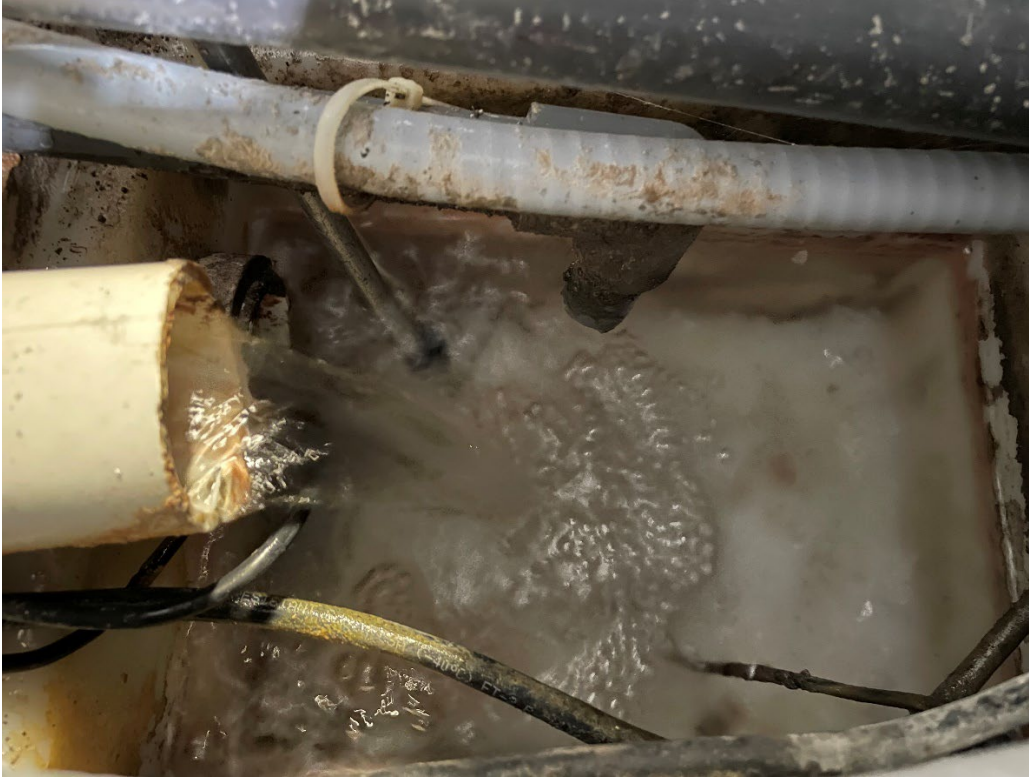
Photo #3. Discharge of pretreated effluent was intermittent into the Sample Box (grey pipe).
