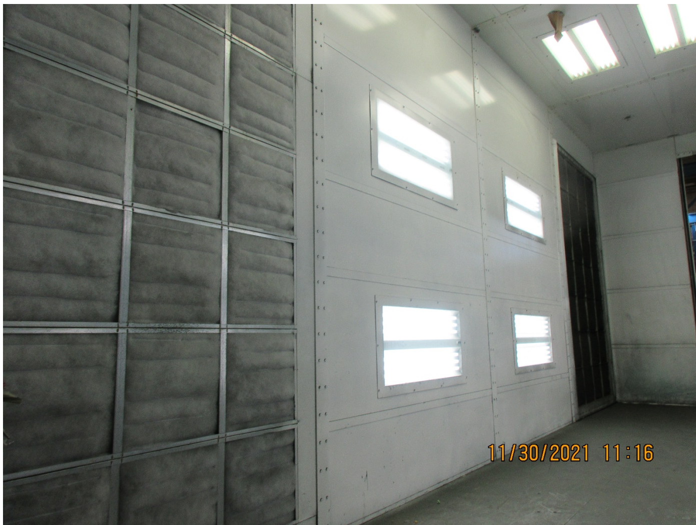
Photo 10 – Inside of prime coat paint booth.
