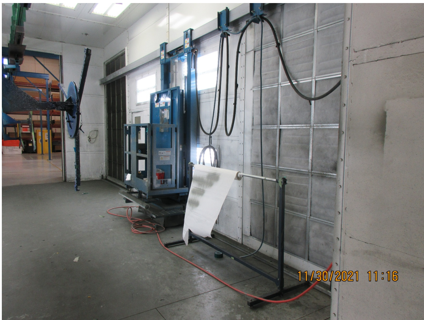
Photo 9 – Inside prime coat paint booth.
