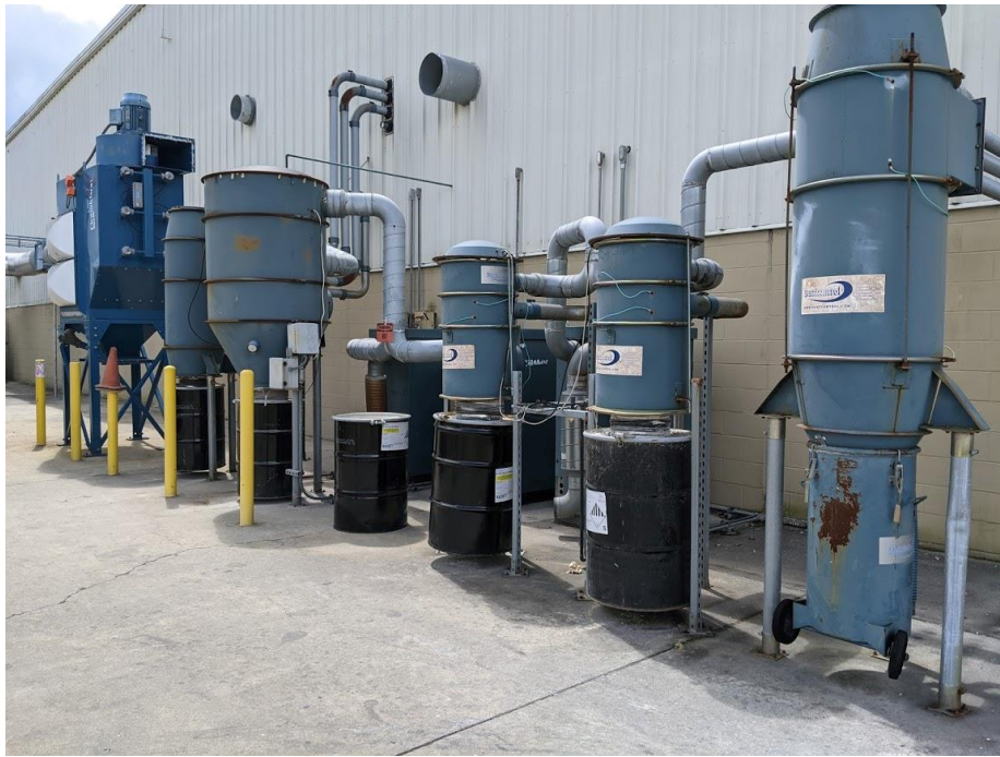
Photograph 3 of 3: Hazardous Waste Blast Media Collection Area
