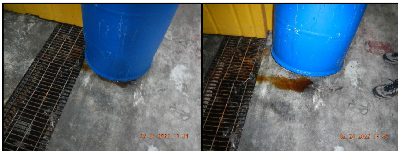
Figure 12. Bulk Chemical Drum With Oily Fluid Draining to the Trench System
