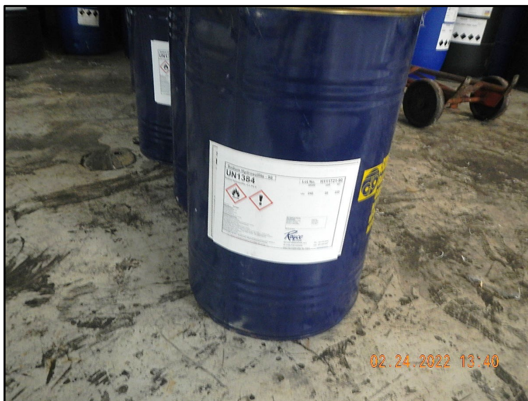
Figure 16. Un-bermed Bulk Chemical Storage Area – Drums Containing Warnings
