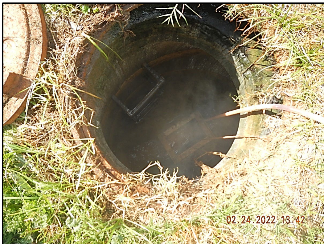
Figure 18. Monitoring Point Manhole – Vapor
