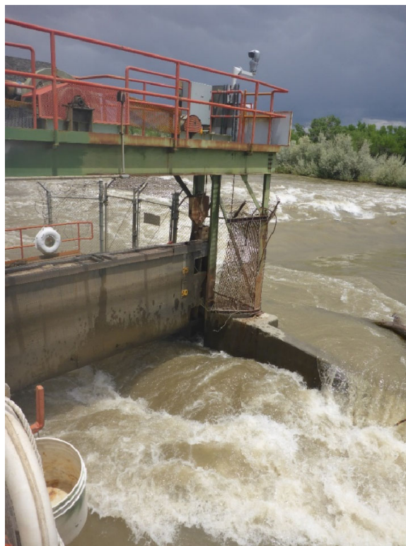
Photo 2 : Cooling water intake structure in the San Juan River.
