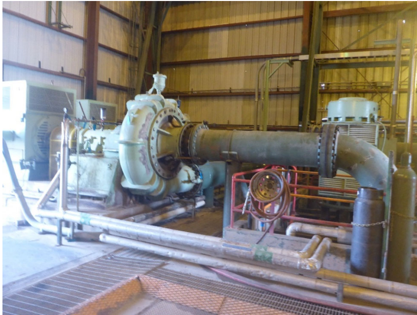
Photo 1 : River station pump gallery.
