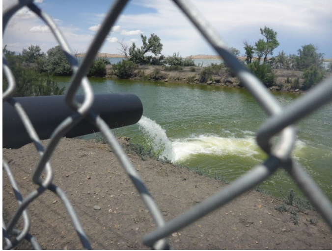
Photo 7: Discharge of condenser cooling water to the Canal.
