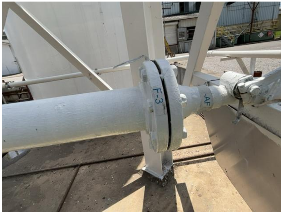
Photo 18 – BB equipment tagging on the hazardous waste tank equipment
