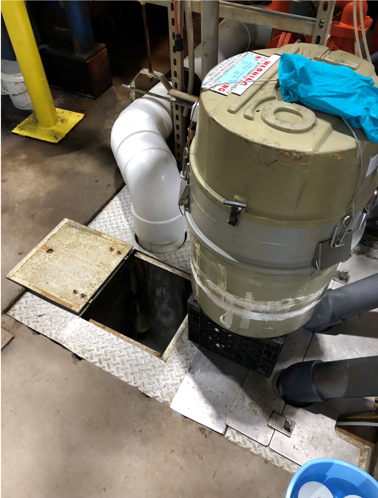
Photo #1: View of the pretreatment discharge location for Outfall 001.
