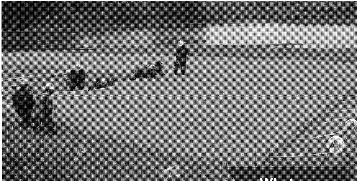
In-channel CCS cap pilot technology installed at Reach J in 2010. Information gained from the pilot about the implementability and effectiveness of the cap was used to inform future cap projects.
