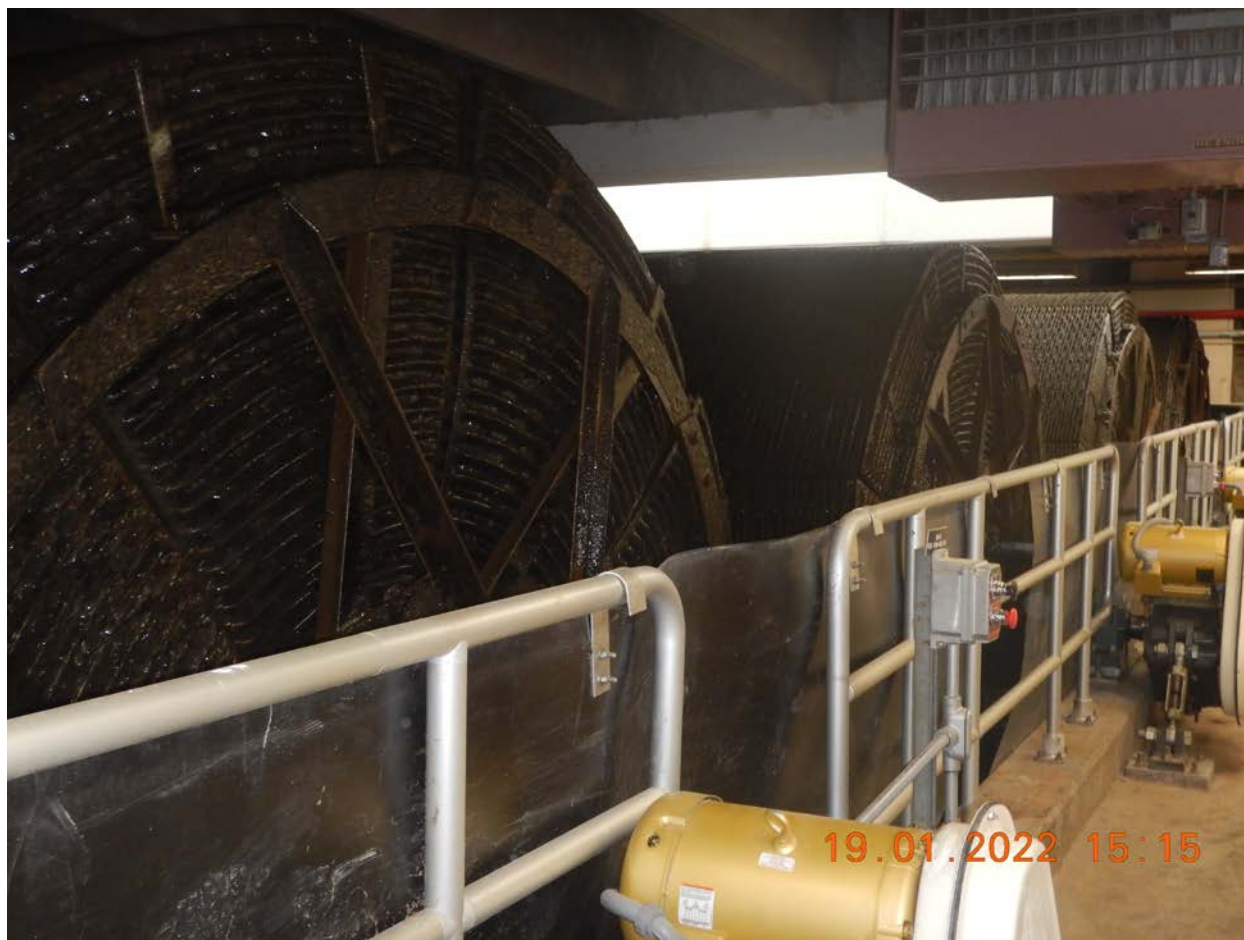
View of the three (3) trains of Rotating Biological Contactors (RBCs): one (1) for biological oxygen demand (BOD) removal and two (2) for ammonia removal. (DSCN 2102). Photographed by D. Esparza
