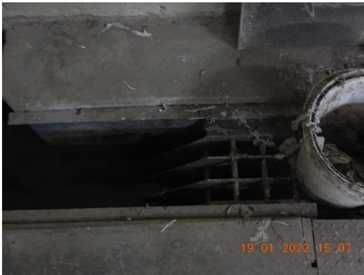
Another view of the headworks comprised of a bar screen/grit removal system. (DSCN2099). Photographed by D. Esparza
