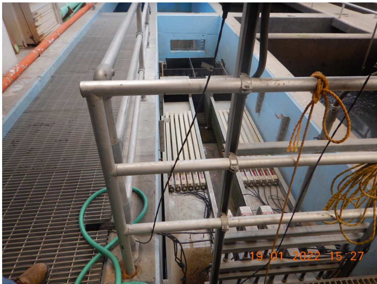
View of the three (3) parallel ultraviolet (UV) disinfection banks. (DSCN 2107) Photographed by D. Esparza
