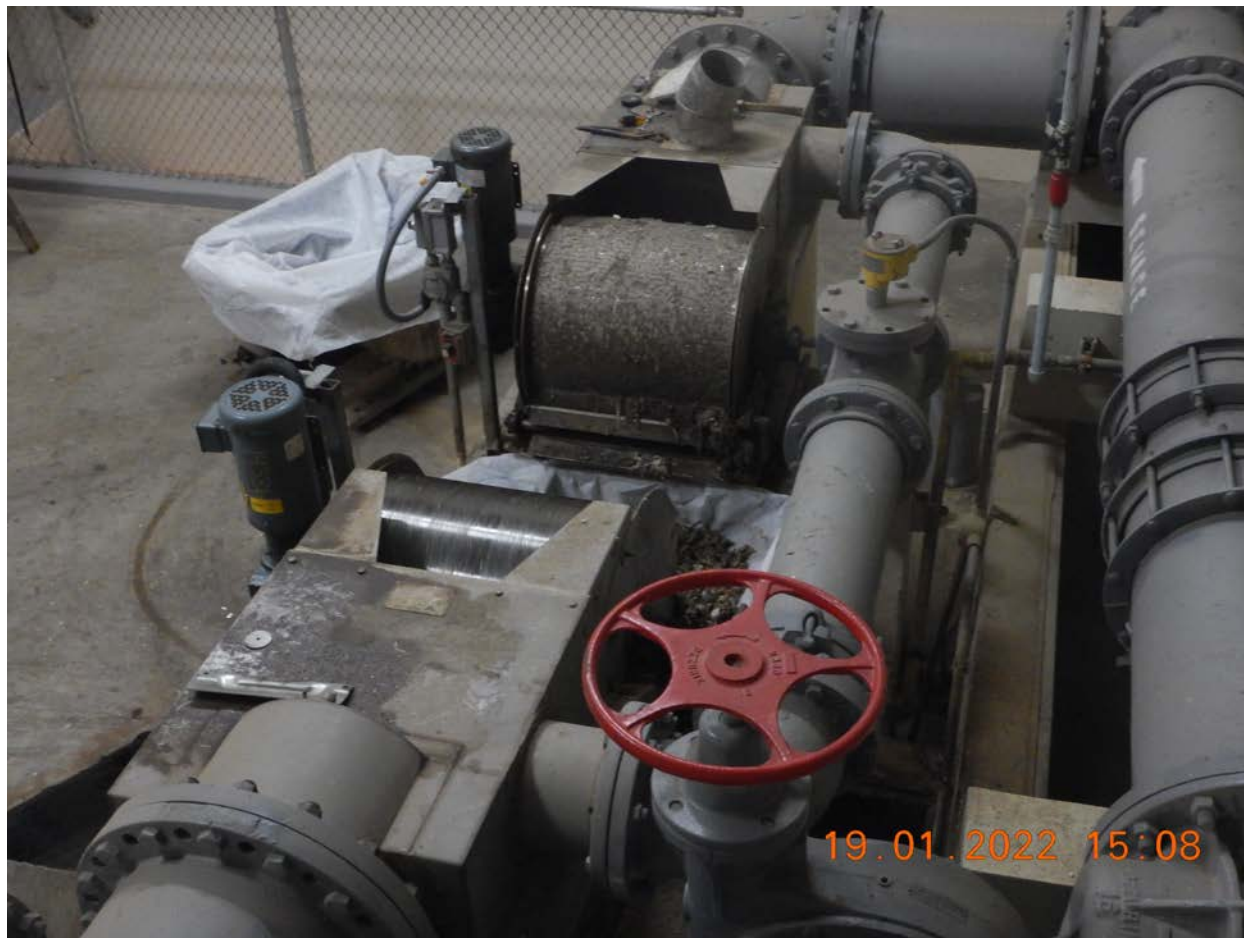
Another view of the screened fine mesh filter. (DSCN2100). Note: one (1) mesh filter is currently off-line awaiting repair and/or maintenance. Photographed by D. Esparza
