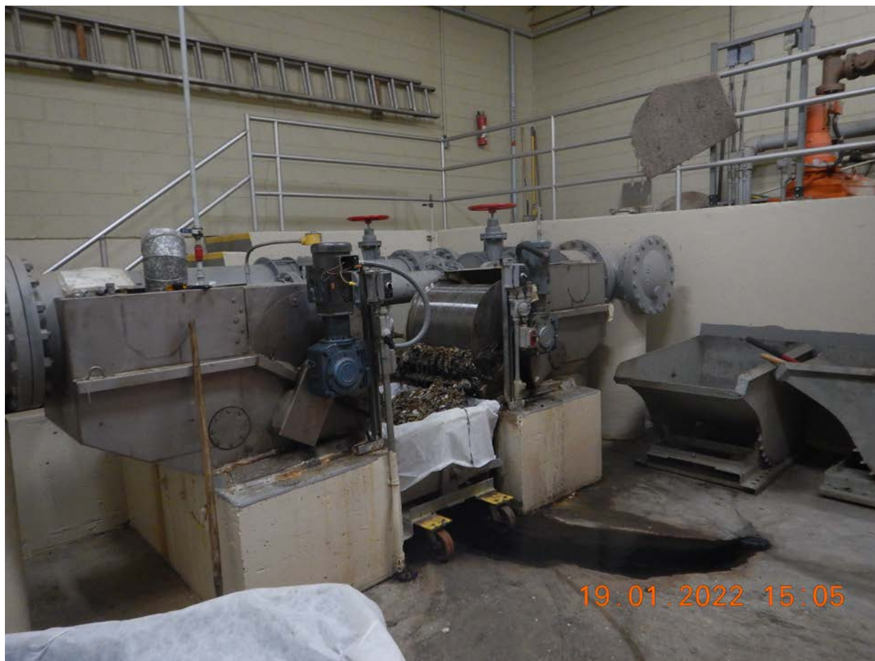
View of the screened fine mesh filter. (DSCN2097). Note: one (1) mesh filter is currently off-line awaiting repair and/or maintenance. Photographed by D. Esparza
