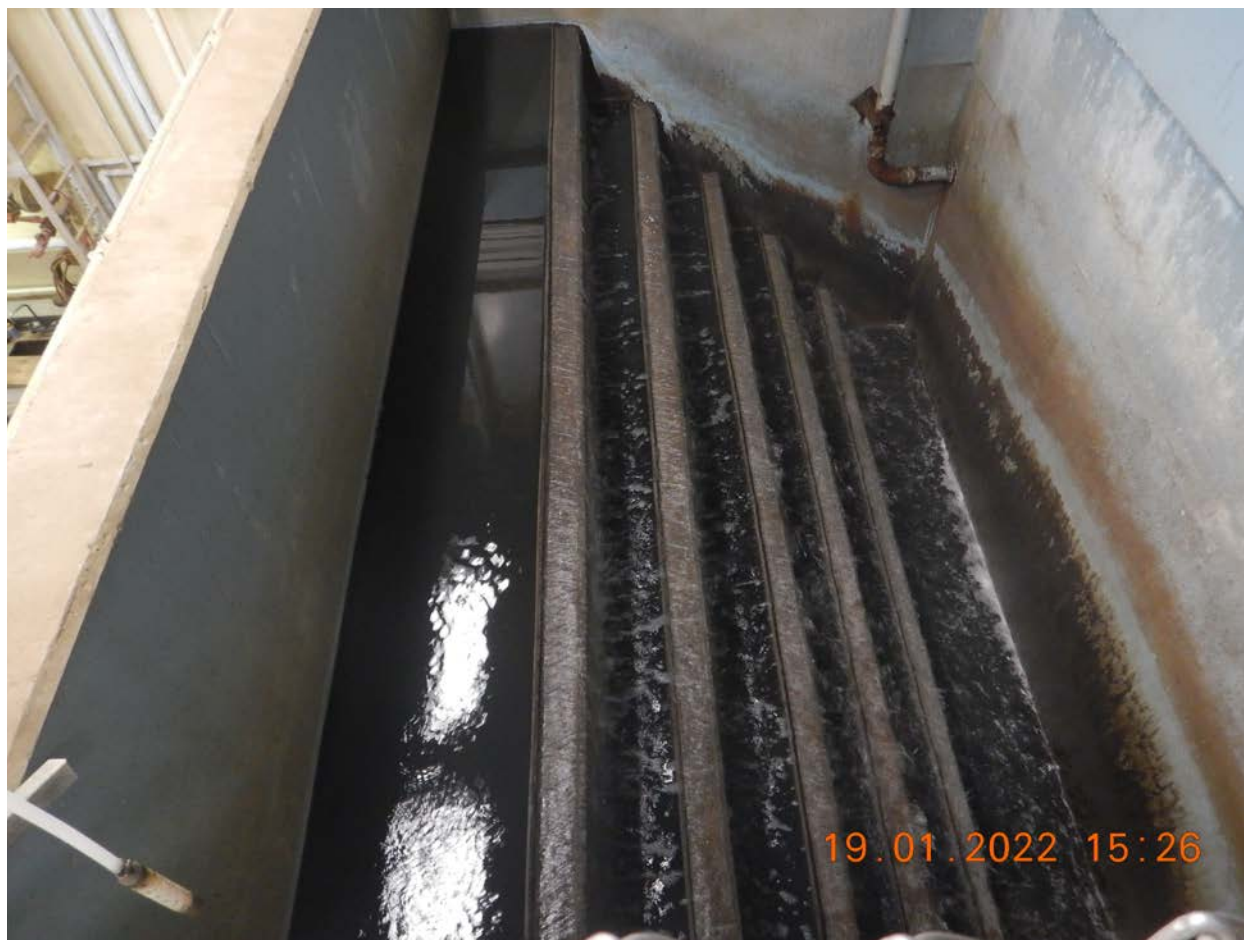
View of the disinfected effluent as it traverses over a stepped cascade structure prior to discharge to the Red River via a closed conduit pipe. (DSCN 2106) Photographed by D. Esparza
