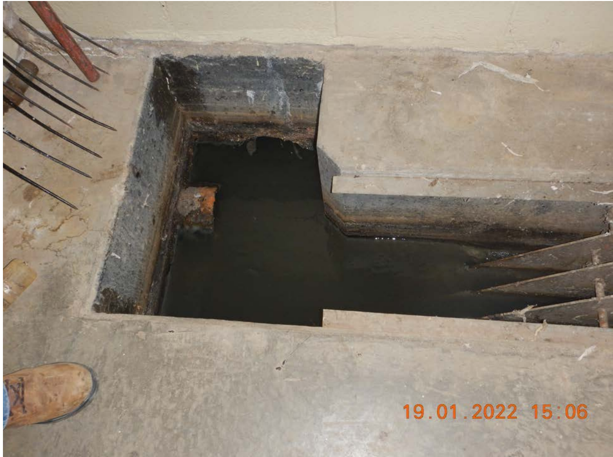
View of the headworks comprised of a bar screen/grit removal system. (DSCN2098). Photographed by D. Esparza
