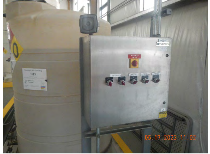
Photo #:18 (DSCN3289) Description: Photo within the cogeneration boiler condensate treatment system building.
