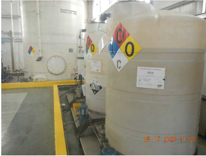
Photo #:17 (DSCN3288) Description: Photo within the cogeneration boiler condensate treatment system building.
