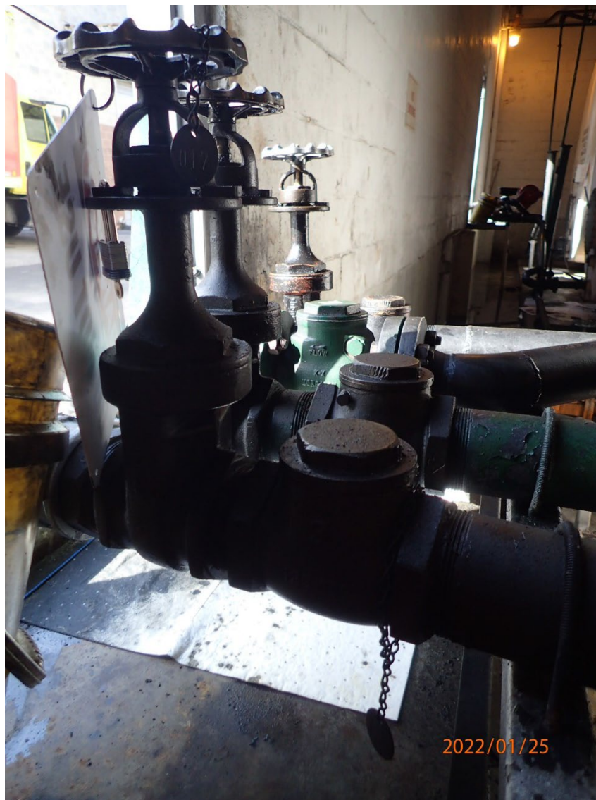
Photo 13: The waste solvent AST lines and associated equipment (flanges, pumps, valves, and, end caps) are inspected daily for leaks and are tagged as required by 40 CFR 264 Subpart BB.
