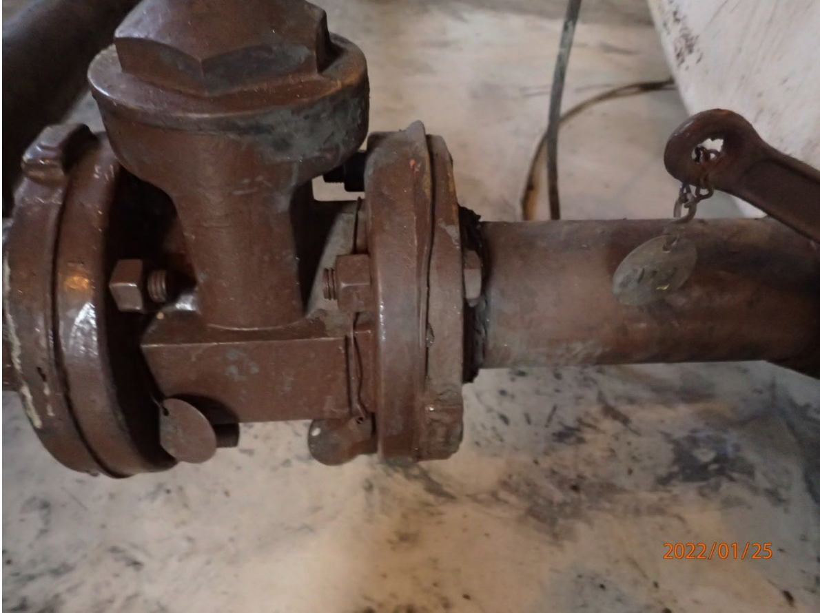
Photo 12: The waste solvent AST lines and associated equipment (flanges, pumps, valves, and, end caps) are inspected daily for leaks and are tagged as required by 40 CFR 264 Subpart BB.
