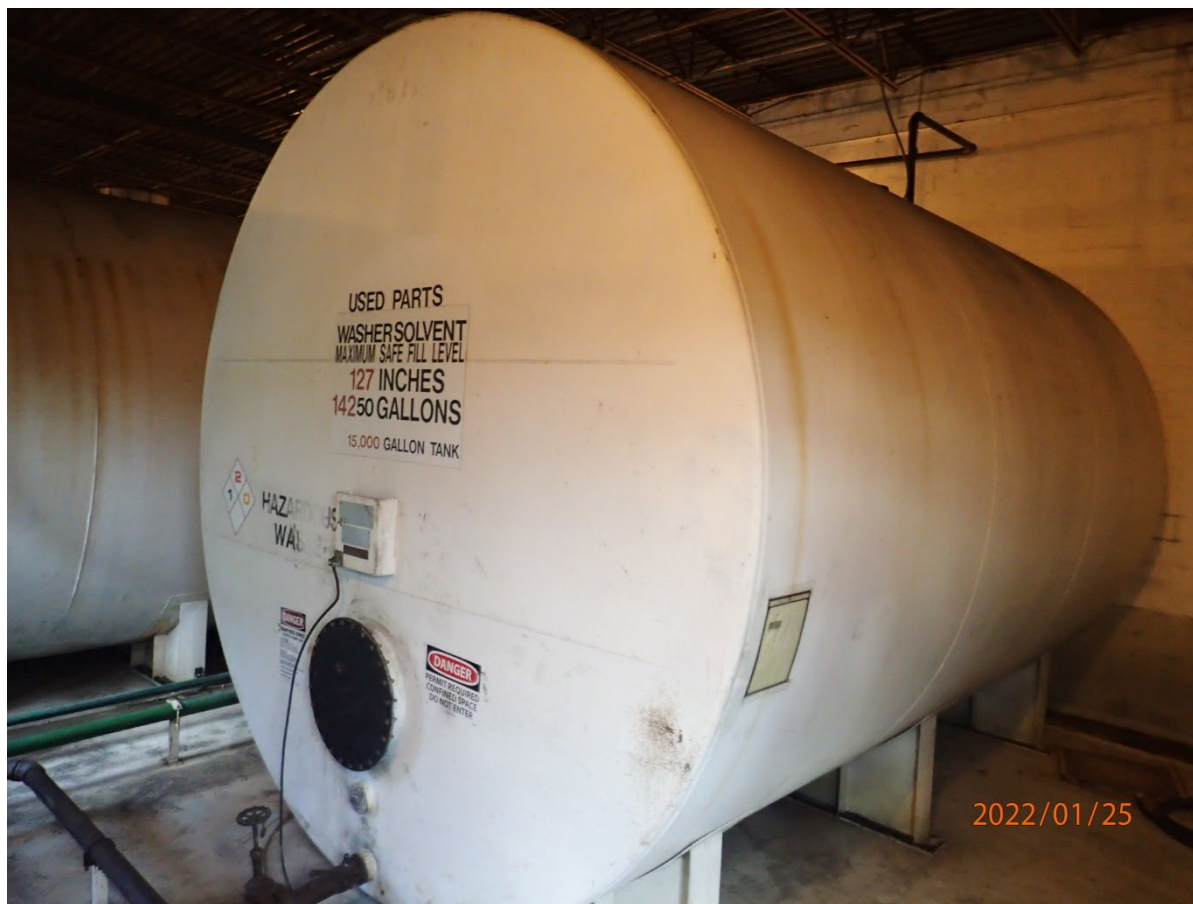
Photo 11: One (1) 15,000-gallon permitted AST for waste solvent, labeled with the words “Hazardous Waste”, and marked with a NFPA diamond as an indication of hazard
