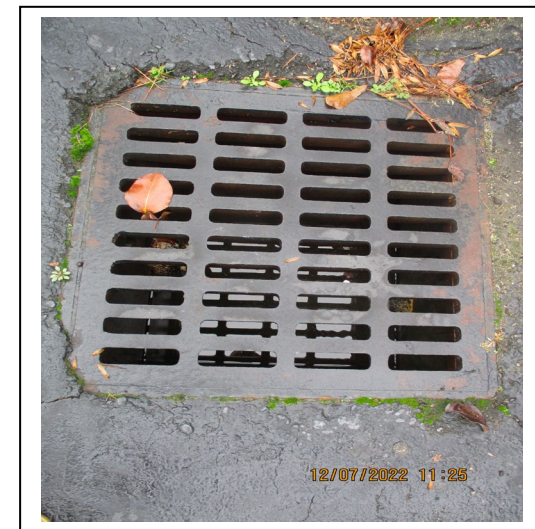
Photo #8 – Stormwater from the CAA pad (Photo #7) discharges into the stormwater drain.
