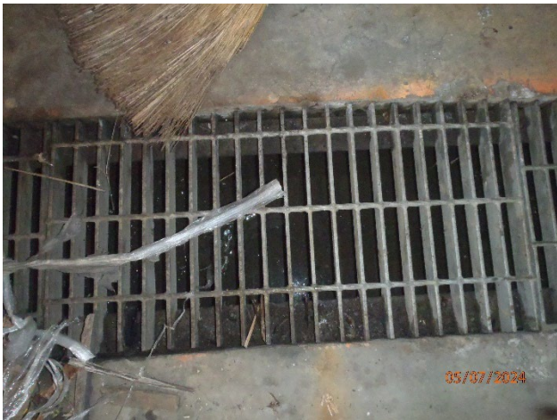
Picture 2 – Main Warehouse floor drain sump need pump out
