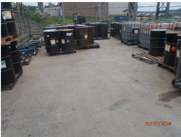
Picture 42 – HWCAA secondary containment cracks and damage
