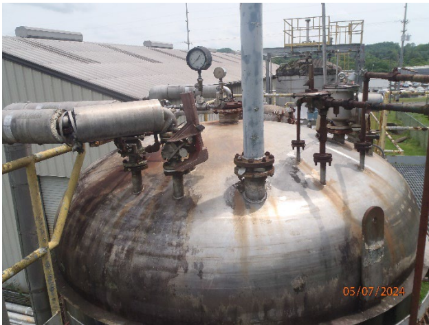
Picture 58 – Hazardous Waste T-61 missing BB tags
