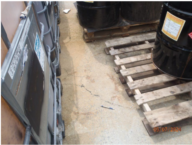
Picture 40 – HWCAA secondary containment cracks
