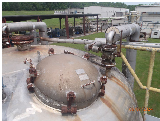
Picture 55 – Hazardous Waste T-61 missing BB tags
