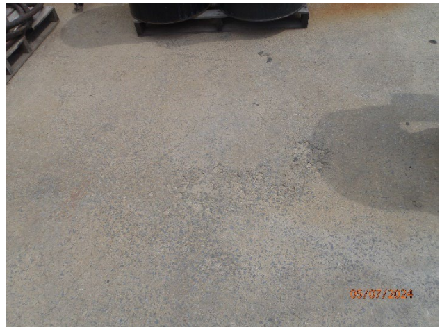
Picture 38 – HWCAA secondary containment damaged
