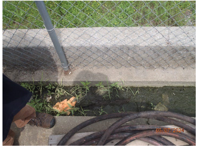
Picture 37 – HWCAA secondary containment sump
