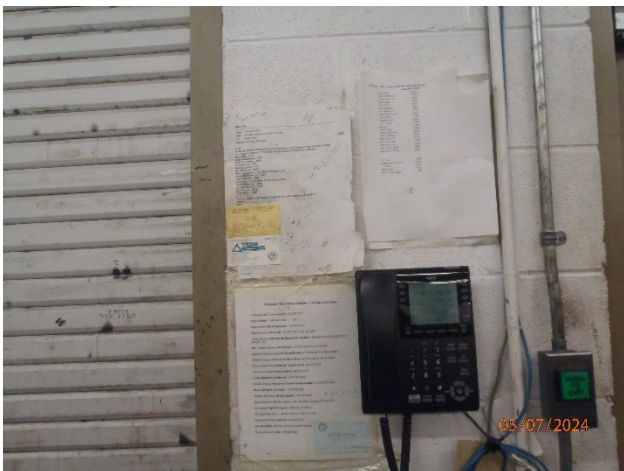
Picture 3 – Maintenance out of date emergency contact list
