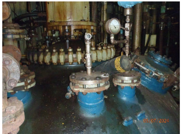
Picture 79 – Building 6 HW Tank 613 roof missing BB tags
