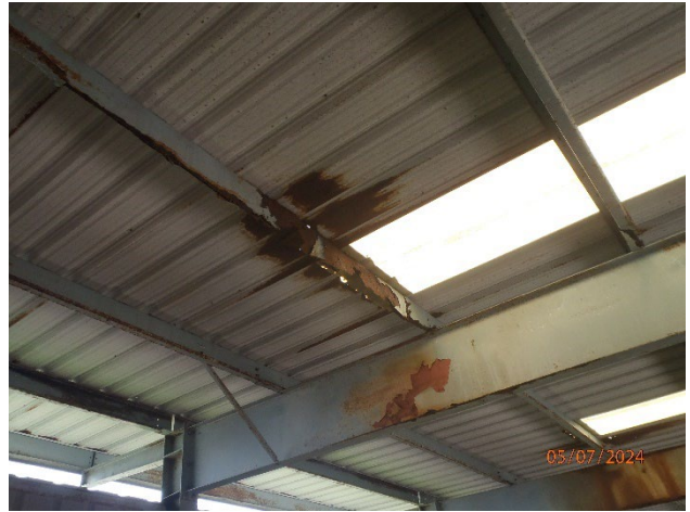
Picture 83 – Building 6 Tank Farm roof corrosion
