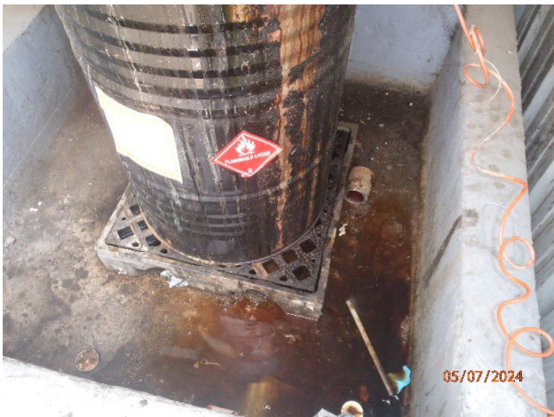
Picture 60 – Lab CAA secondary containment needs clean out
