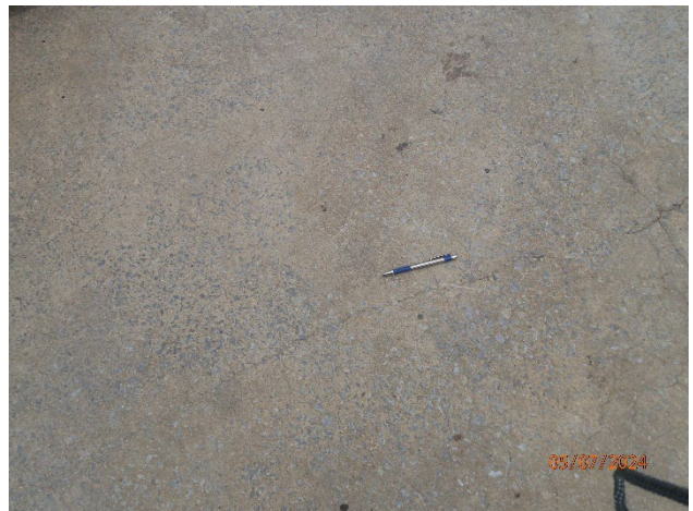
Picture 39 – HWCAA secondary containment cracks
