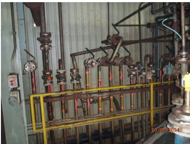
Picture 76 – Building 6 HW Tank 613 missing BB tags
