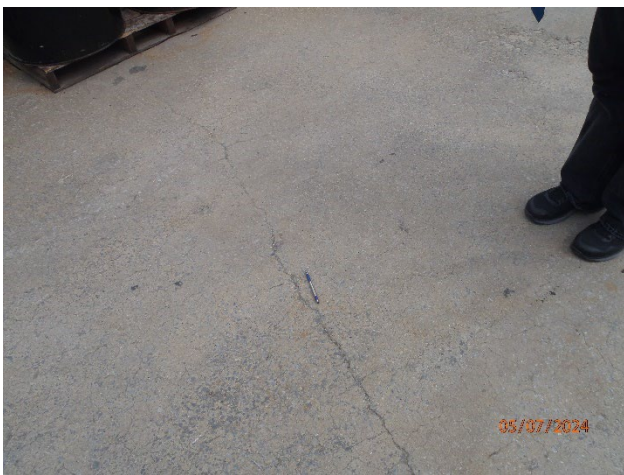
Picture 41 – HWCAA secondary containment cracks
