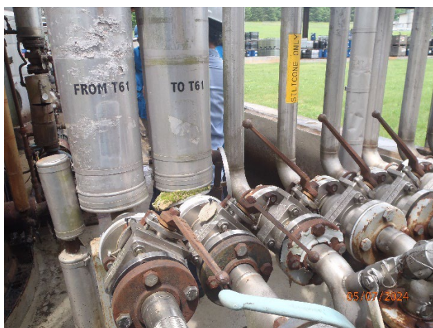
Picture 54 – Hazardous Waste T-61 missing BB tags
