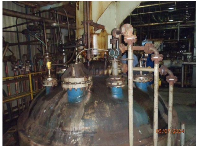
Picture 78 – Building 6 HW Tank 613 roof missing BB tags
