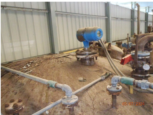
Picture 82 – Building 6 Tank Farm missing BB tags
