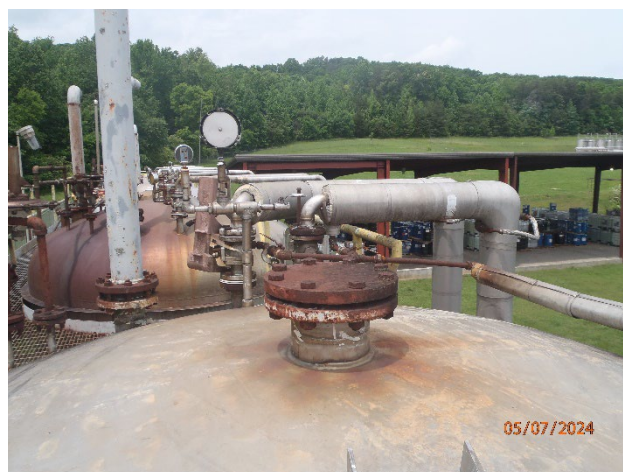
Picture 57 – Hazardous Waste T-61 missing BB tags
