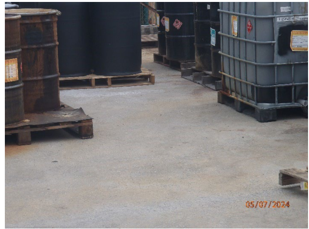
Picture 43 – HWCAA secondary containment cracks and damage
