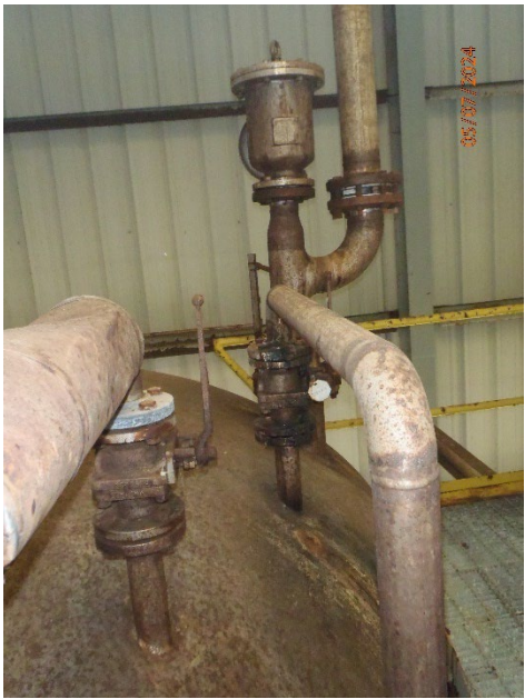
Picture 80 – Building 6 Tank Farm missing BB tags
