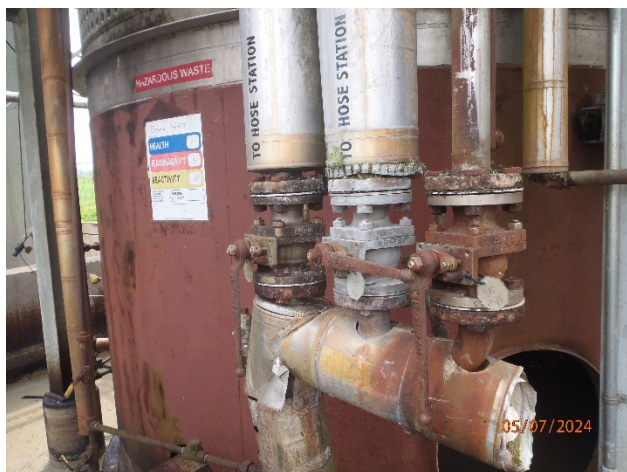
Picture 52 – Hazardous Waste T-61 missing BB tags
