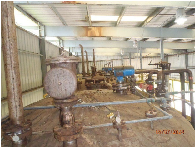
Picture 81 – Building 6 Tank Farm missing BB tags
