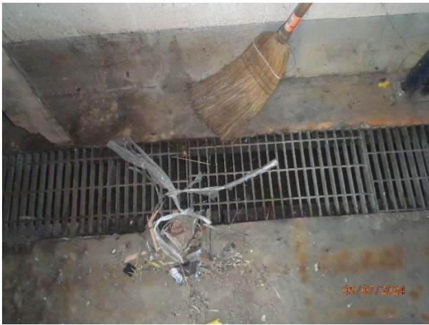
Picture 1 – Main Warehouse floor drain sump need pump out
