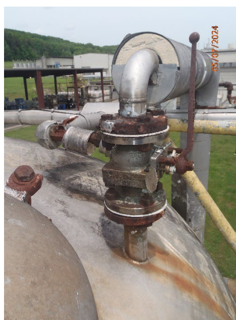
Picture 56 – Hazardous Waste T-61 missing BB tags
