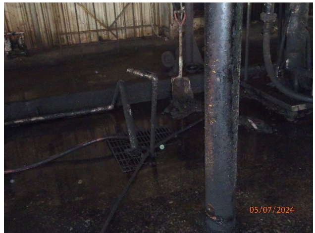
Picture 85 – Building 6 loading area with resin and water on ground
