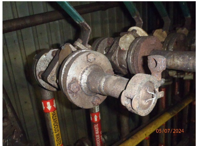
Picture 77 – Building 6 HW Tank 613 missing BB tags
