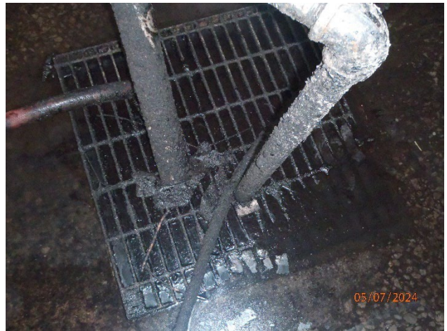
Picture 84 – Building 6 sump drain of resin and water
