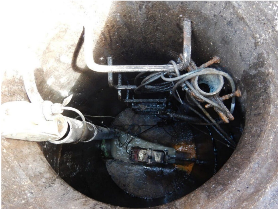
Photograph 3: Sampling manhole at DFA.
