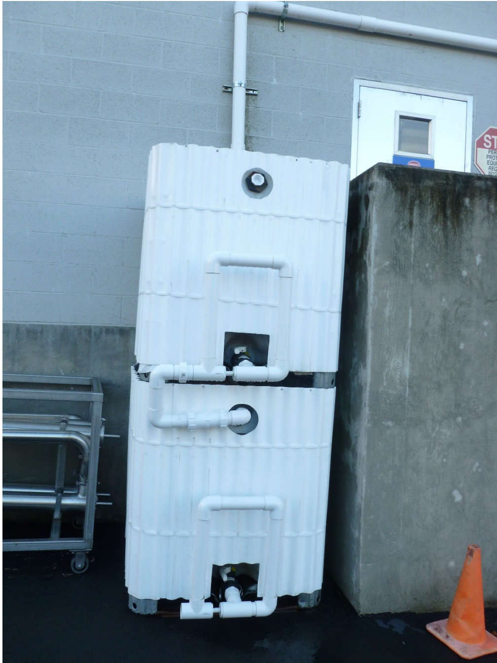
Photo 5 / P1010155 – Filtration System
