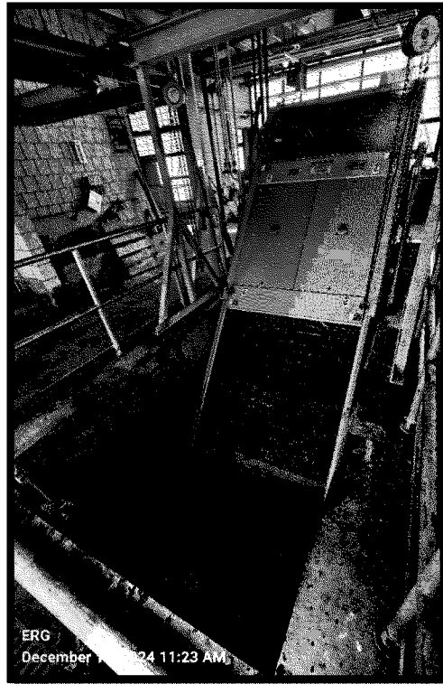
Photograph 3. Offline Step screen, the red arrow added by inspector to indicate a high-water level line.
