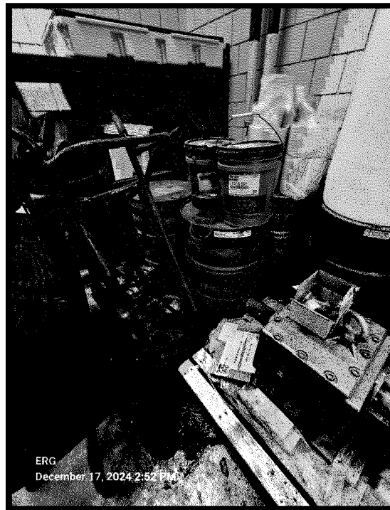
Photograph 29. Buckets and drums of oil and lubricants stored in the stock room without containment. Note the pathway of oil from the floor drain to the nearest 55-gallon drum.
