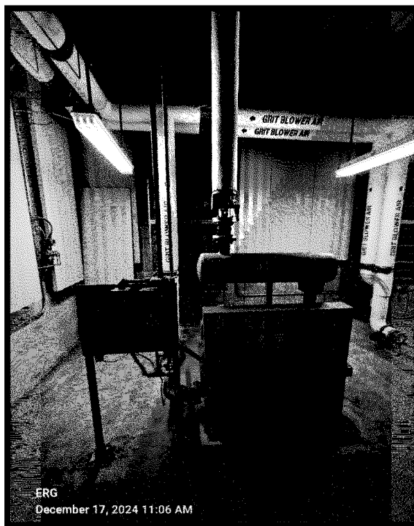
Photograph 4. Aerated grit removal blowers.
