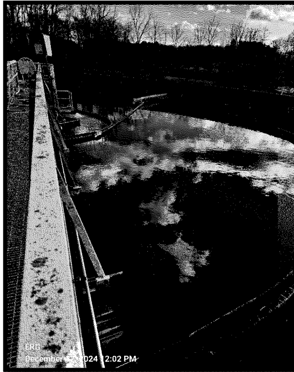
Photograph 15. Secondary clarifier scum skimmer arms. Note the floating solids on the water surface.
