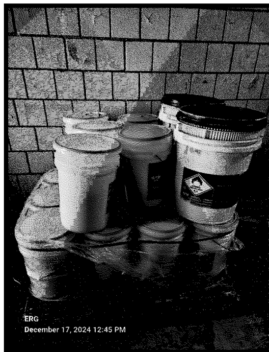
Photograph 28. Buckets of ProChlo stored on a pallet containment located between the gravity thickening area and the sludge blending area.
