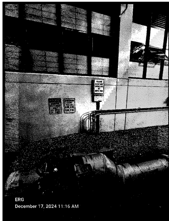
Photograph 2. Septage receiving station.
