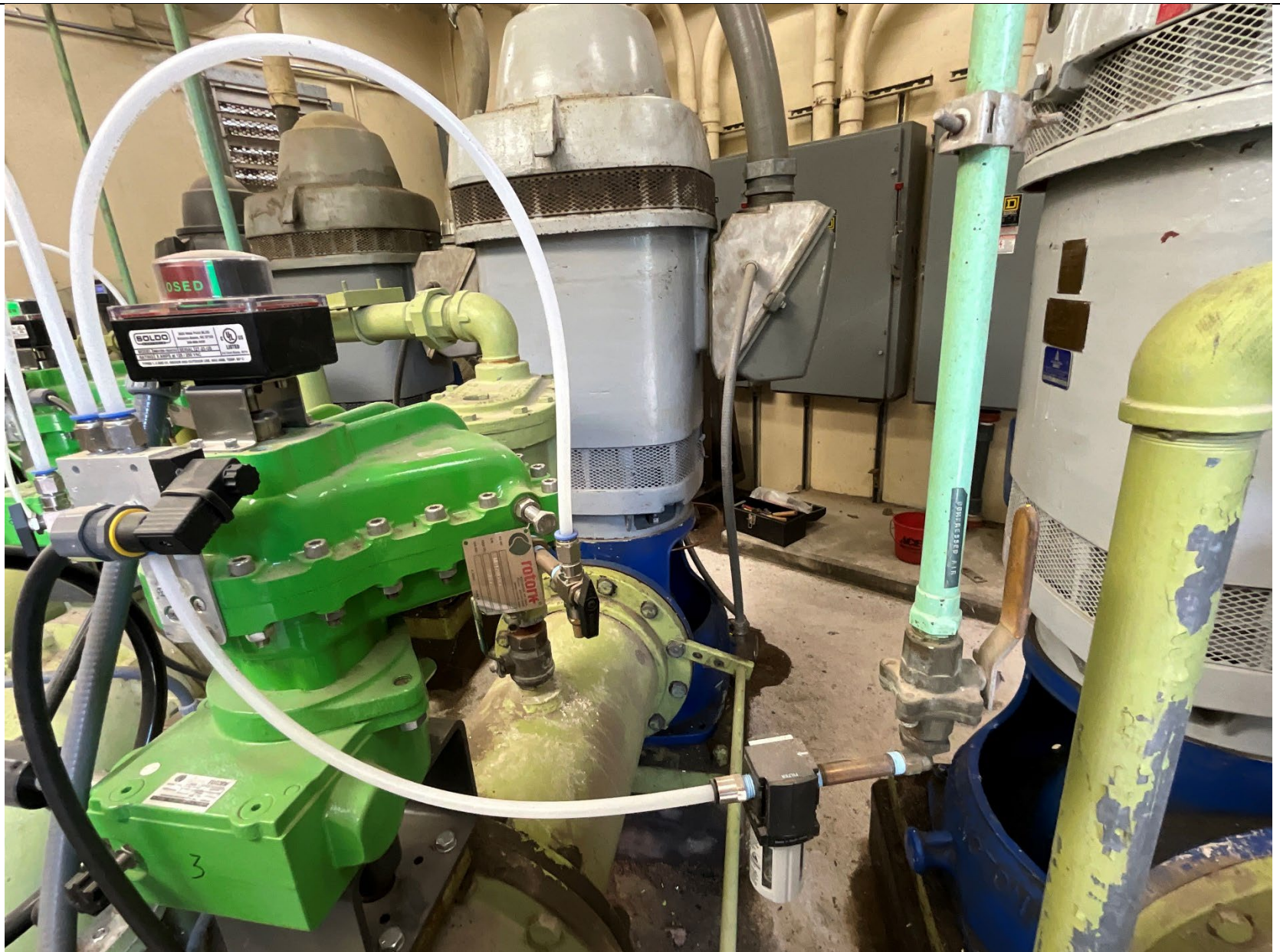
Same as photo 20, zoomed in showing the upgraded valve system that operated on compressed air.
