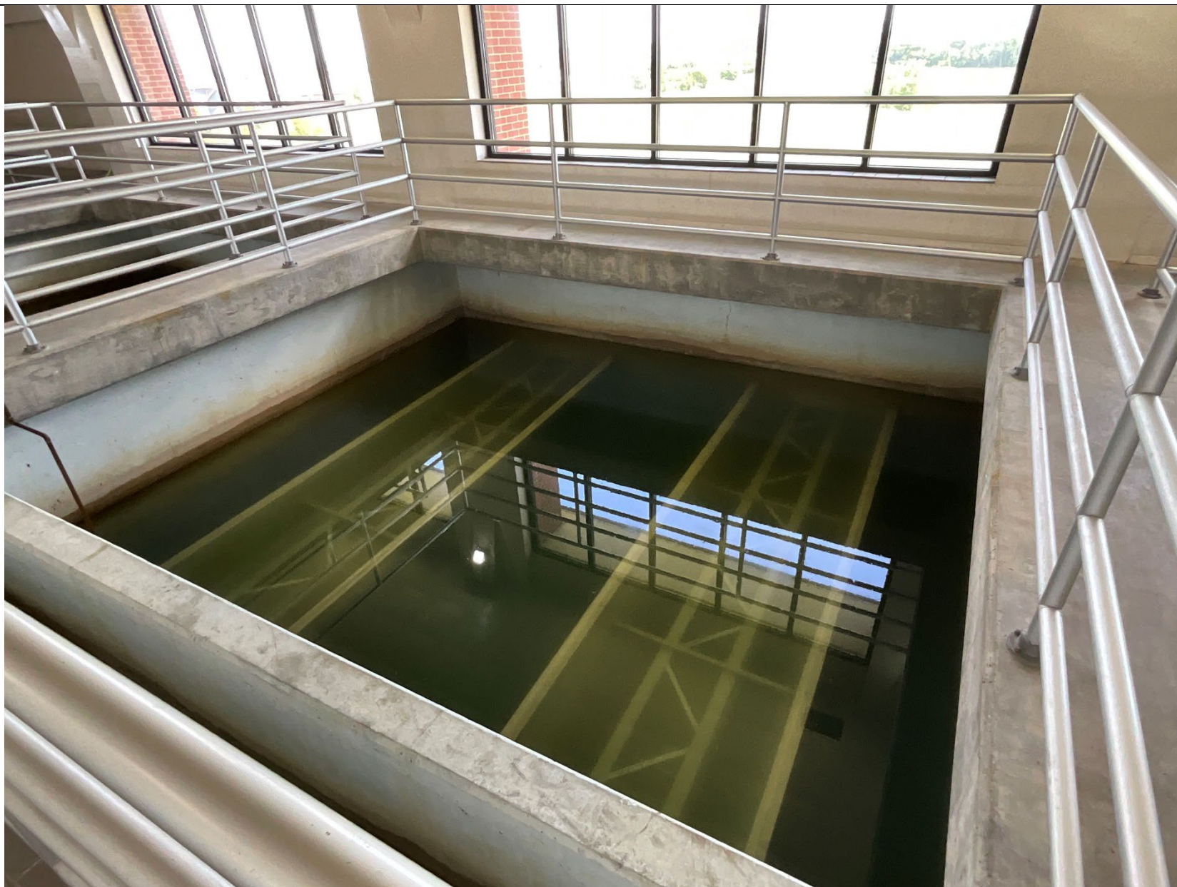
Filtration building, showing 1 of 10 filter basins.
