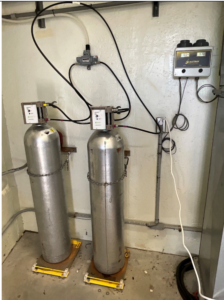
Chlorine gas canisters stored inside the Warren Way elevated water storage tower chemical room.
