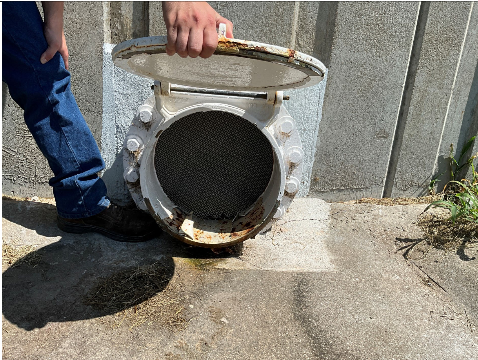
The 12th Avenue elevated water storage tower overflow fitted with a metal flap gate and mess screen. The bottom of mesh screen was blown out.
