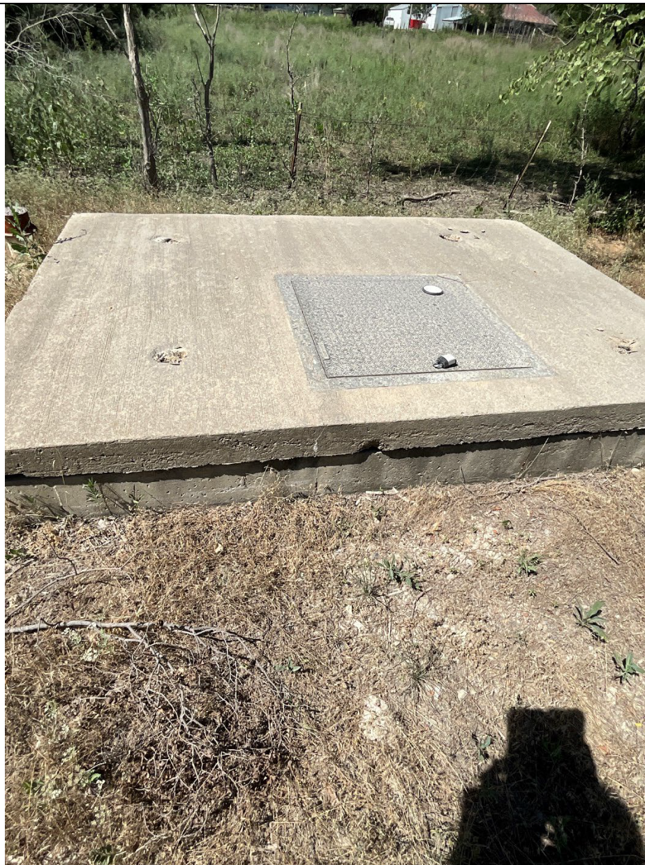
Exterior view of the master meter pit to the consecutive connection to Coffey County RWD #2.
