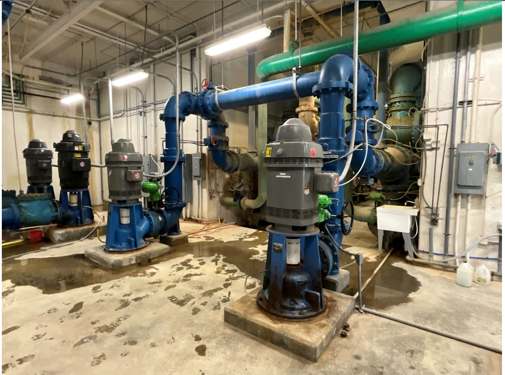
Same photo as photo 13 looking left. Two grey pumps are filter backwash pump. Far left are the 3rd and 4th pumps used to pump finished water to the ground storage tanks.
