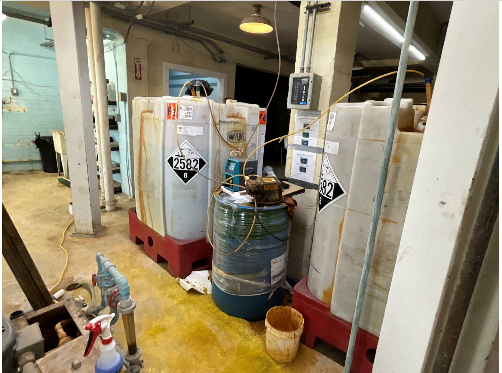
Photo of old chemical building with chemical storage totes, showing spills and spill absorbant materials on the ground.
