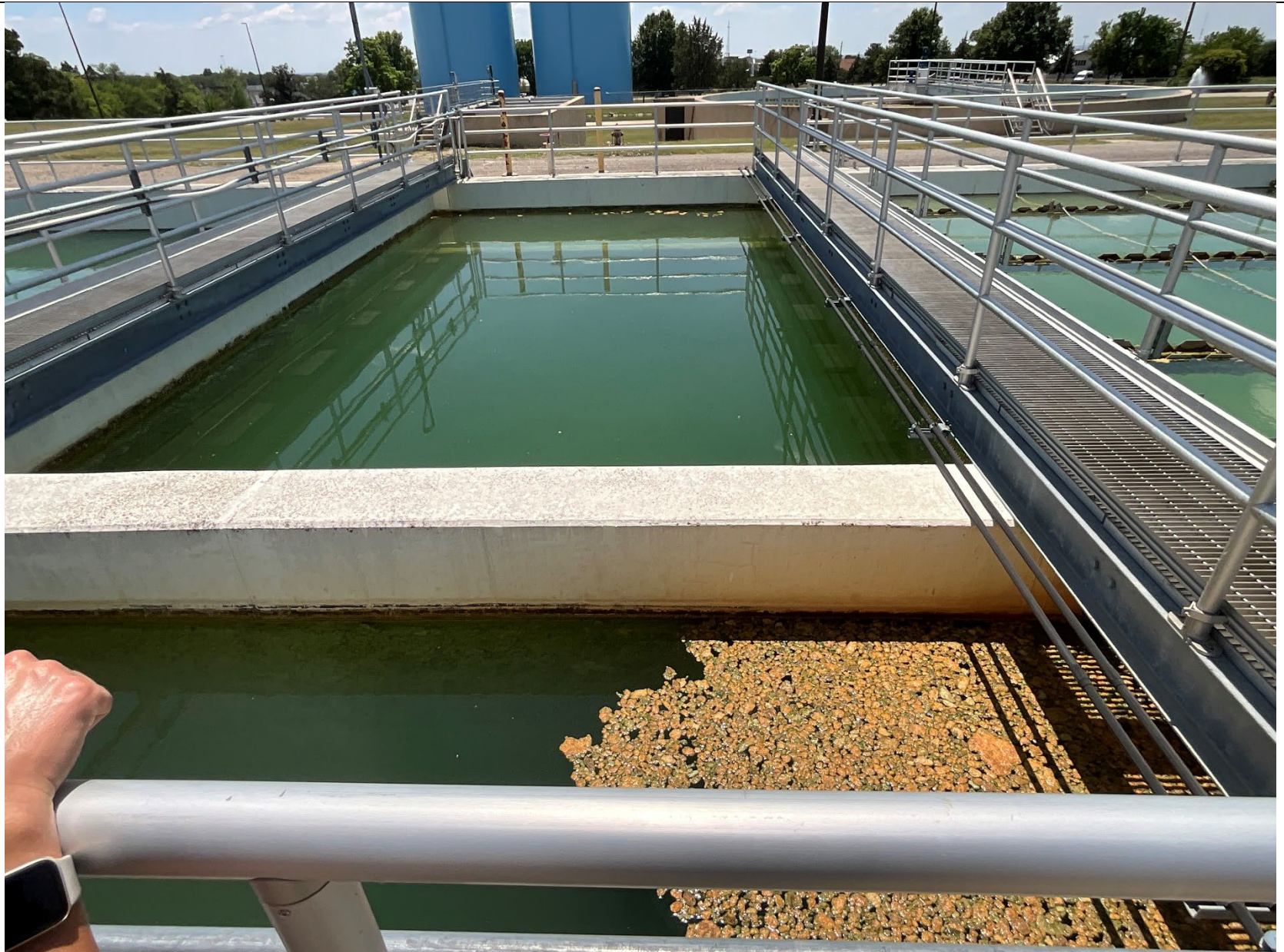
Photo of 1st recarbonization basin #2, showing algae growth floating on the surface of the water.
