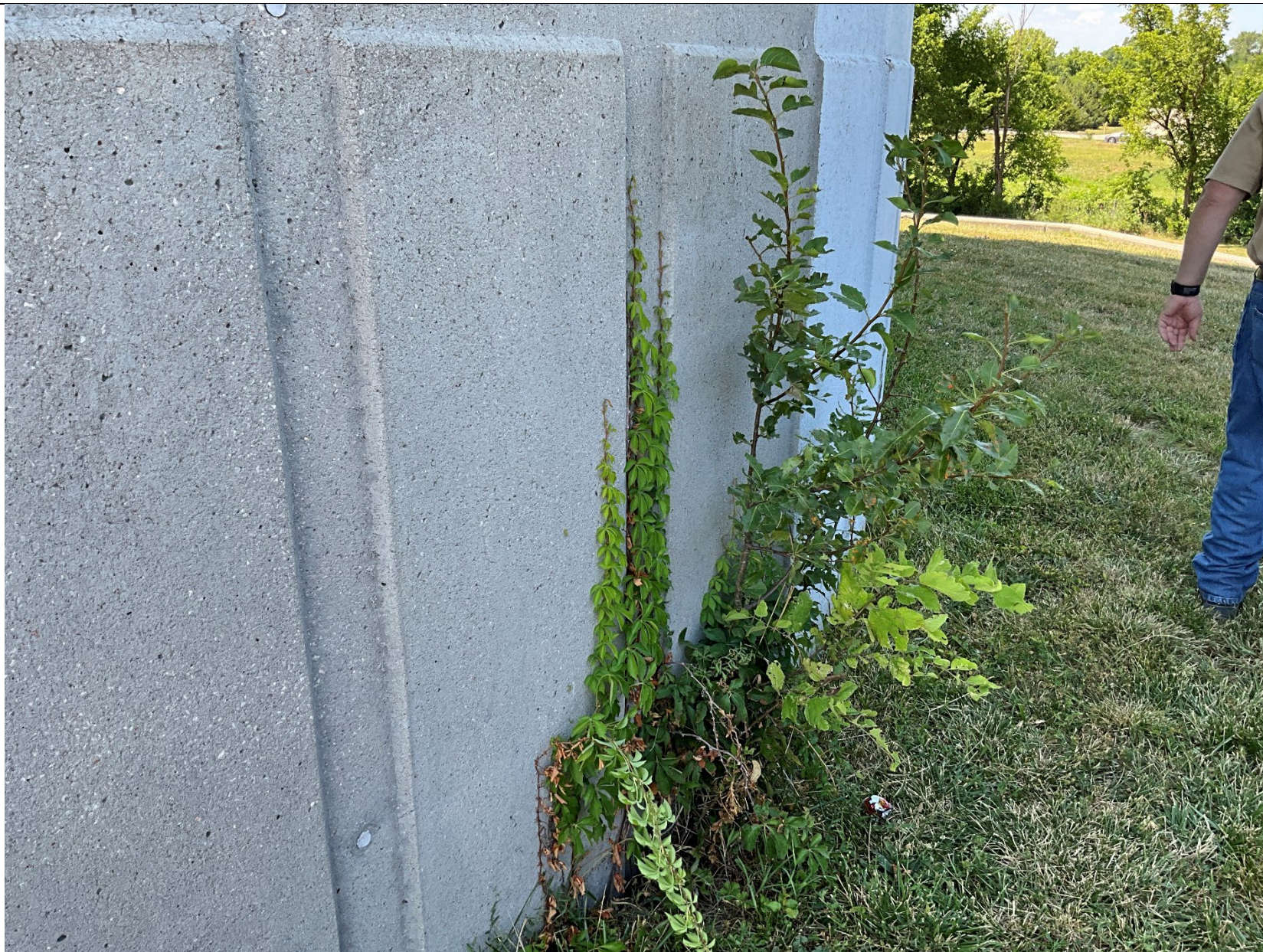
Photo of woody vegetation growing at the base of the 12th Avenue elevated water storage tower.
