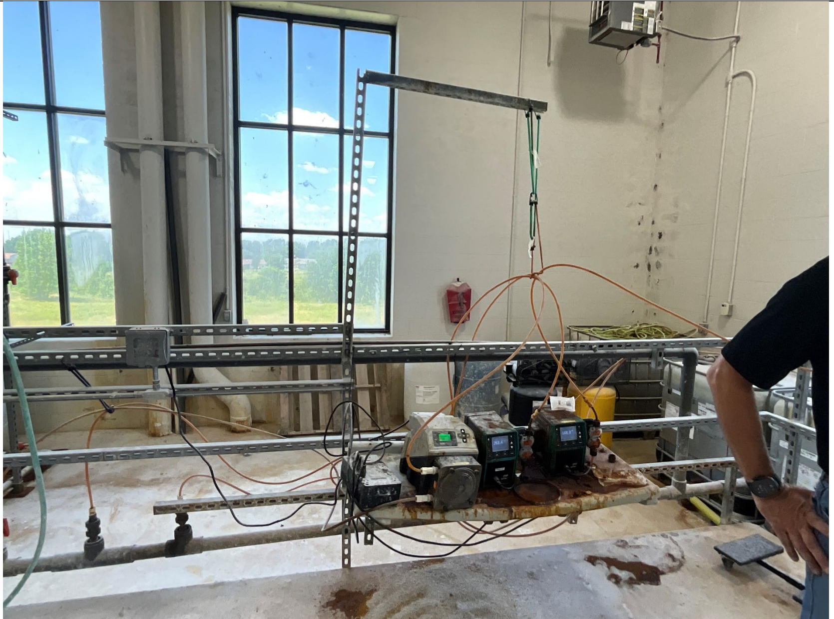
Lime softening building, ferric chloride feed pumps sitting on unstable shelf, significant rusting and deterioration observed.
