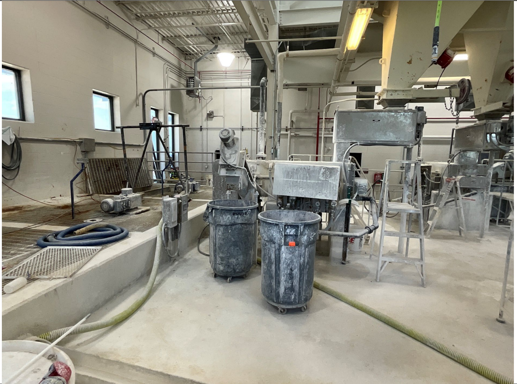
Lime softening building, showing the slaker and basin on the far left where lime is mixed into the water.
