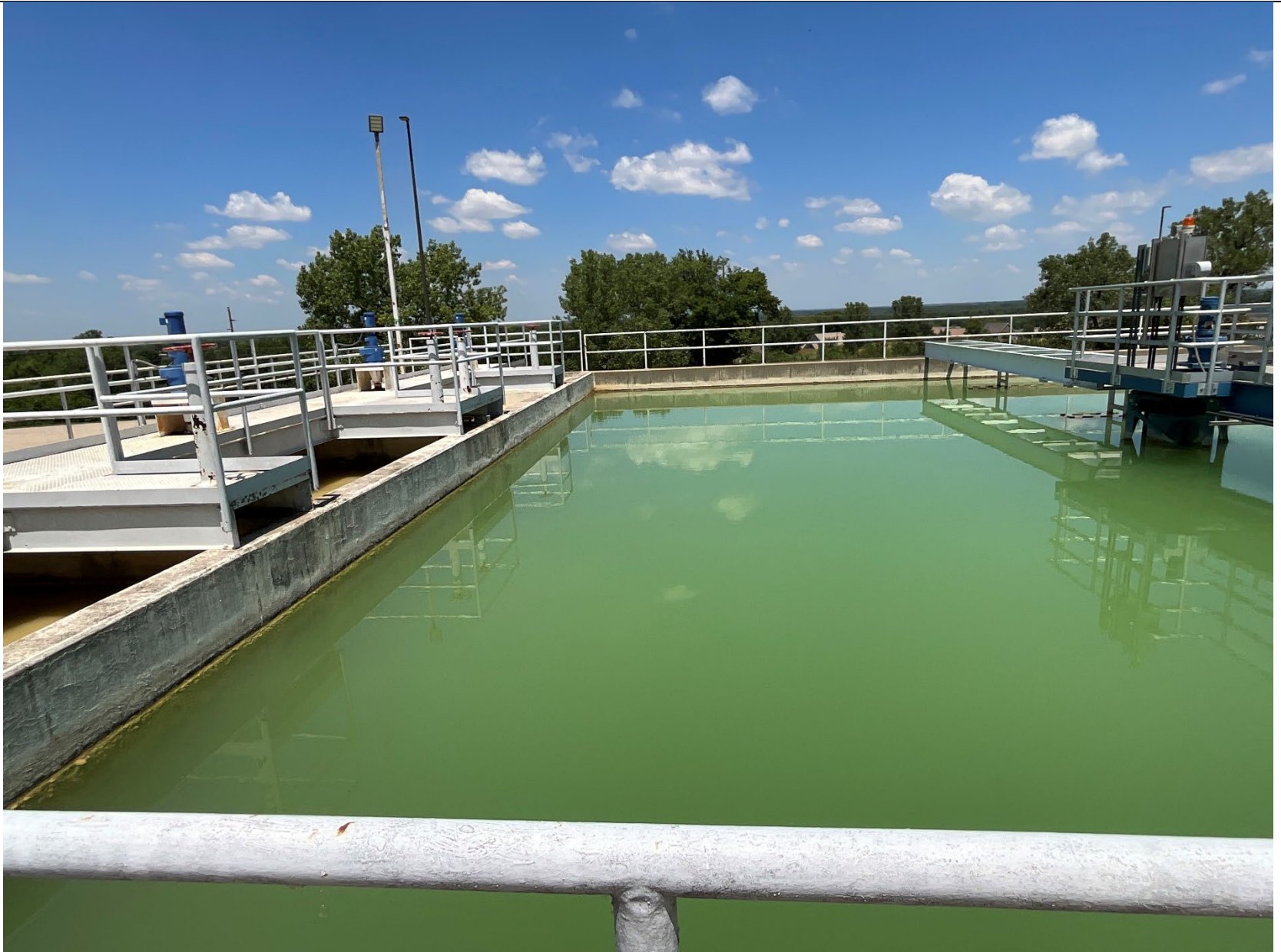
Photo of sedimentation basin #3. Some build up observed around the perimeter of the basin.
