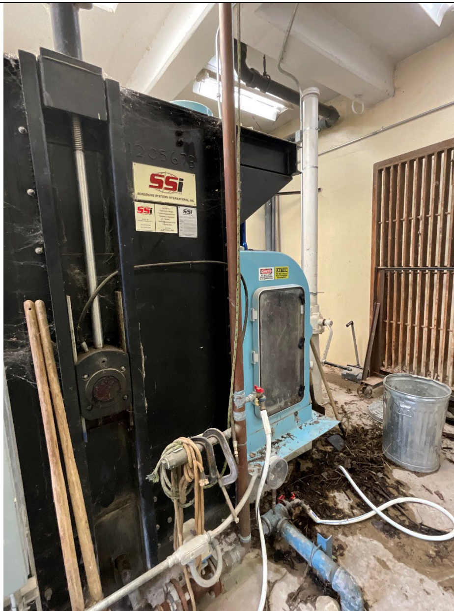
Intake mechanical bar screen with accumulated debris, twigs and leaves on the ground.
