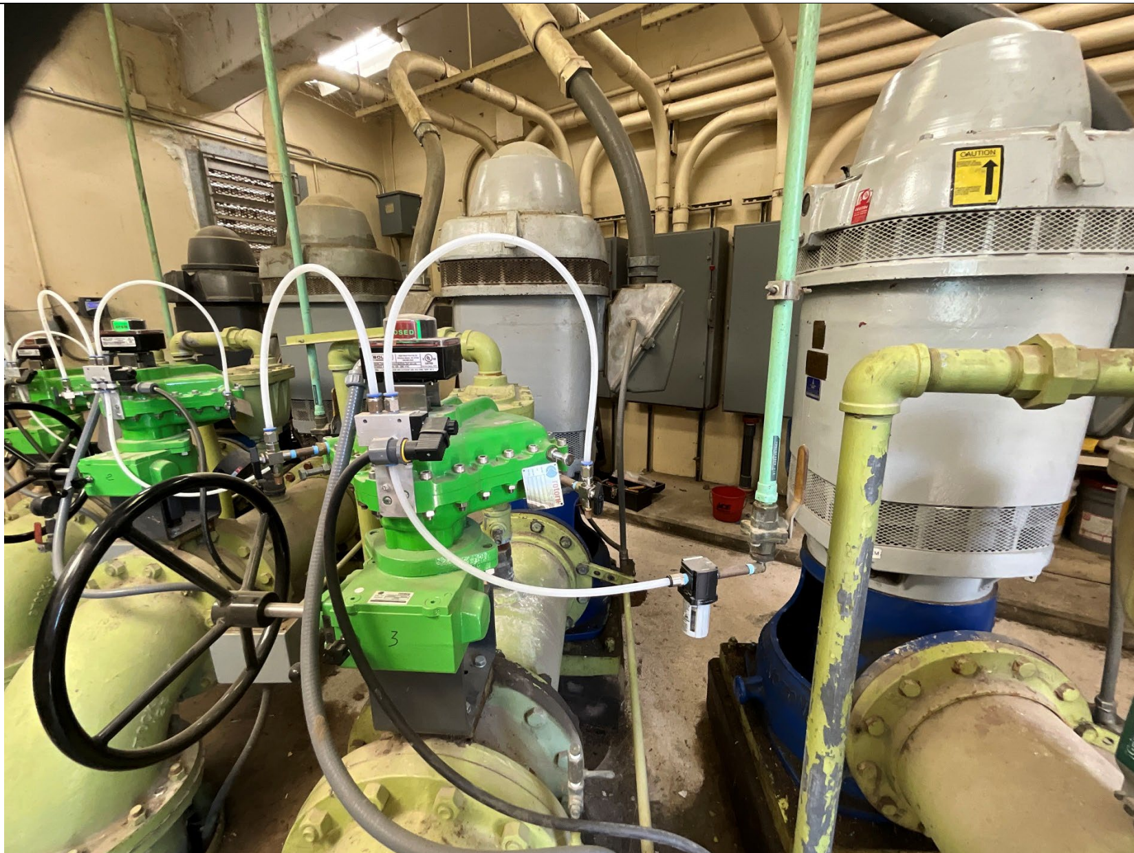
Four turbine pumps housed in the intake building which pump raw water from the Neosho River.
