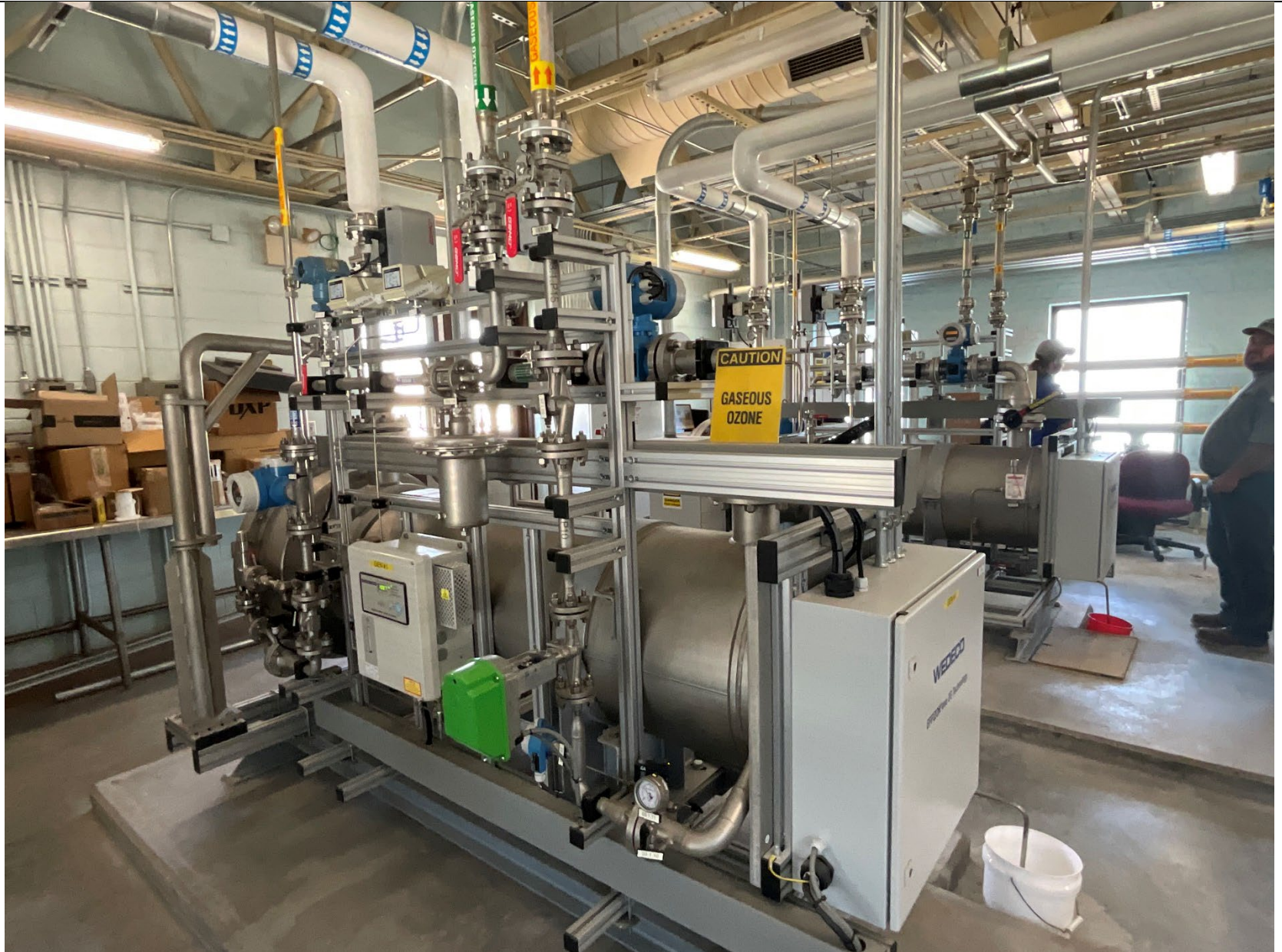
Ozone contact building, showing ozone production equipments converting oxygen to ozone.
