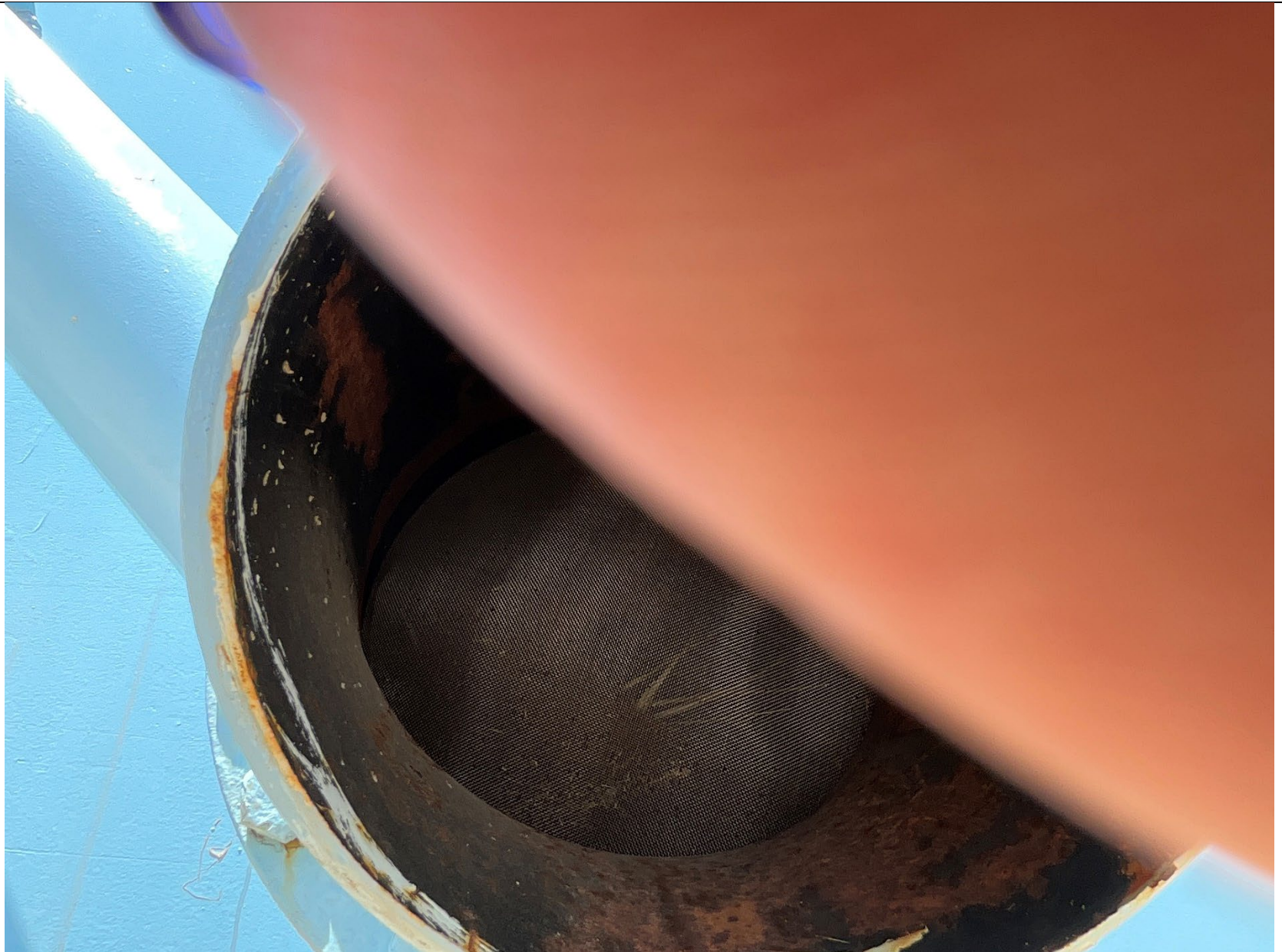
East stand pipe overflow downturned and screened., close up view of screen.
