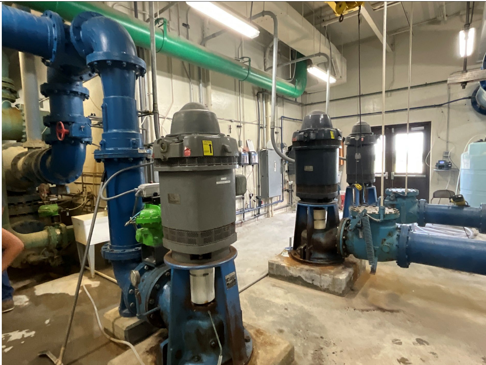
Pipe gallery below the filter basins, pump of the left is one of two filter backwash pumps that filter to waste. Two pumps on the right pump finished water to the ground storage tanks.
