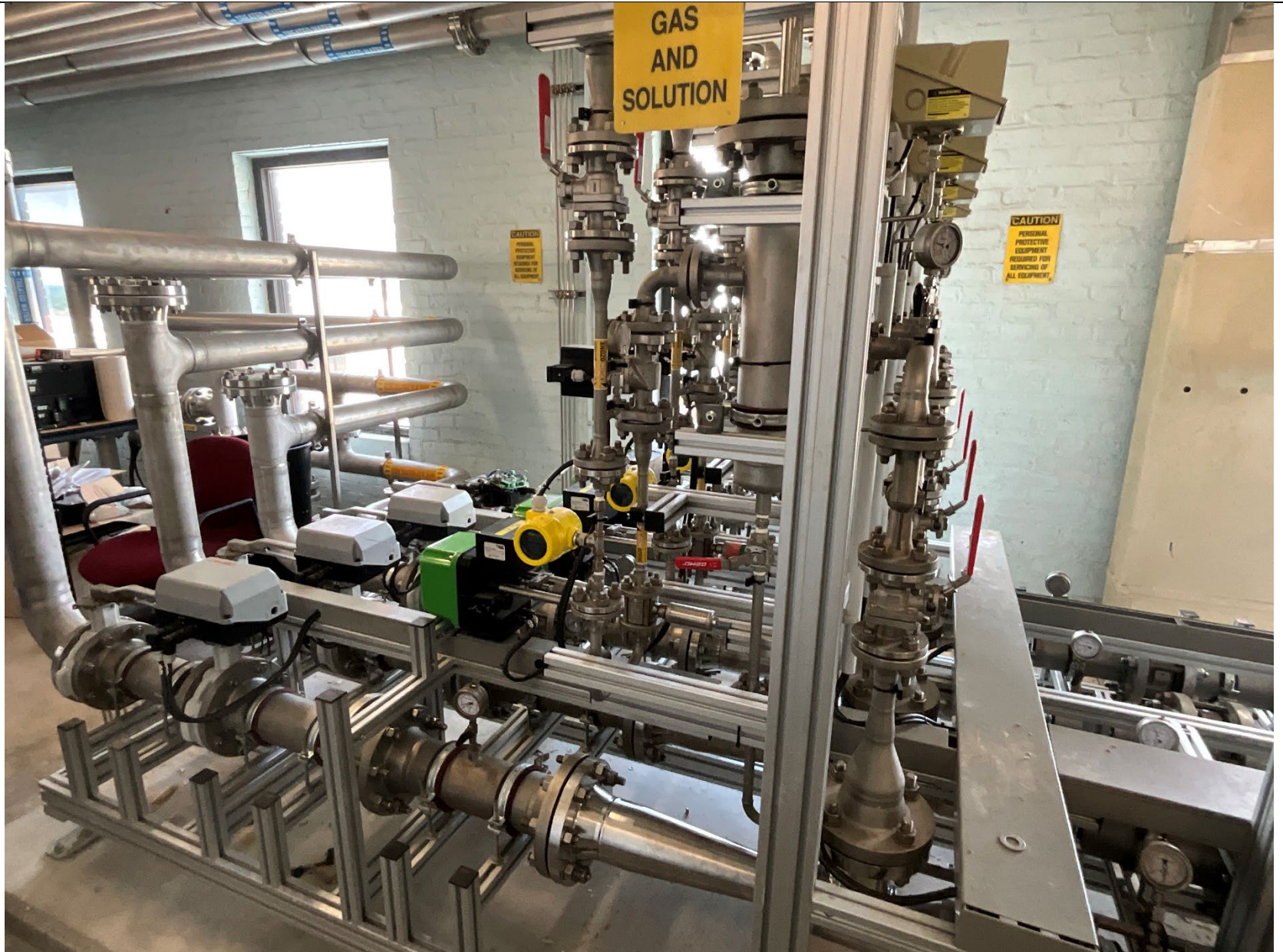
Ozone contact building, showing the ozone injection points. The 4th injection point was down for repair.
