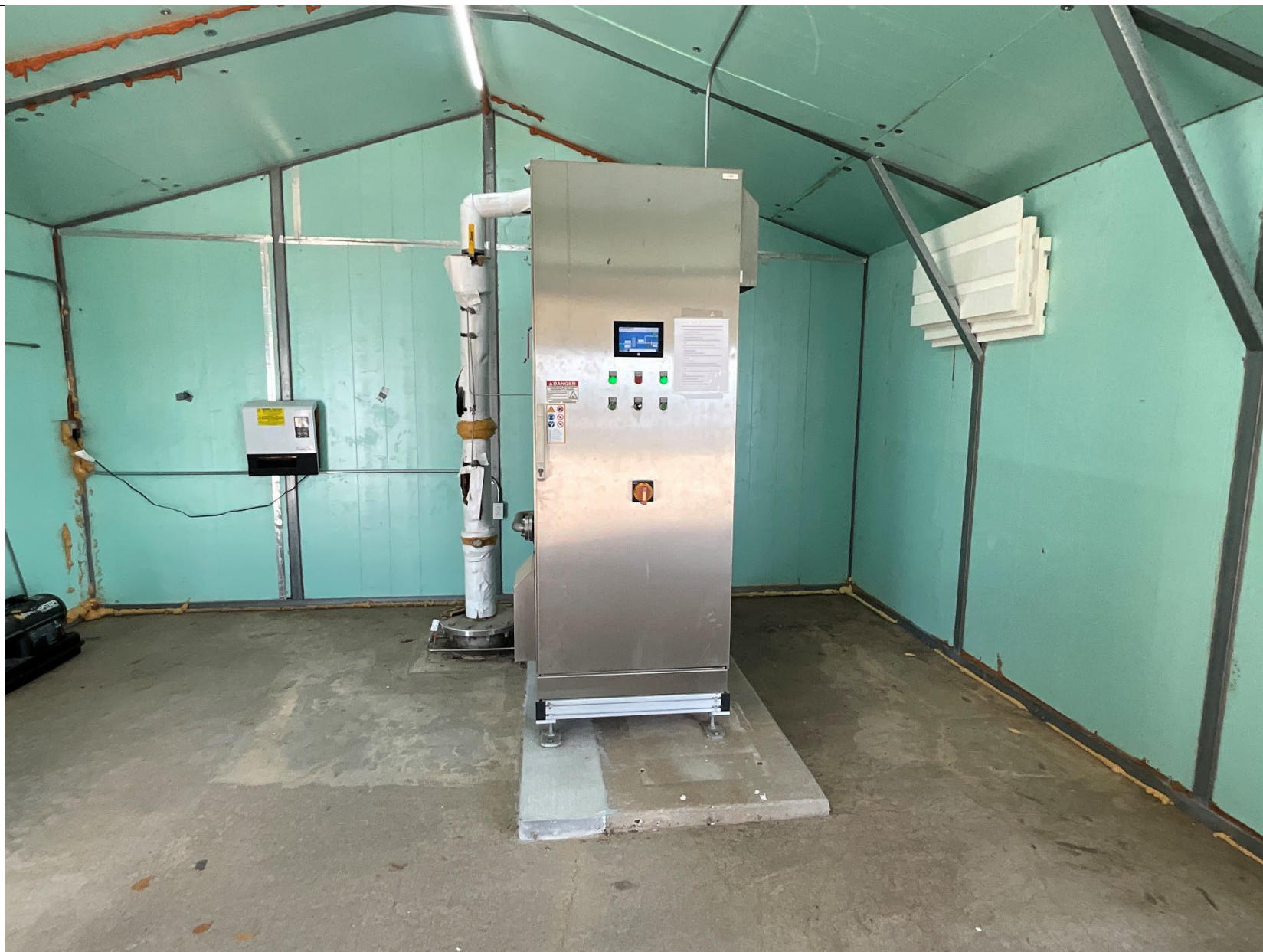
Ozone destruction unit housed in separate building.
