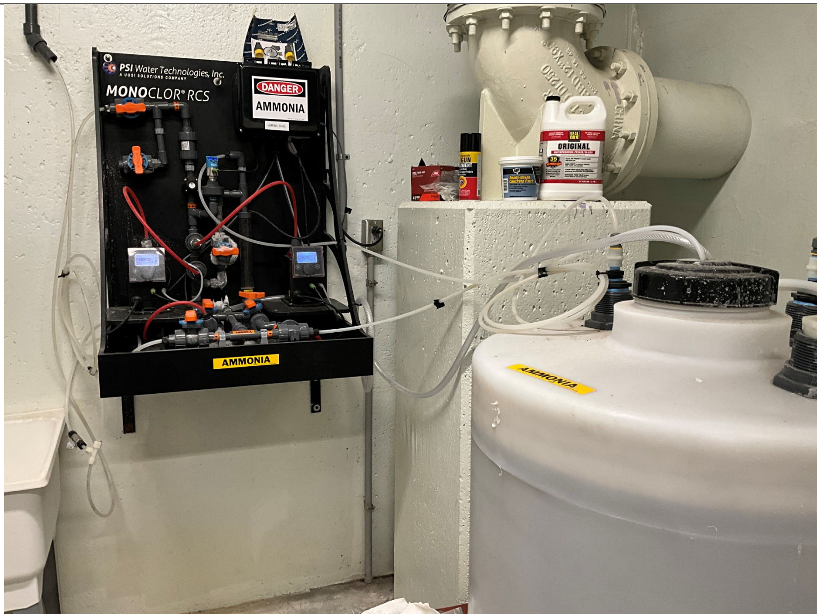
Liquid ammonia storage and feed pump located inside the Warren Way elevated water storage tower chemical room.
