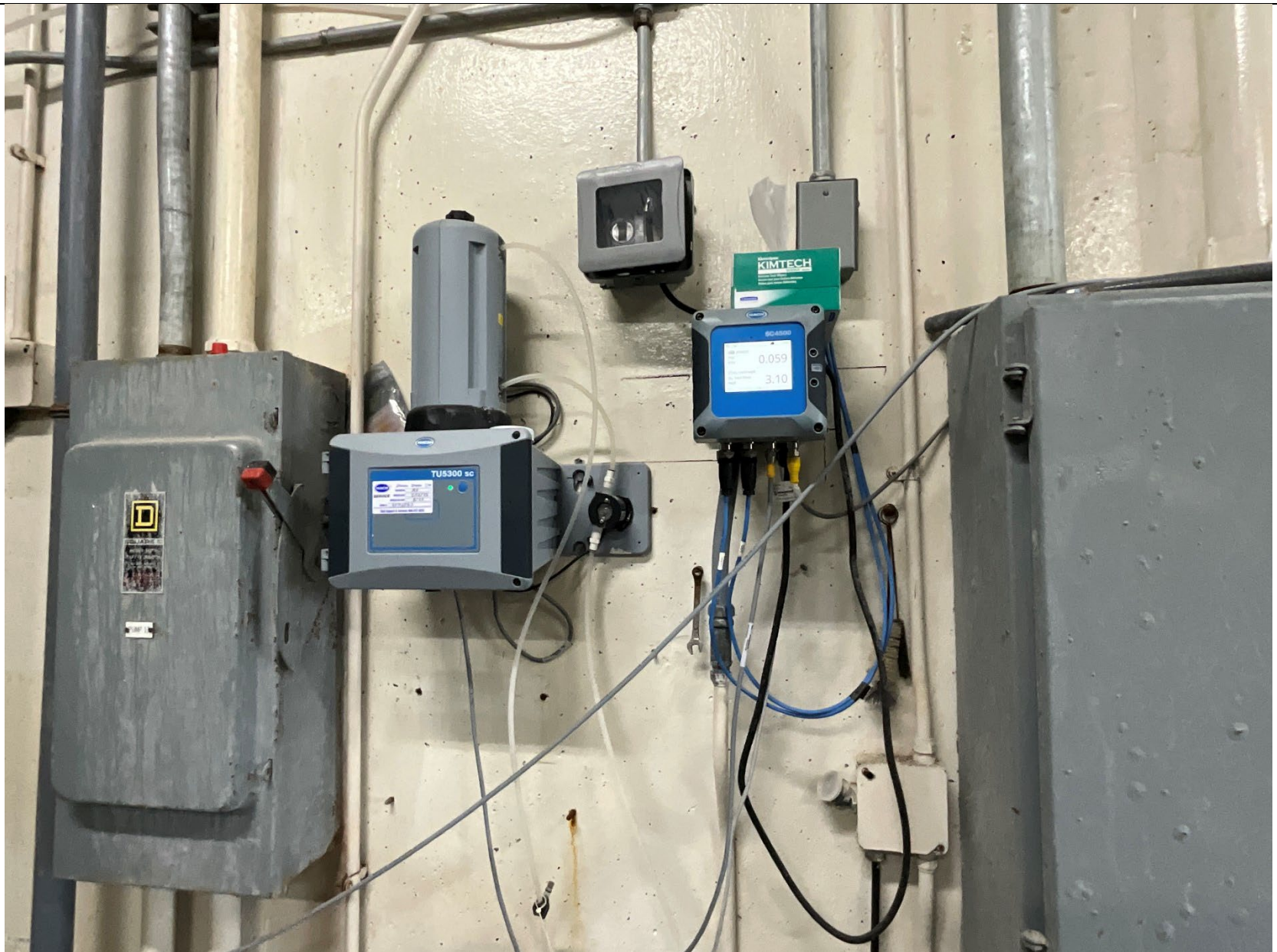
Photo of the CFE turbidimeter located in the pipe gallery below the filter basins, reading 0.059 NTU.
