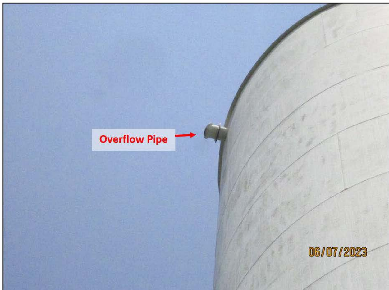
Photograph 14. Overflow Pipe, Liberty Hill Water Tank View of the overflow pipe that extended out of the top of the Liberty Hill Water Tank. It was unclear if the pipe was covered by a screen, and there was no splash pad beneath the pipe.
