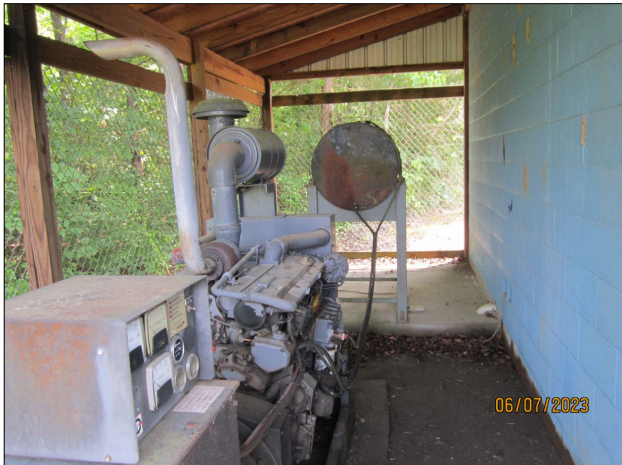
Photograph 31. Backup Generator, Pump Station #1 View of the backup generator that was positioned next to Pump Station #1. The generator was not functional and did not contain a battery.
