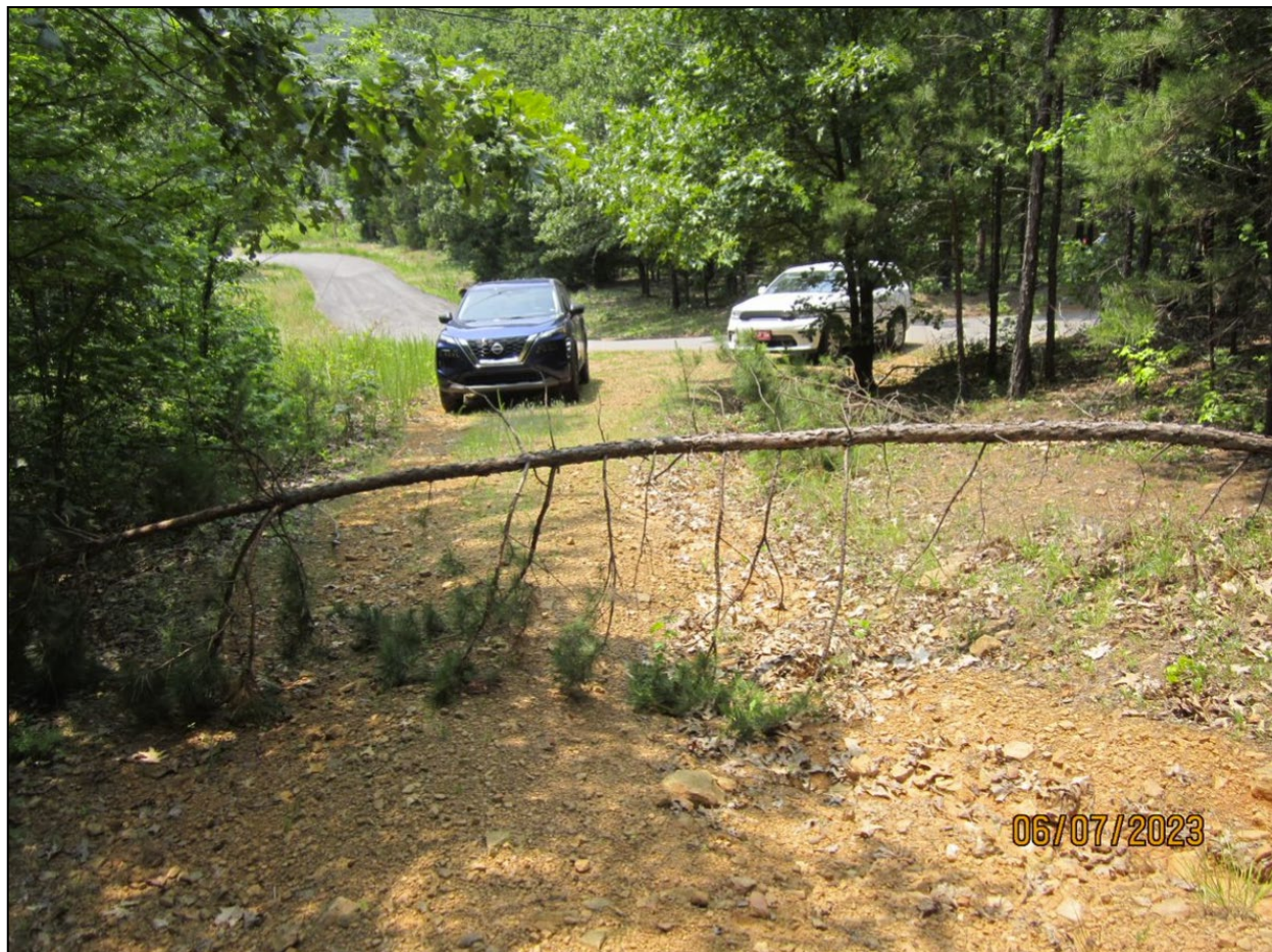
Photograph 18. Access Road, Water Tank #1 View of a fallen tree that was blocking the access road to Water Tank #1. The tree made it so that vehicles could not access the tank. Also visible in this image is heavy erosion in the road due to rainfall.
