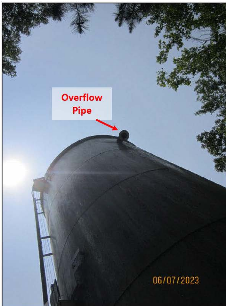
Photograph 21. Water Tank #1 View of the overflow pipe extending out of the top of Water Tank #1. There was no splash pad beneath the overflow pipe.
