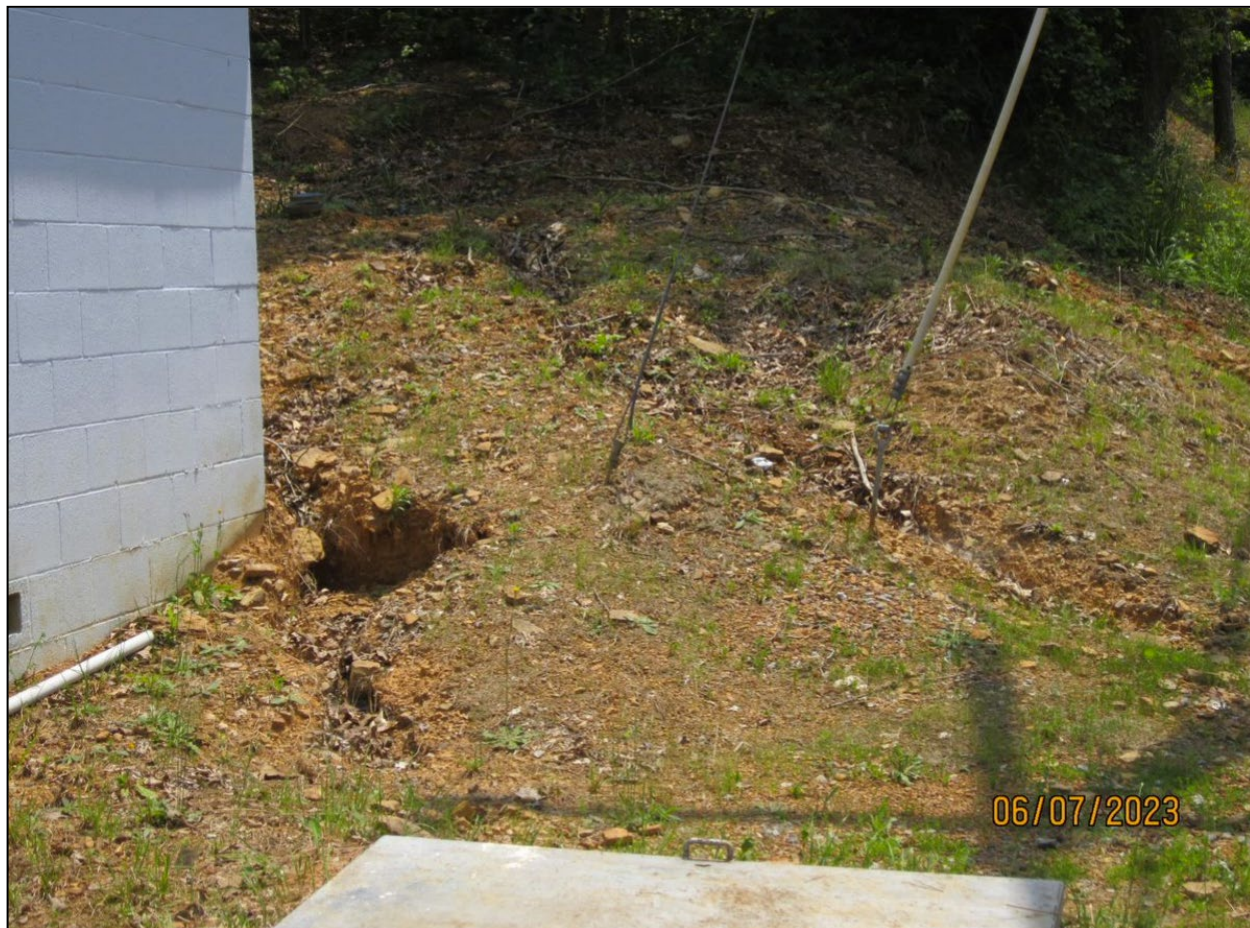
Photograph 37. Pump Station #2 View of the erosion next to Pump Station #2. The hill was sloped toward the pump station, causing rainwater to erode the ground on either side.
