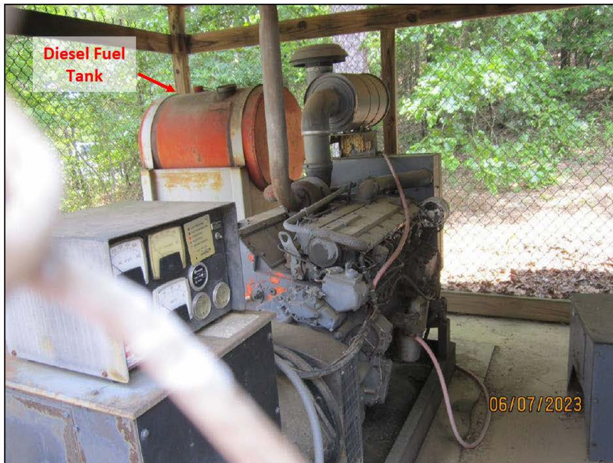
Photograph 32. Backup Generator, Pump Station #2 View of the backup generator that was positioned next to Pump Station #2. The generator was not functional, and there was sludge at the bottom of the diesel fuel tank next to the generator.
