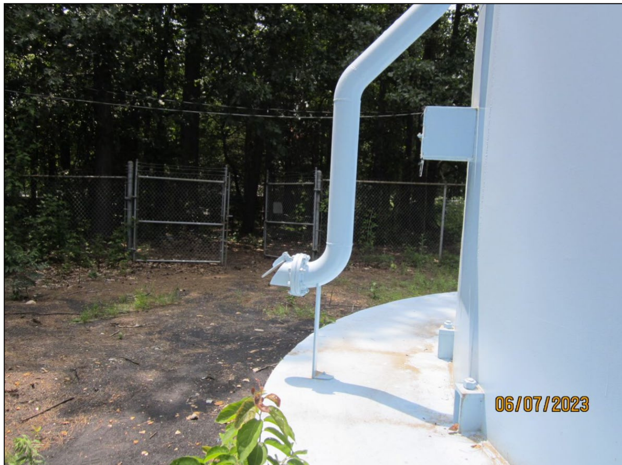
Photograph 26. Overflow Pipe, Ridgecrest Water Tank View of the end of the overflow pipe that extended out of the Ridgecrest Water Tank. The flapper valve was open and there was no concrete splash pad beneath the pipe.
