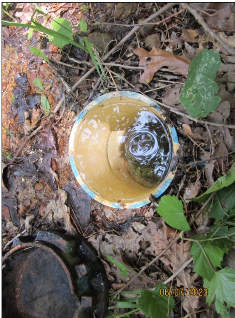
Photograph 34. Valve Port, Pump Station #2 View of a valve box PVC line to valve stem that was leaking potable water. The water was running down the hill toward the pump station, and the System Manager stated that he was aware of the leak. The area had blue spray paint line on the ground in preparation for excavation.
