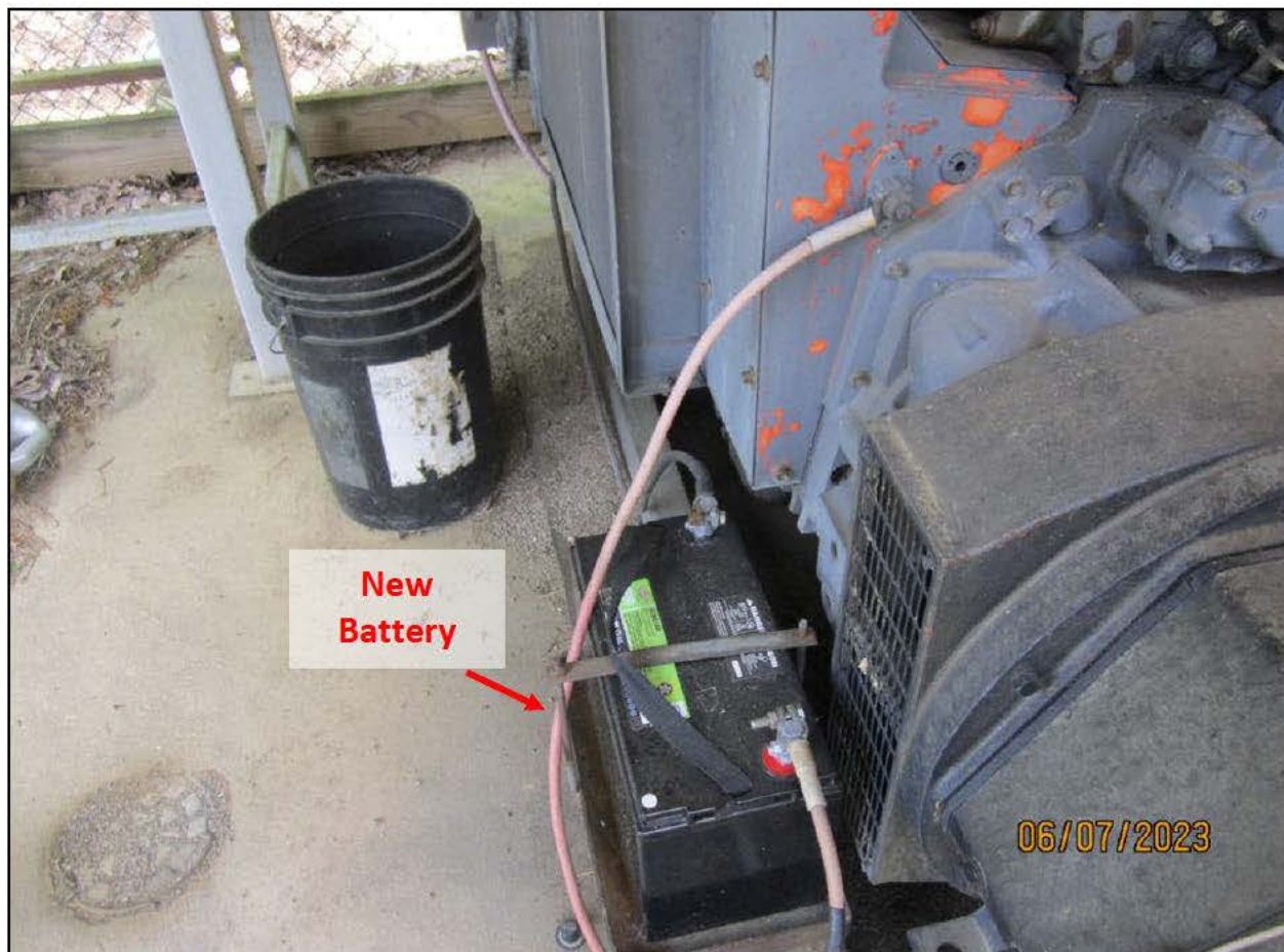
Photograph 33. Backup Generator, Pump #2 View of the battery sitting next to the backup generator next to Pump #2. The generator was not functional, but System representatives stated that the battery was new.
