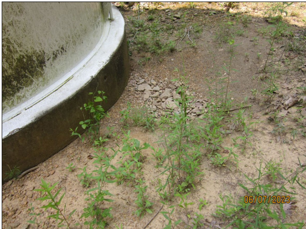
Photograph 22. Water Tank #1 View of the erosion underneath the overflow pipe at Water Tank #1.
