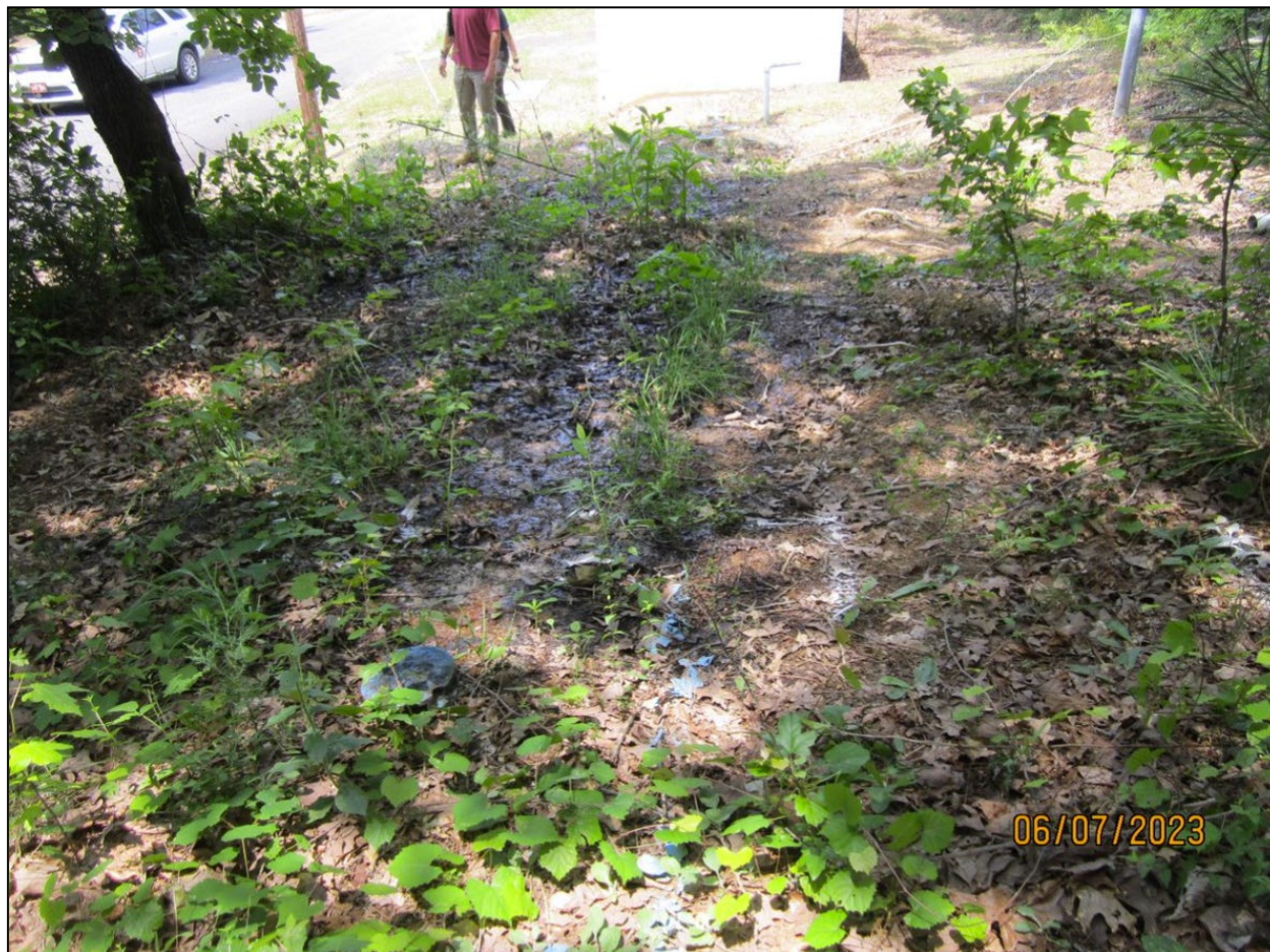
Photograph 35. Valve, Pump Station #2 View of hill sloping toward Pump Station #2 where potable water leaking from the valve was draining. Blue paint was observed on the ground in this area.
