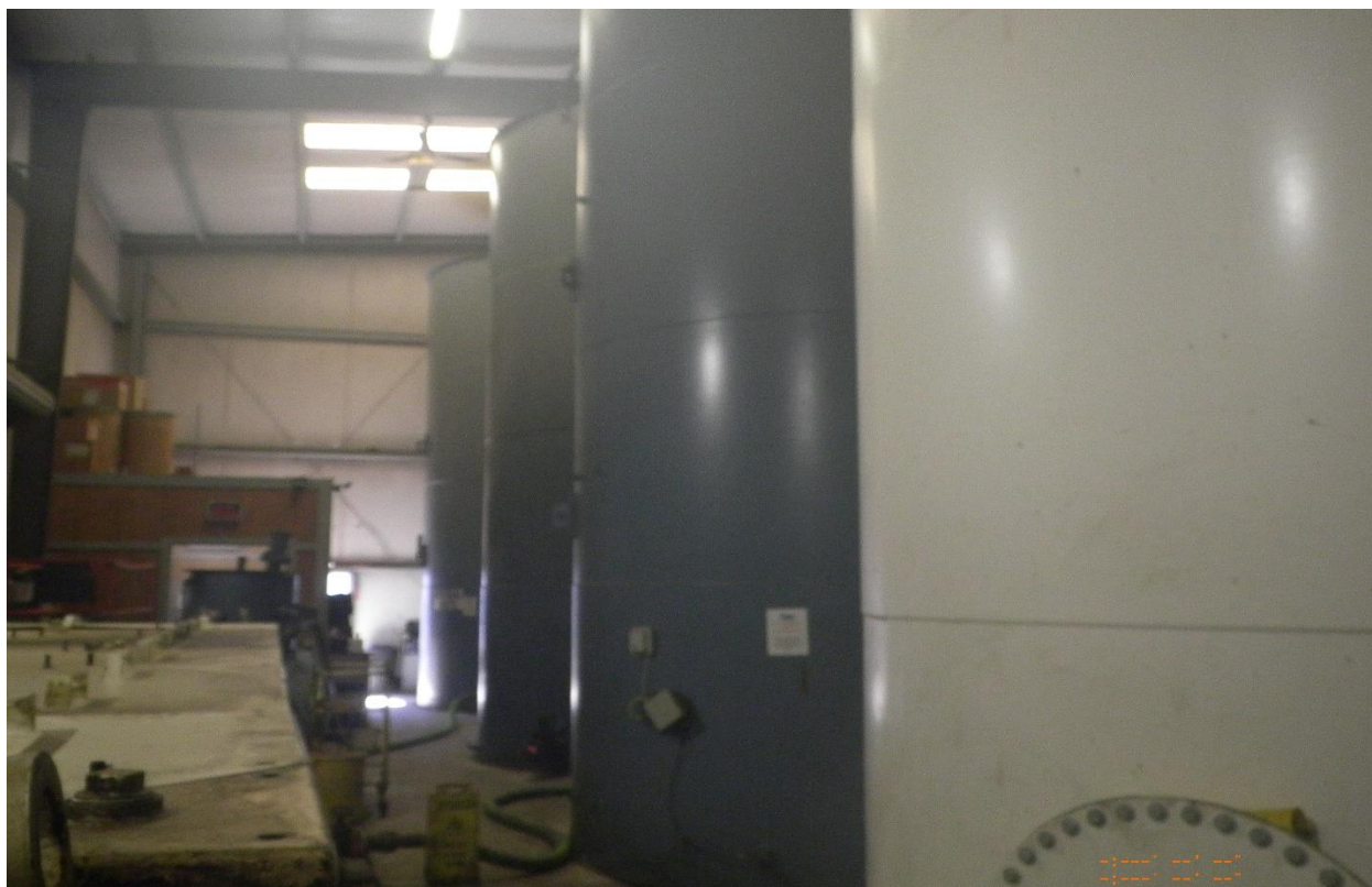
8. 20,000 gallon wastewater tanks inside building – PRC – 09/14/22
