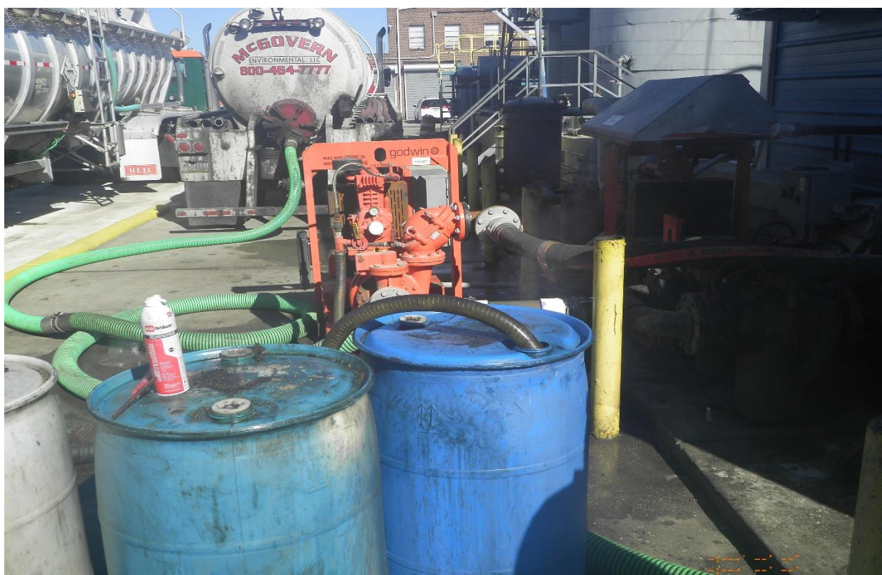
2. Portable Pump Venting to Drum w/Visible Smoke – PRC – 09/14/22
