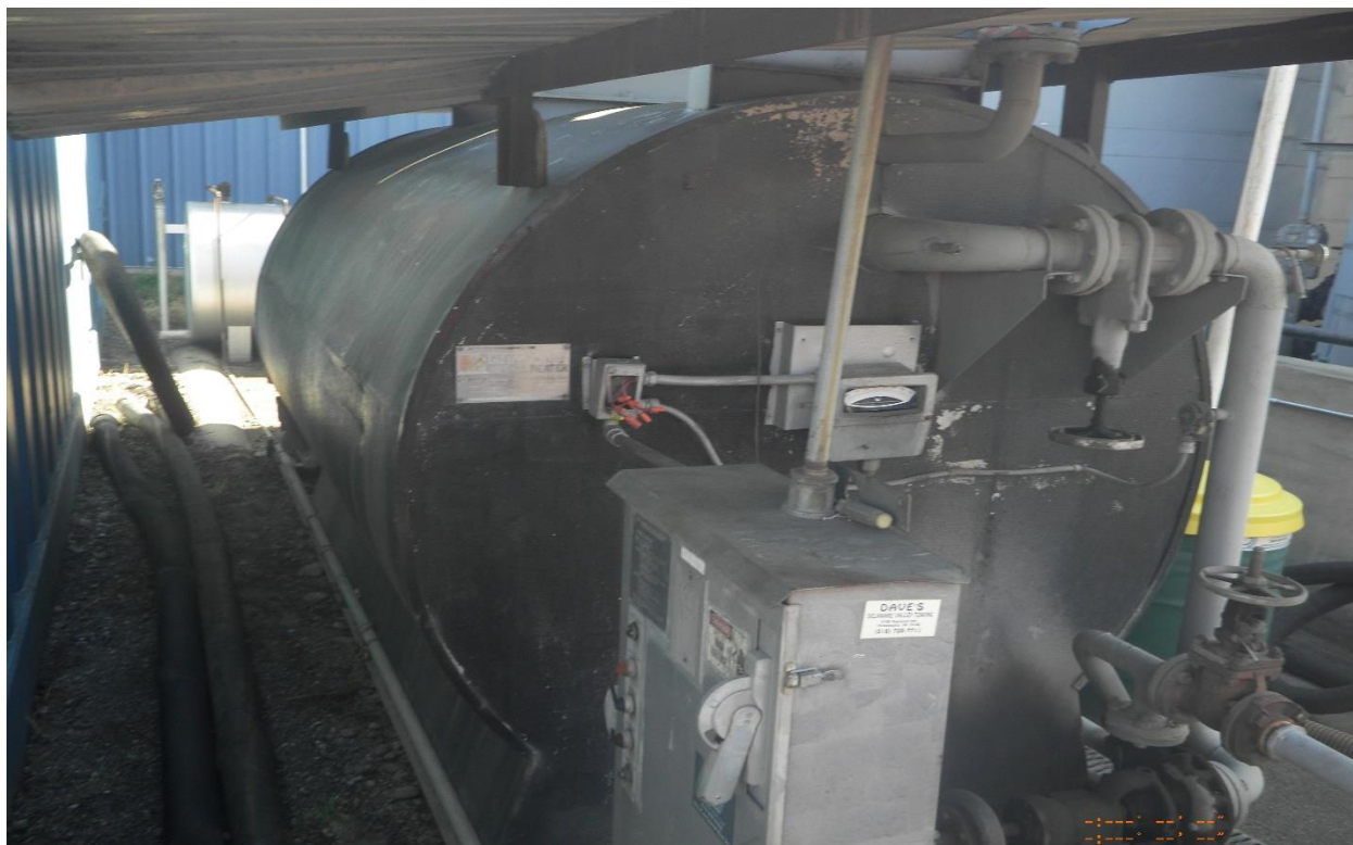
5. HyWay Hot Oil Boiler (not operating) – PRC – 09/14/22
