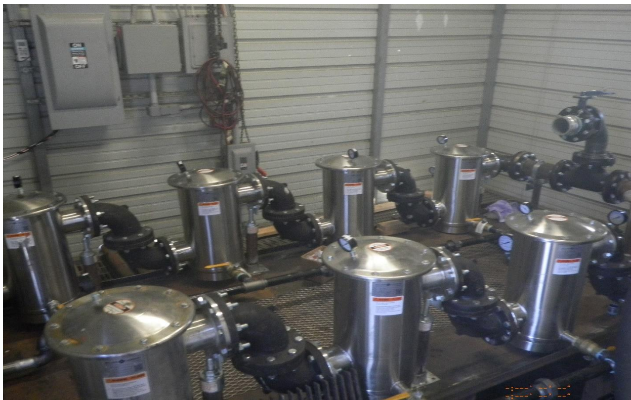
3. New Filter System (not operating) – PRC – 09/14/22
