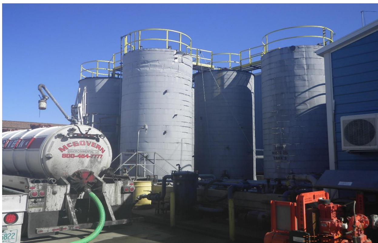
4. Vertical Oil Tanks (Tank 6 front left) – PRC – 09/14/22
