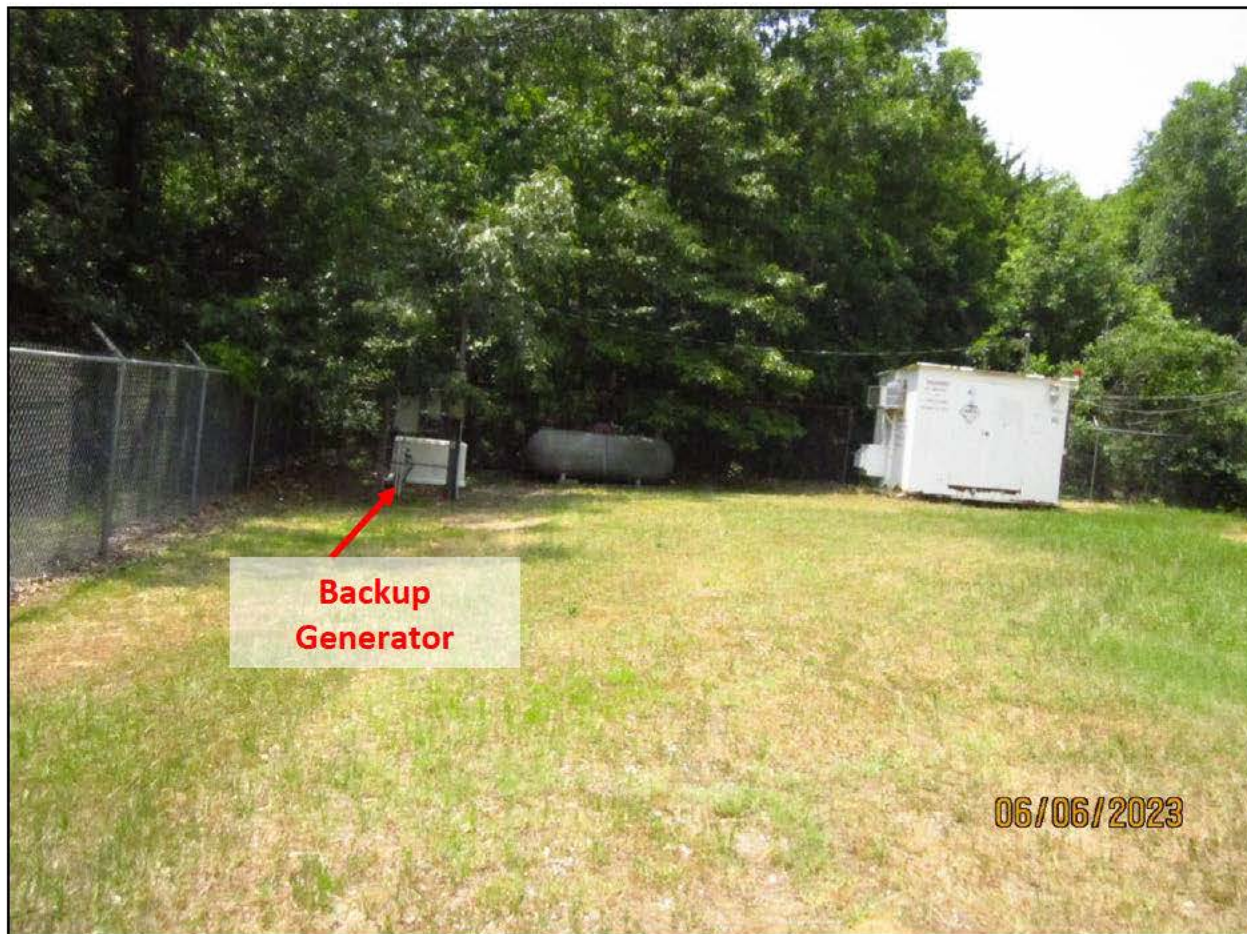
Photograph 9. Backup Generator, Horseshoe Mountain Water Tank View of the backup generator and propane tank that were positioned next to the Horseshoe Mountain Water Tank. System representatives stated that the generator was owned by Community Water. [REDACTED]
