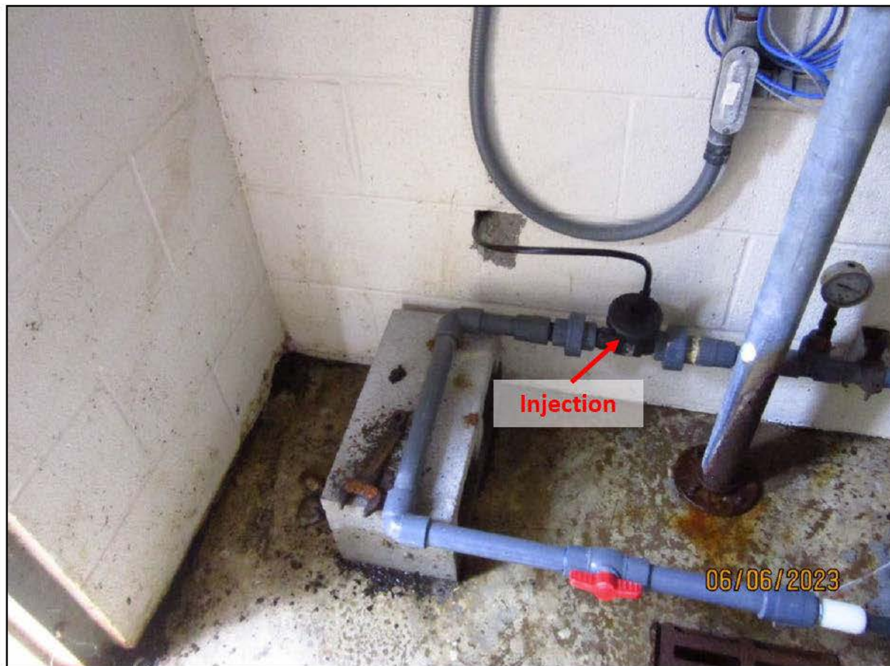
Photograph 27. Chlorine Injection, Master Meter #2 View of the inside of the backflow protection/chlorine injection room where chlorine gas was being injected into carry water. This injection was in a separate room from the chlorine storage room.
