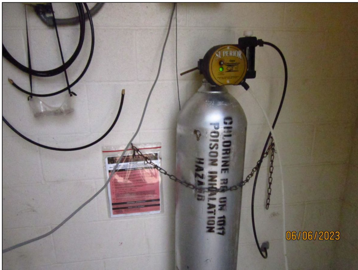
Photograph 23. Chlorine Gas Storage Room, Master Meter #2 View of the 150 lb. chlorine gas cylinder inside the Master Meter #2 chlorine storage room. The gas was being fed through the wall into the backflow protection/chlorine injection room.
