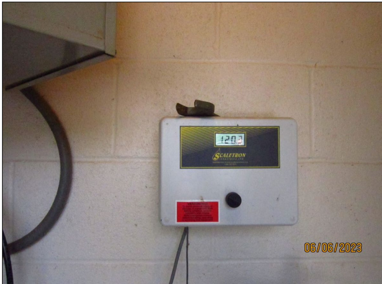
Photograph 26. Chlorine Cylinder Scale, Master Meter #2 View of the functional chlorine cylinder scale in the chlorine gas storage room at Master Meter #2.
