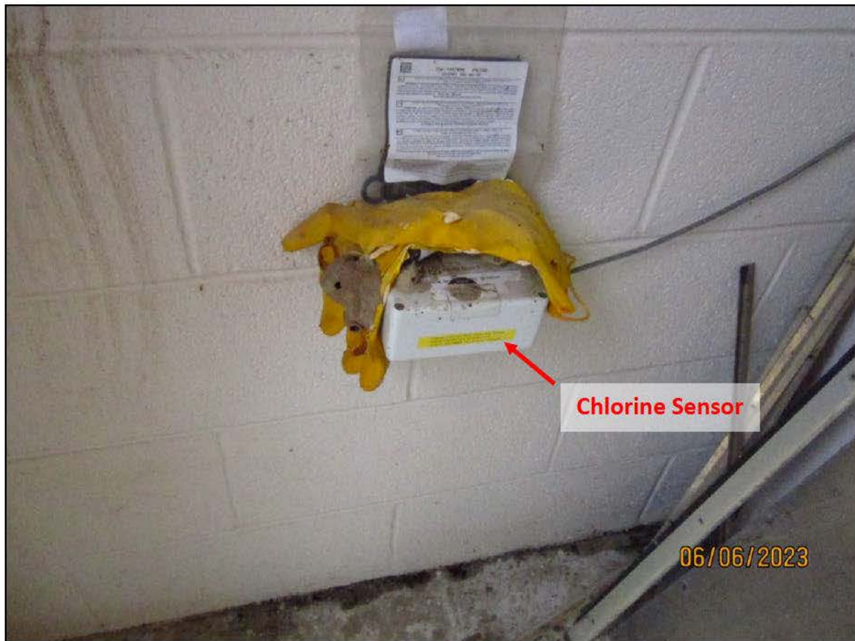
Photograph 17. Chlorine Sensor, Master Meter #1 View of the sensor near the floor of the chlorine storage room at Master Meter #1. It was unclear if the sensor was functional. There was a large wasp nest on top of old rubber gloves that were resting on the chlorine gas alarm sensor, and it appeared that it had not been cleaned/serviced recently. In addition, the sensor was positioned approximately 20-inches off the floor. Since chlorine gas settles close to the ground, the position of this sensor is concerning because it may not detect a chlorine gas leak until levels of chlorine become dangerously high.
