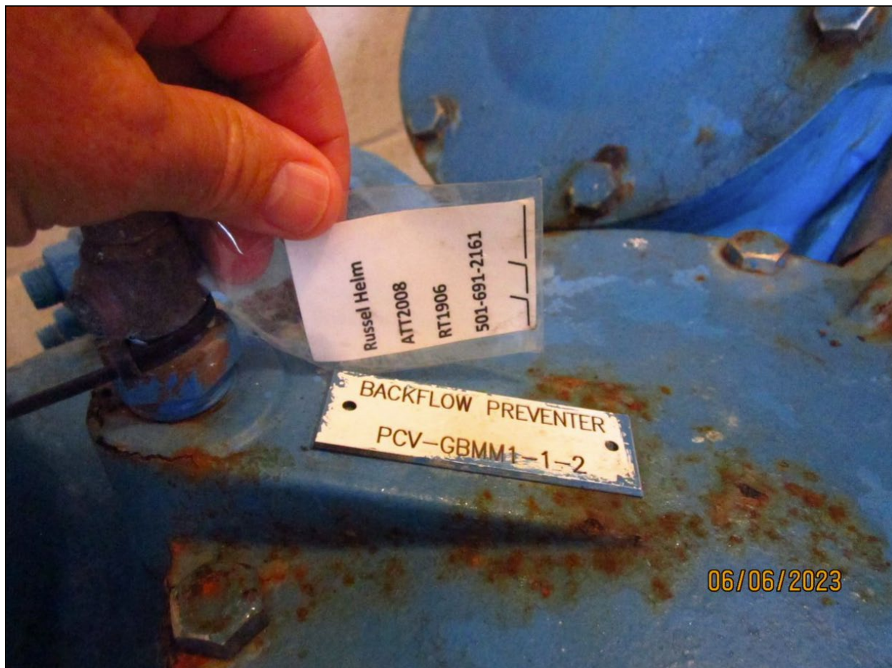
Photograph 20. Backflow Preventer, Master Meter #1 View of the backflow preventer on the Master Meter #1 line that appeared to contain an asset identification nameplate.
