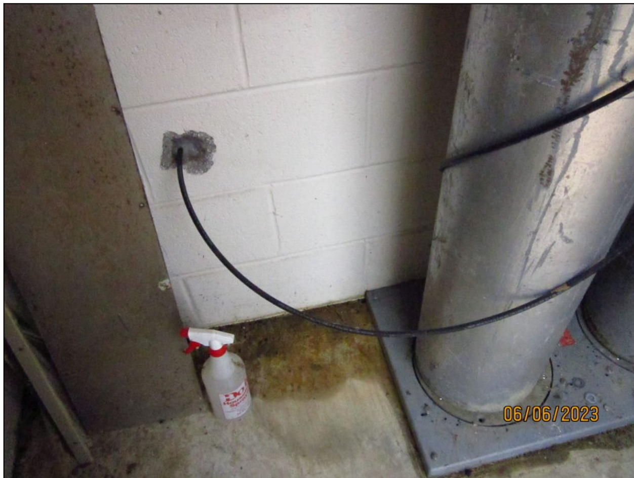
Photograph 15. Chlorine Storage Room, Master Meter #1 View of the chlorine gas line that feeds through the wall into the backflow protection/chlorine injection room where it is injected into carry water before final injection downstream of Master Meter #1.
