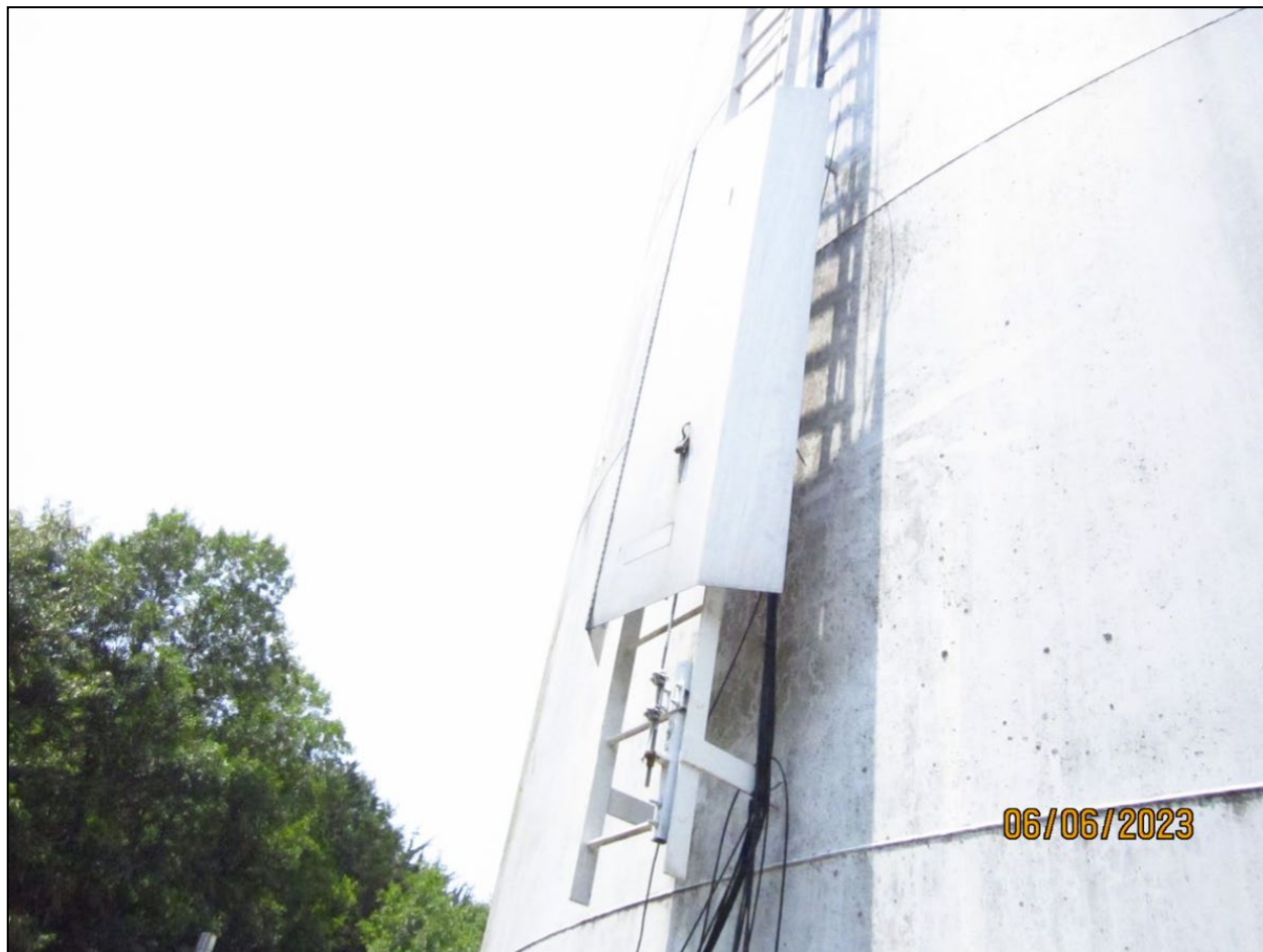
Photograph 8. Horseshoe Mountain Water Tank View the locked security plate over the bottom rungs of the ladder at the Horseshoe Mountain Water Tank.
