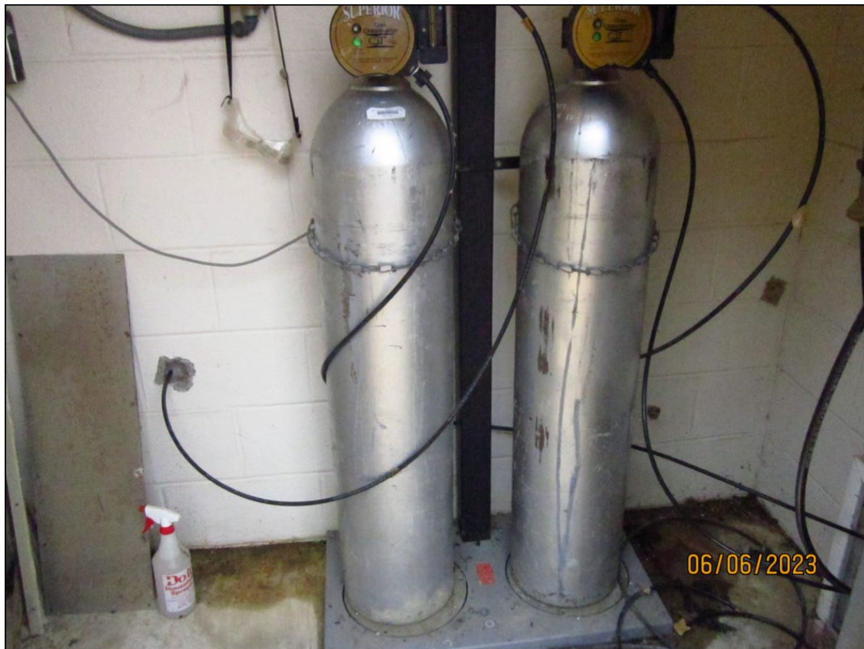
Photograph 14. Chlorine Storage Room, Master Meter #1 View of the inside of the chlorine storage room at Master Meter #1. There were two, 150 lb. cylinders with one in use and one on standby. The chlorinator vent lines were run through an exhaust vent with moveable louvers. It was unclear if the lines will negatively impact the rooms design ability to properly manage a release of chlorine gas.
