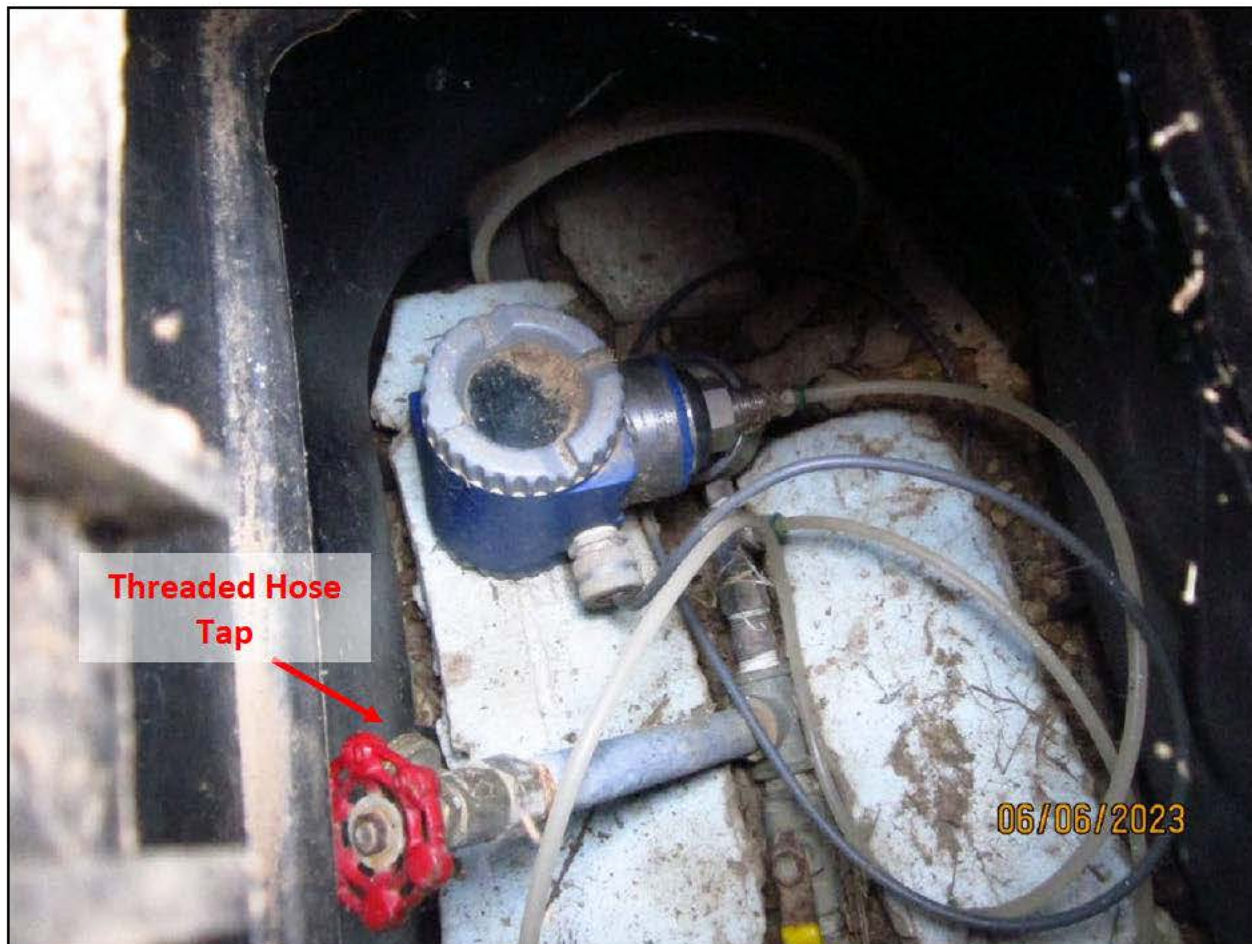
Photograph 4. Valve Box, North Water Tank View of the inside of a valve box at the North Water Tank that contained a pressure gauge indicator and a threaded hose tap without backflow prevention.
