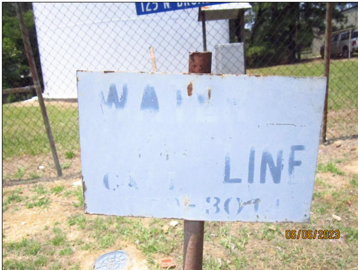
Photograph 2. Security Sign, North Water Tank View of the security sign that was posted in front of the perimeter fence at the North Water Tank. The sign was sun bleached and illegible.
