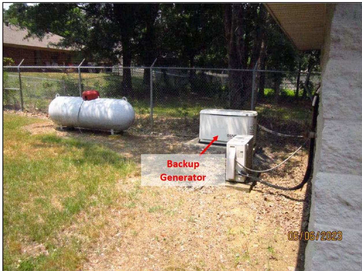
Photograph 21. Backup Generator and Propane Tank, Master Meter #1 View of the backup generator and propane tank that were located inside of fence line at Master Meter #1. System representatives stated that the generator was owned by Community Water.
