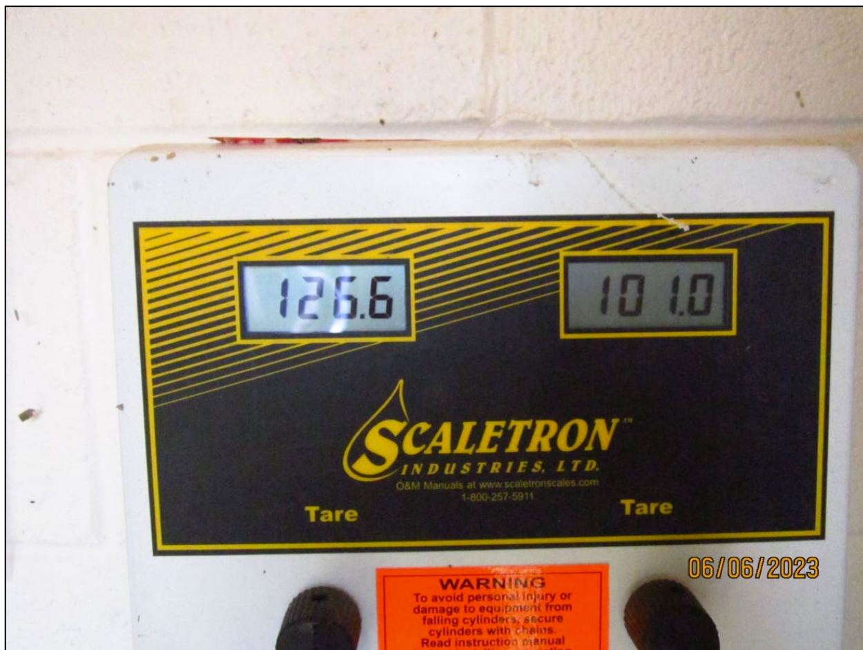
Photograph 18. Chlorine Cylinder Scale, Master Meter #1 View of the functional chlorine cylinder scale in the chlorine gas storage room at Master Meter #1.
