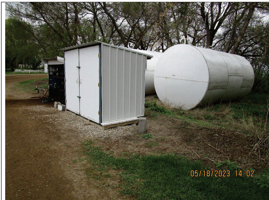
Three large fueling tanks located on site.
