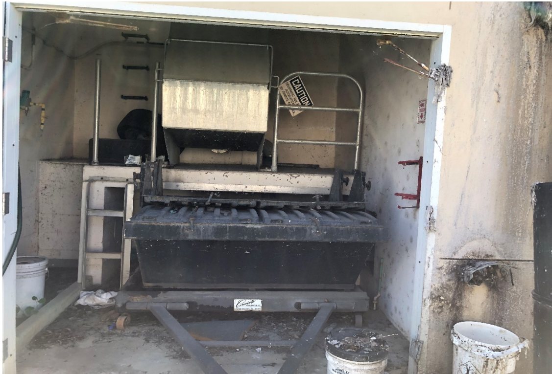
Photo #2. The Grit Removal System has been out-of-service since the 2017 hurricane.
