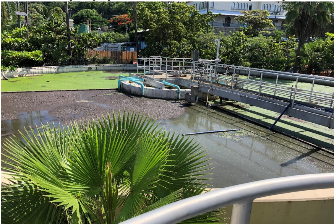
Photo #6. The second packaged plant is out-of-service but receives septic sludge.
