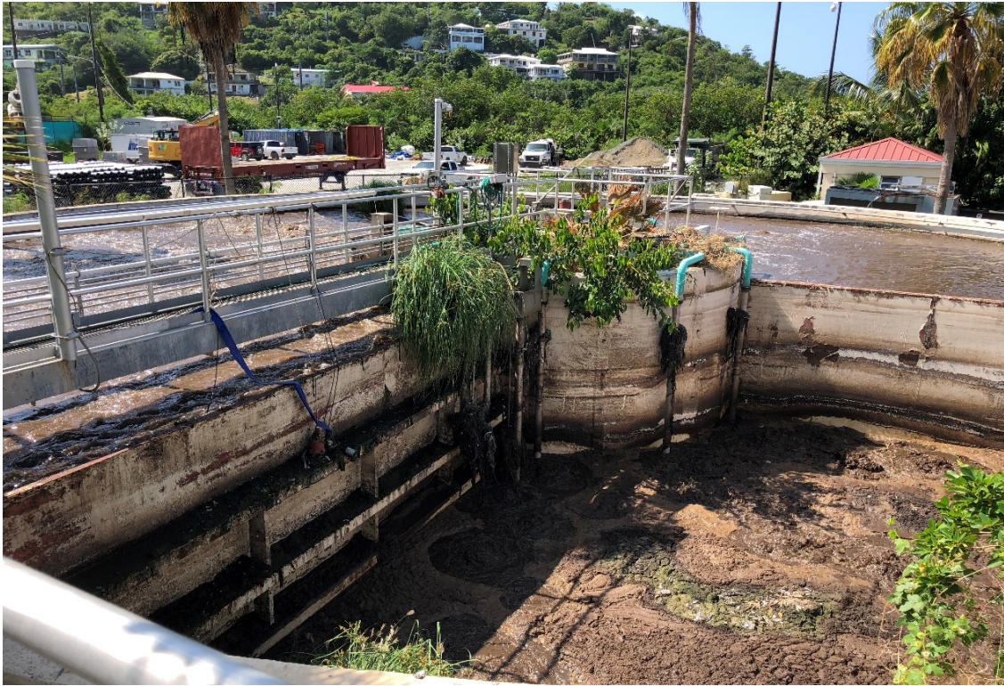
Photo #5. Vegetative growth can be seen in the sludge digester, the circular clarifier & walkway.
