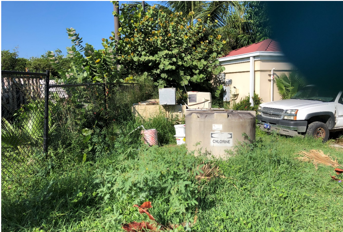
Photo #8. The plant effluent automatic composite sampler has been out-of-service since 2017.
