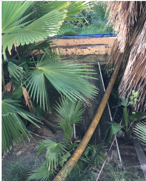
Photo #12. The walkway to the packaged plants landing collapsed during the 2017 hurricane.
