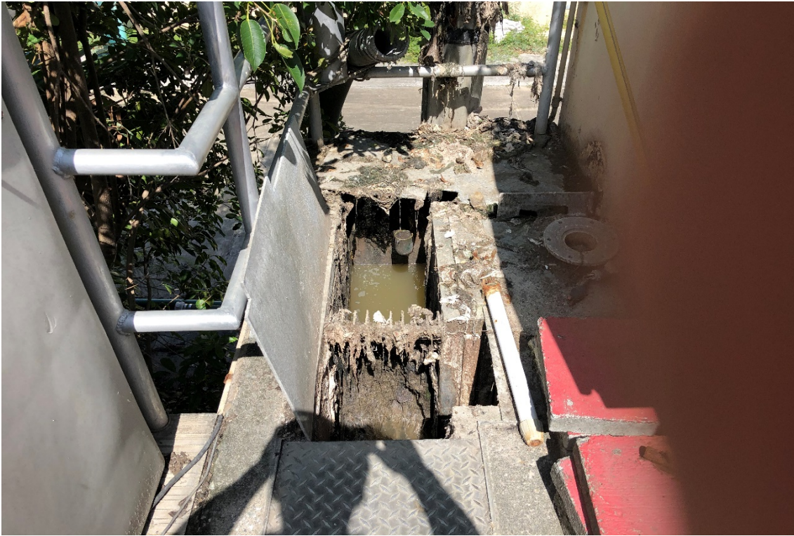
Photo #3. Screenings in the bar screen are restricting downstream flow.
