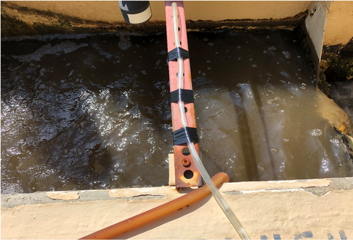
Photo #7. Cruz Bay WWTF effluent discharges into Cruz Bay.
