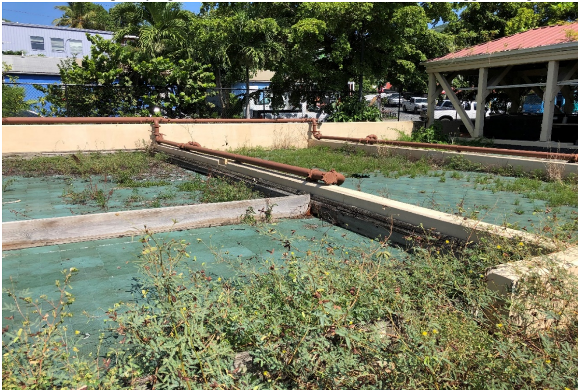
Photo #10. The Sludge Drying Beds have been out-of-service since the clogged sludge line.
