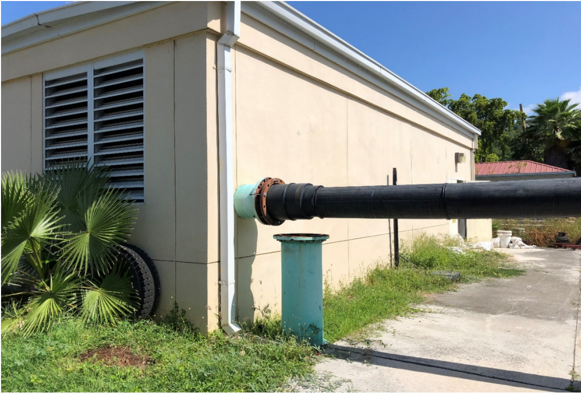
Photo #9. The temporary air-supply line has been in place since 2017.
