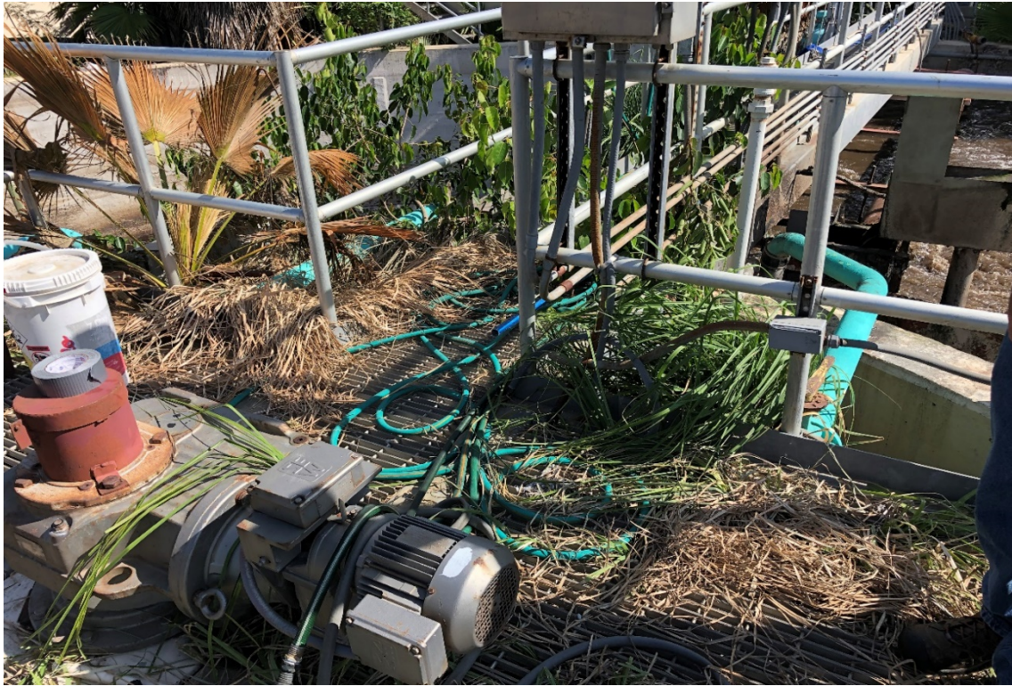
Photo #13. Overgrown vegetation was observed in the circular clarifier and along the walkway.
