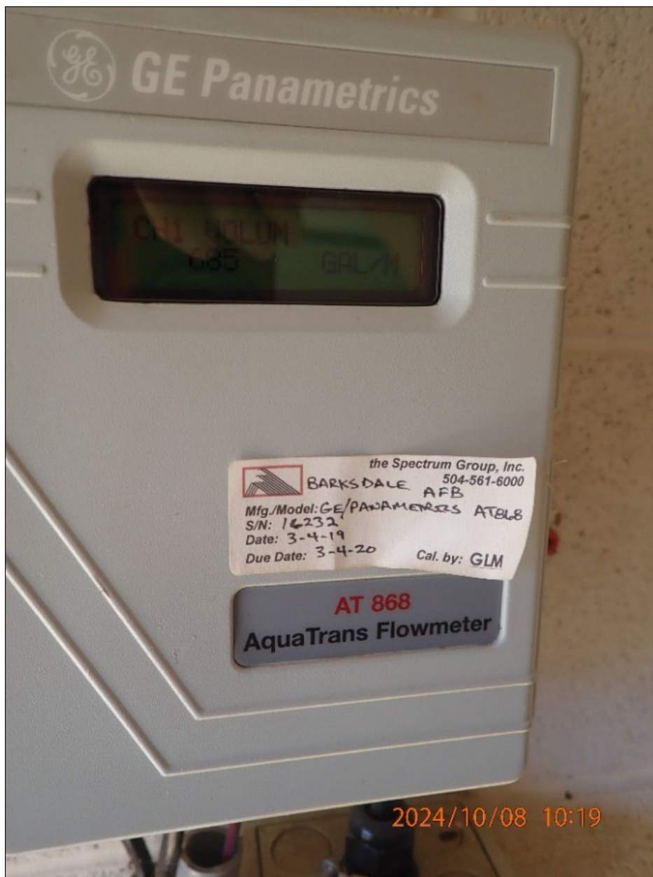
Photograph 2. Treatment Plant at Entry Point 10/08/2024 10:19 PA080185.JPG
