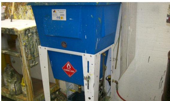
Photograph #5: Paint gun cleaner container without “Hazardous Waste” and indication of hazards “Toxic” label.
