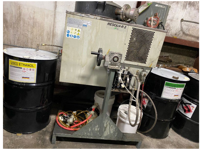
Photograph #10 – Resolv-r 2 solvent recovery system.
