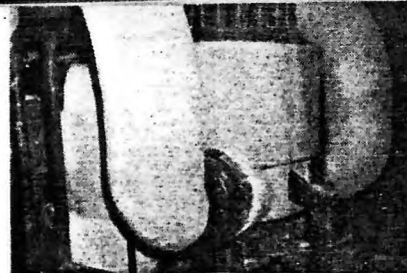
BLOCK AND PLASTIC insulation cover turbine hydraulic throttle valve, strainer
