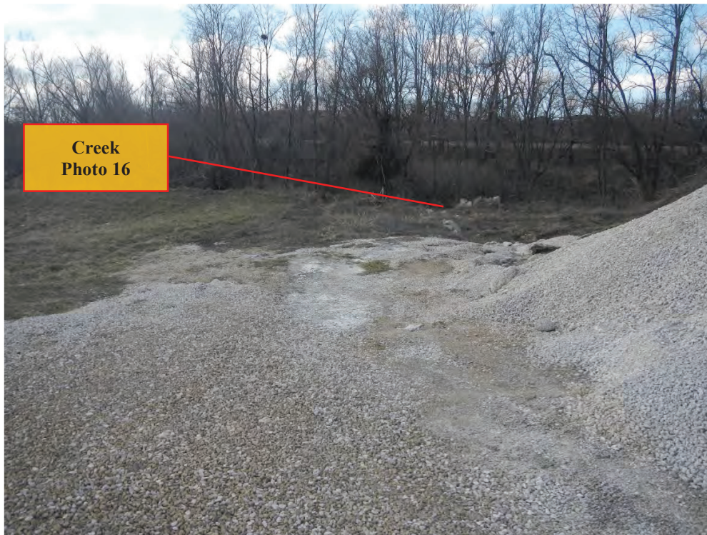
Photo 22, Concrete washout runoff toward the Creek
