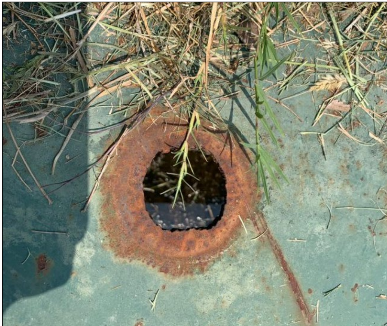
Photograph 6. Master Meter #2 Vault View of a hole in the surface of the Master Meter #2 vault caused by corrosion and metal loss.
