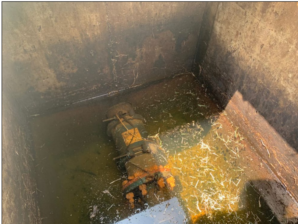
Photograph 7. Master Meter #2 Line View the Master Meter #2 line that was completely submerged. The wiring associated with the meter telemetry was also fully submerged.
