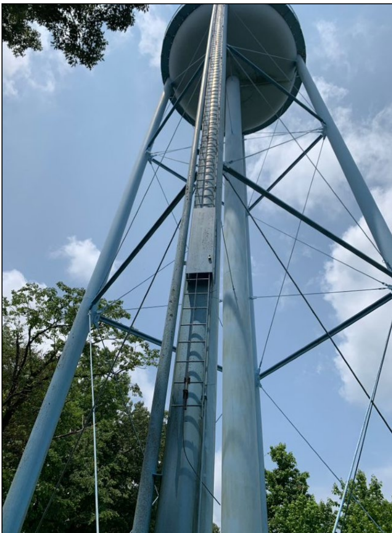
Photograph 21. Security Ladder, West Point Water Tank View of the security ladder and ladder shield at the West Point Water Tank. The ladder shield was locked, and the bottom rungs of the ladder were removed.
