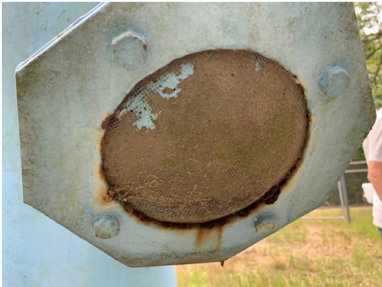
Photograph 20. Overflow Pipe, West Point Water Tank Close up view of the screen covering the end of the overflow pipe at the West Point Water Tank. The screen was mostly covered with debris that was clogging the mesh screen.
