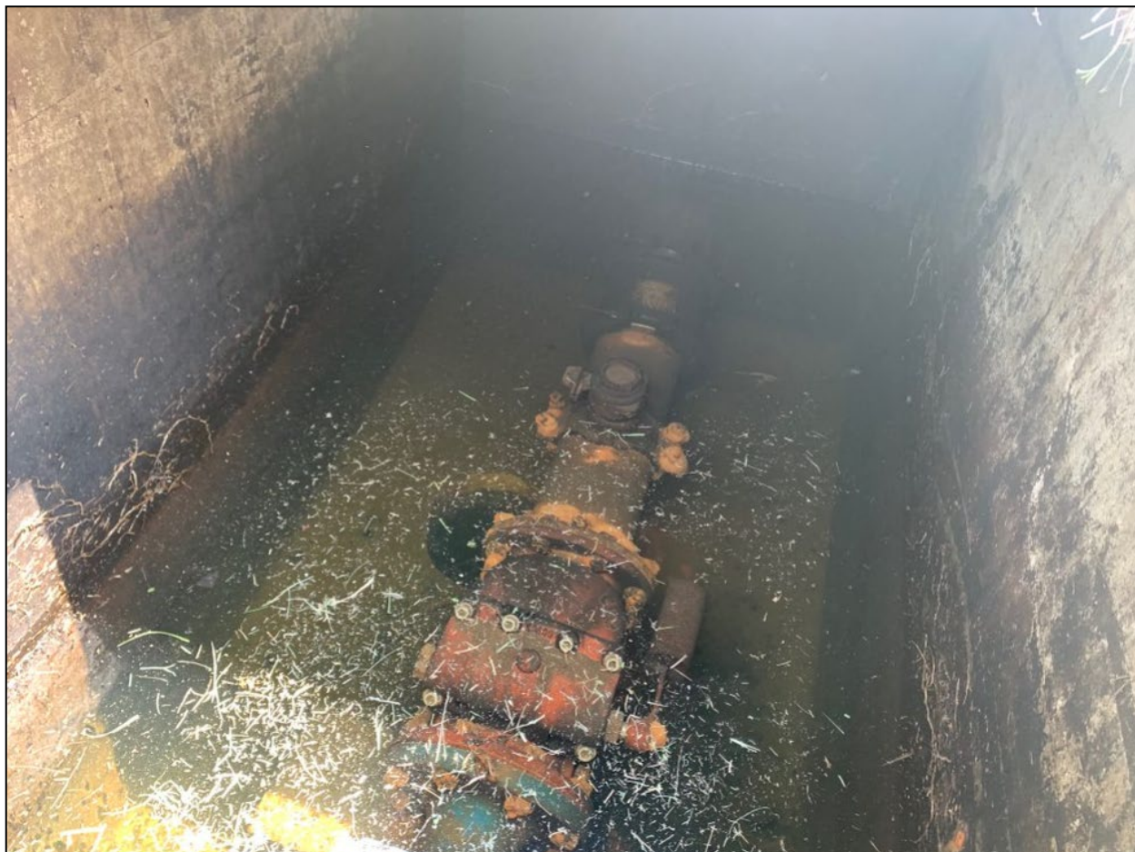
Photograph 8. Master Meter #2 Line Alternate view of the fully submerged Master Meter #2 line.
