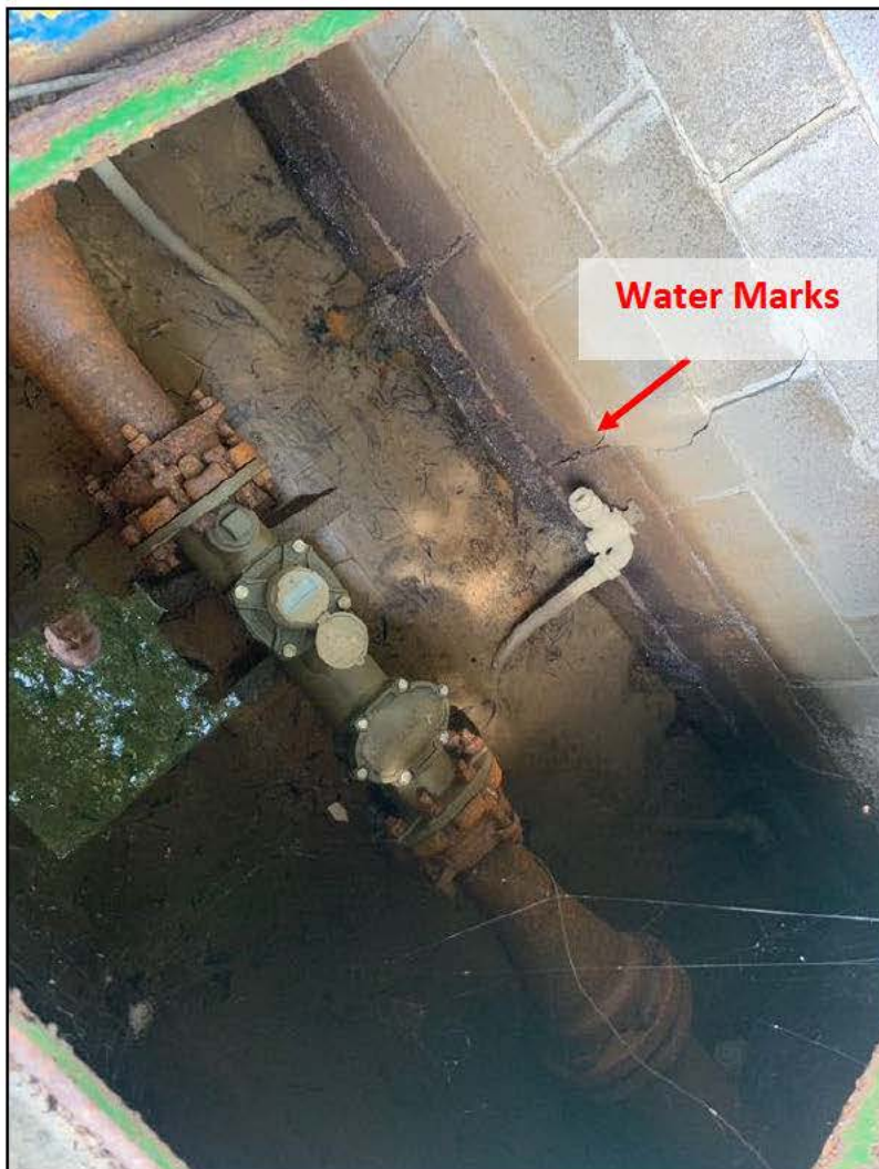
Photograph 3. Master Meter #1 Line View of the Master Meter #1 Line. Water marks on the wall show that the water level had been higher than the meter line at some point.
