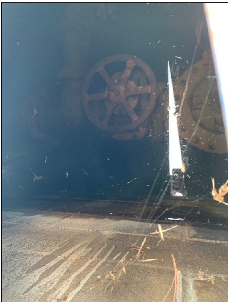
Photograph 29. Valve Vault, Griffithville Water Tank View of the inside of the valve vault at the Griffithville Water Tank. The vault was flooded, and the valves were completely submerged. The sump pump that was typically used to empty the valve vault was not functional.
