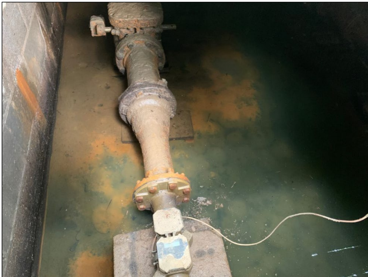
Photograph 13. Master Meter #3 Line View of the water flooded below the Master Meter #3 line. There were approximately four inches of water below the line.
