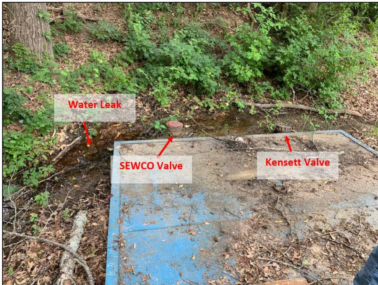
Photograph 10. Kensett Water and SEWCO Valves View of the City of Kensett Water valve and the SEWCO Master Meter #3 valve that can be used to shut off water supply from Searcy Waterworks. There was a leak coming through the ground, but it was unclear if the leak was coming from a line or one of the valves.
