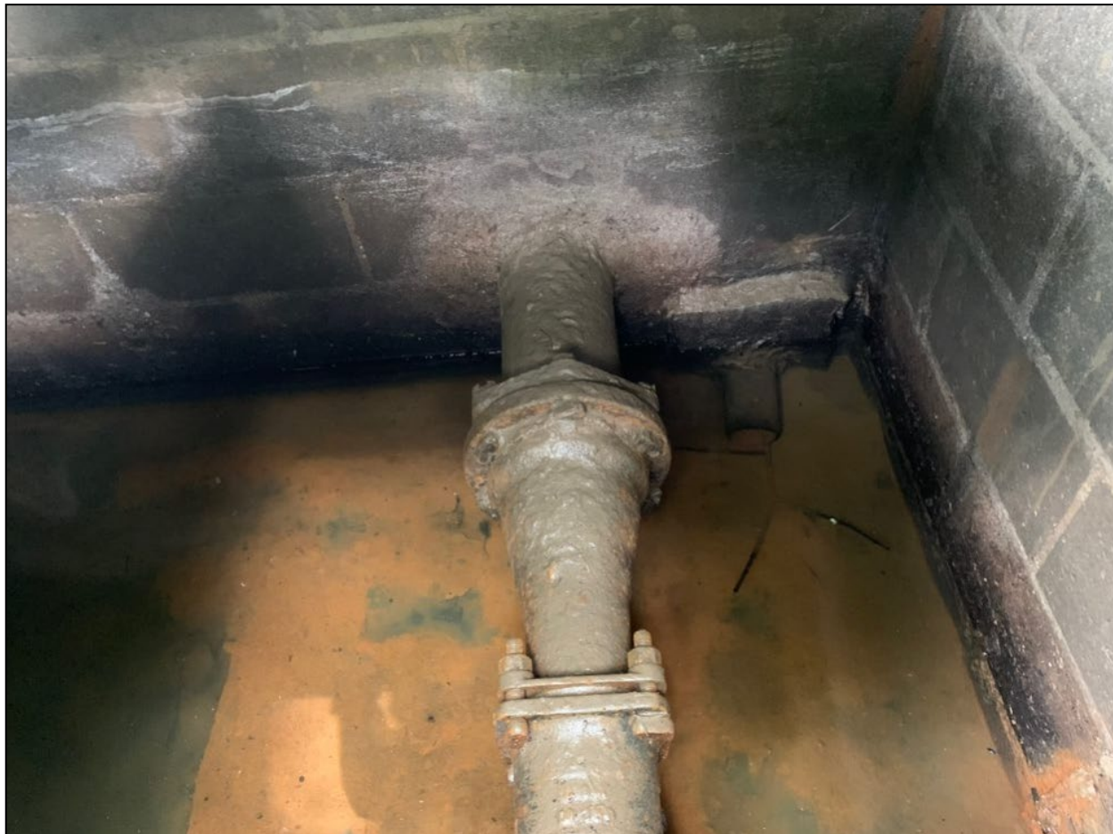
Photograph 14. Master Meter #3 Line Alternate view of the Master Meter #3 line which had approximately four inches of water beneath it.
