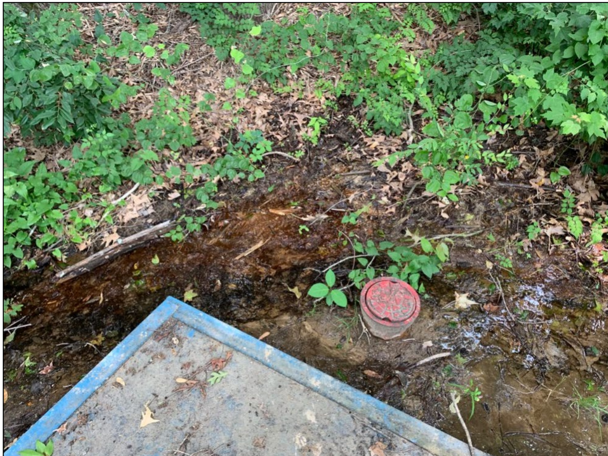
Photograph 11. Water Leak, Master Meter #3 Close up view of the water leak upstream of Master Meter #3. It was unclear where the leak was coming from.
