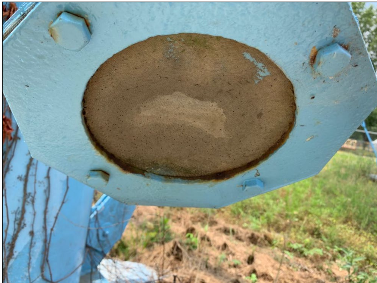
Photograph 26. Overflow Pipe, Griffithville Water Tank View of the mesh screen covering the end of the overflow pipe at the Griffithville Water Tank. The screen was mostly clogged with debris.
