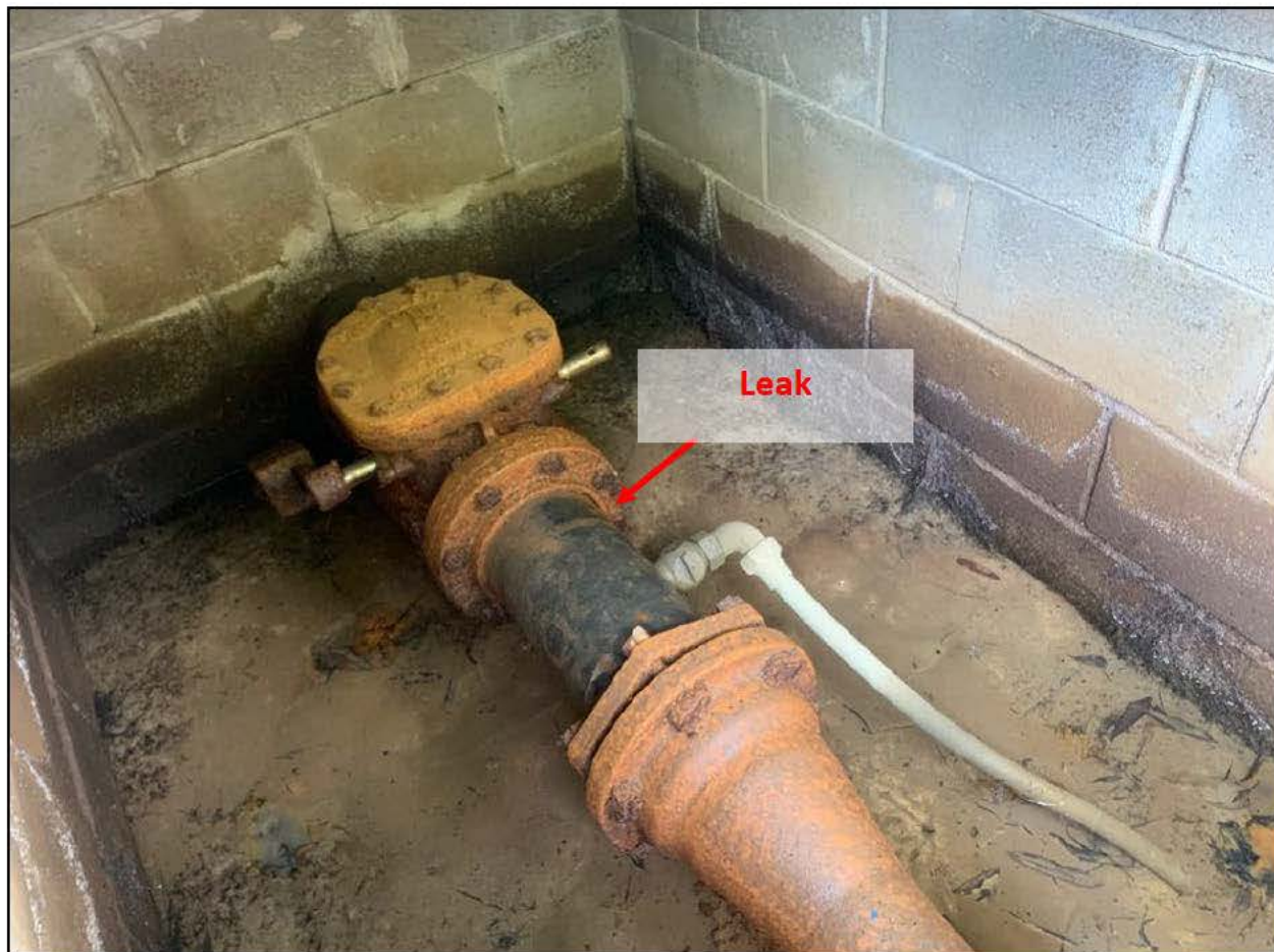
Photograph 2. Master Meter #1 Line View of the Master Meter #1 line. There were approximately five inches of water below the line, and water was dripping constantly from the line downstream of the meter.
