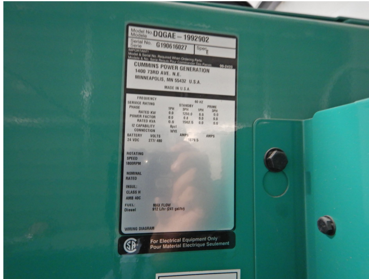
Photo 5 – Line 1 emergency generator plate
