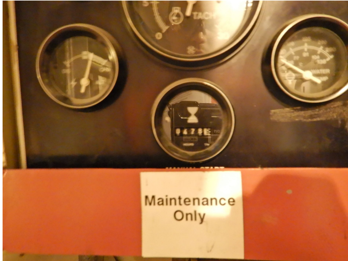
Photo 1 – Line 1 emergency generator hour meter
