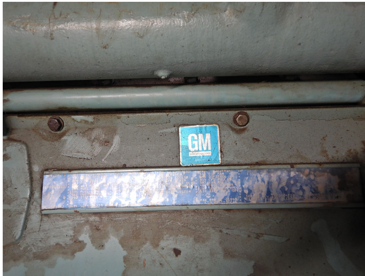
Photo 3 – Mobile generator plate
