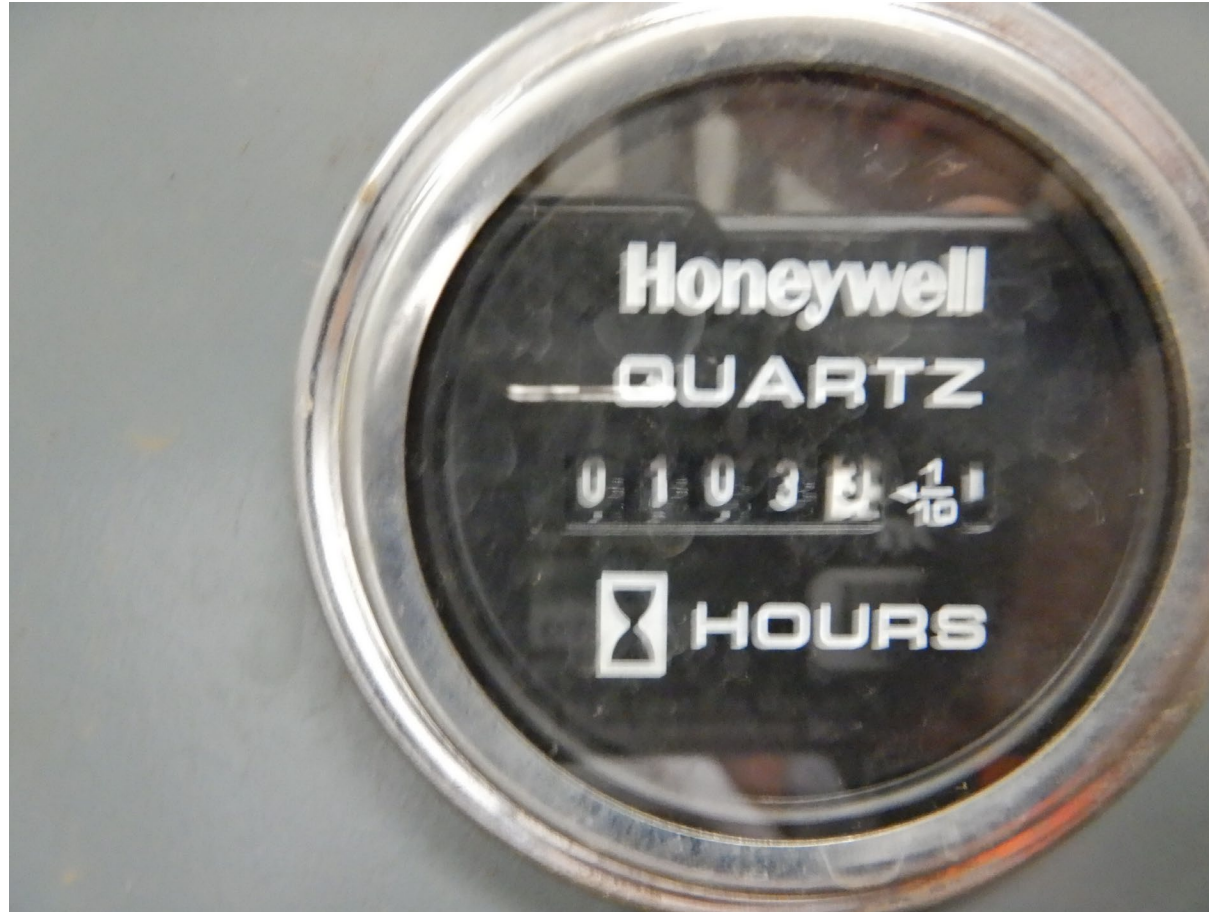
Photo 23 – 29 HP Fire pump hour meter
