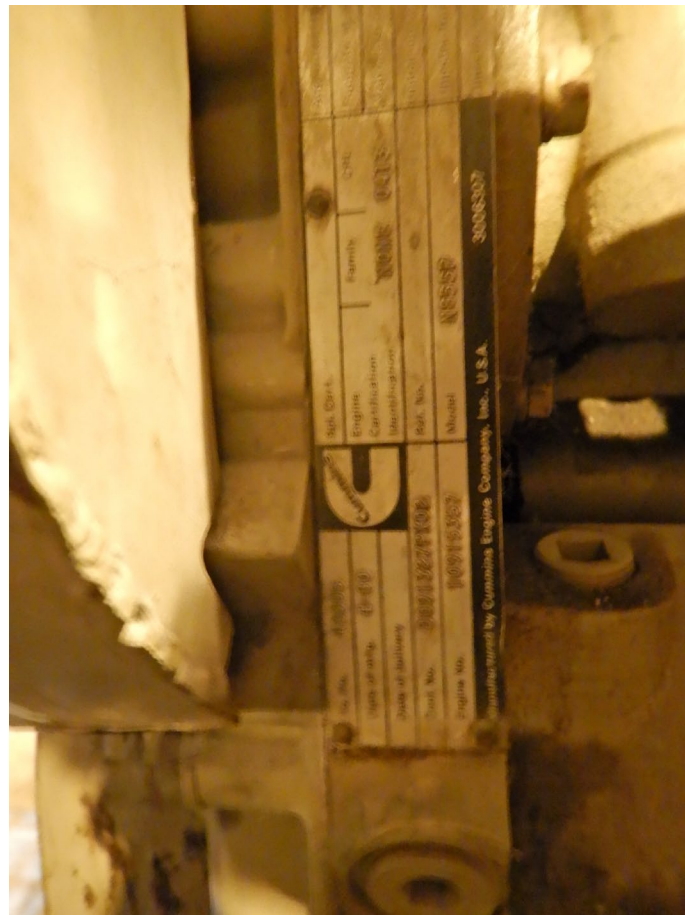
Photo 26 – Mill use emergency generator plate
