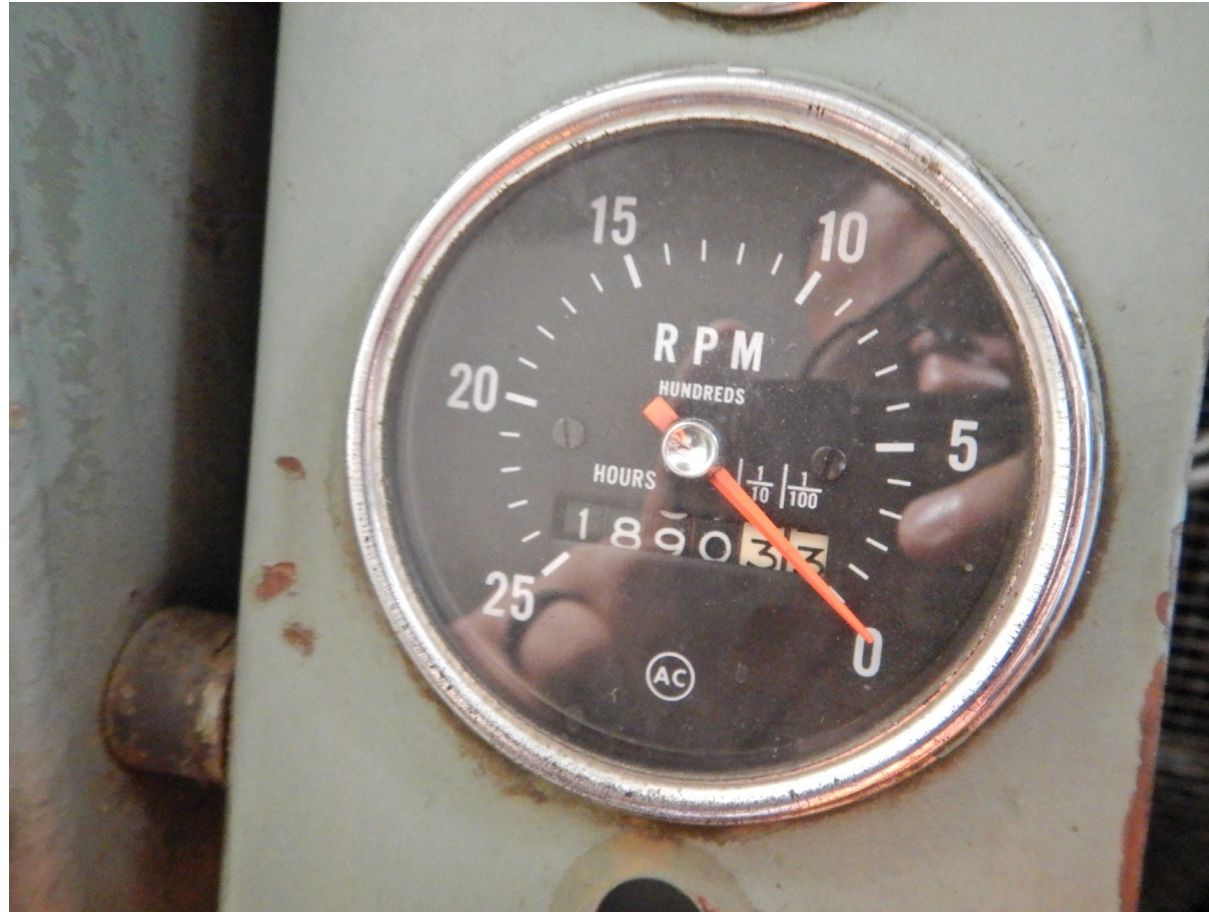
Photo 2 – Mobile generator hour meter
