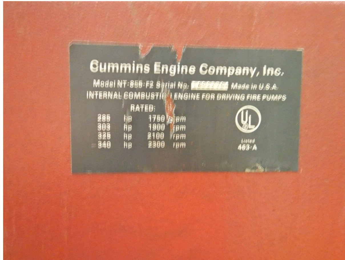
Photo 21 – 340 HP fire pump plate retake
