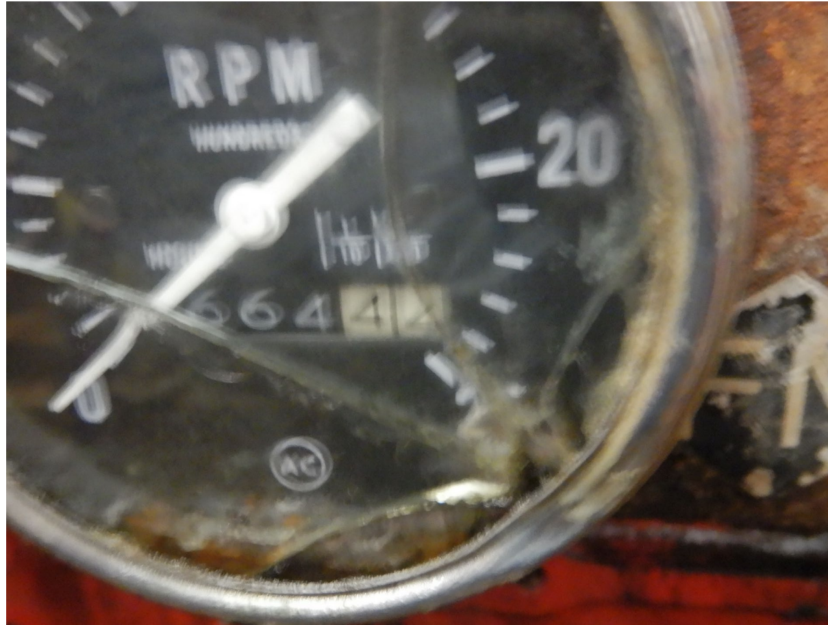
Photo 24 – 340 HP Fire pump hour meter
