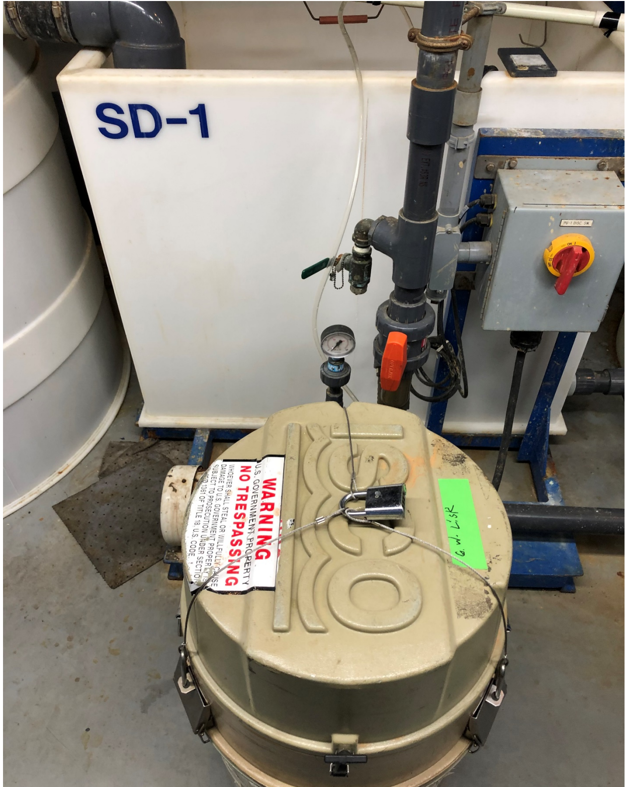
Photo #2: View of Tank SD-1, where discharge effluent samples were collected.
