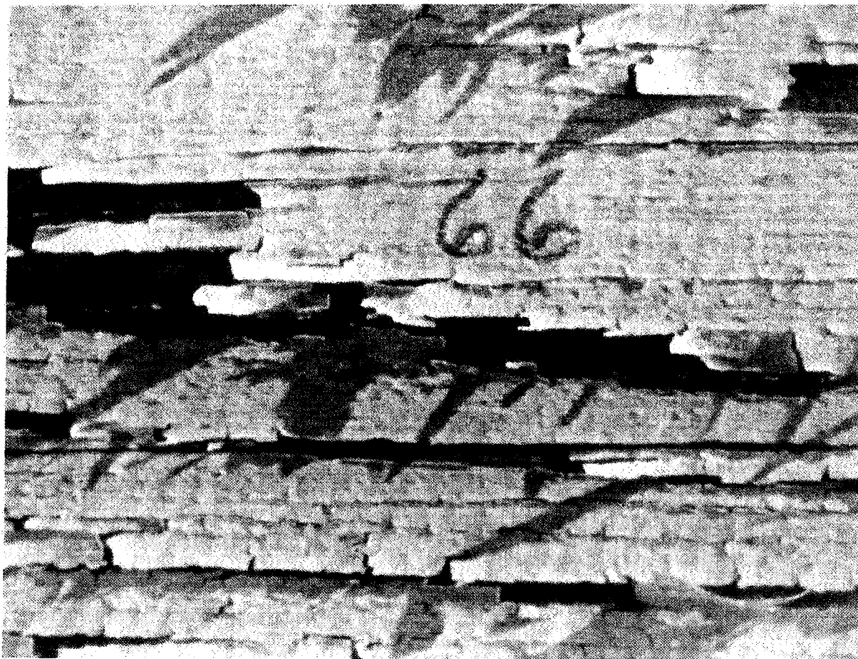
Figure 89. Severe Cracking, Curling and Flaking.
