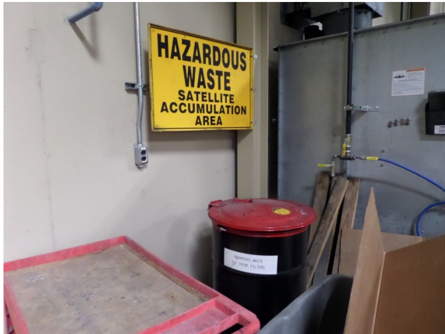
Photograph 8: Spent paint spray booth filters (D001) accumulation container observed in the Bushings Manufacturing Area. The container was neither marked nor labeled with an indication of the hazards of its content.
