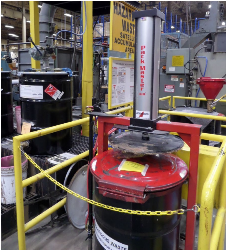
Photograph 4: Spent paint spray booth filters (D001/D008) 55-gallon accumulation container in the Cable Accessories Production Area. The container was neither marked nor labeled with an indication of the hazards of its contents.
