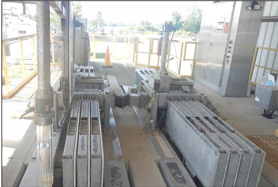
Photo 5. Trojan UV disinfection system (nonoperational).
