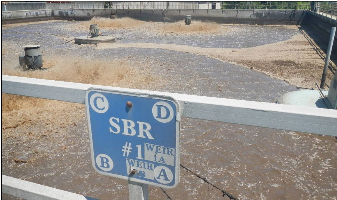
Photo 1. SBR #1 reactor basin. August 20, 2024
