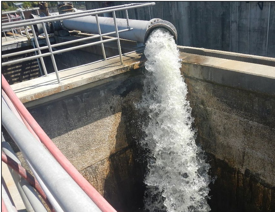
Photo 6. Reactor basin outfall to the post equalization basin.
