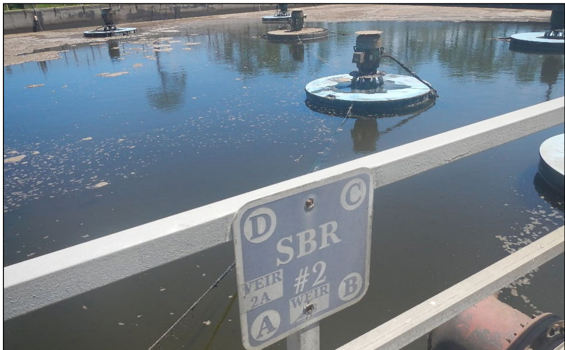
Photo 2. SBR #2 reactor basin. August 20, 2024
