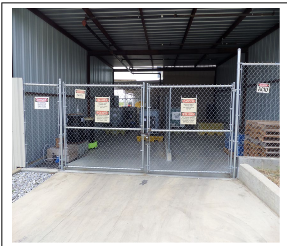
Hager. Acid and Alkaline Hazardous Waste Storage Area – 90-Day. Front view of 90-Day. Photograph 11 taken at 11:01 a.m.
