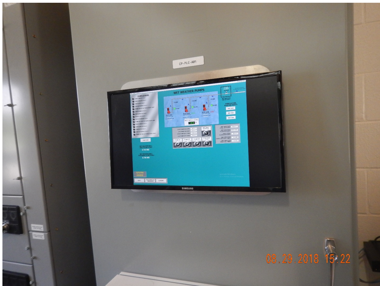
Photo File Name: Sunnymead EQ Basin Building SCADA example (SCADA typical of all City EQ basins). Photographer: DLM
