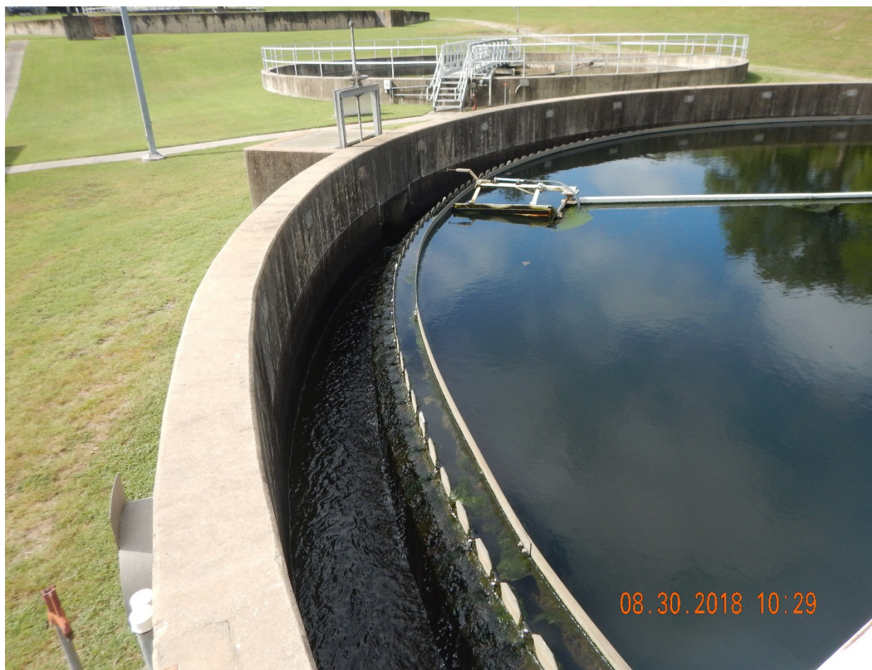
Photo File Name: Secondary Clarifier Effluent Baffle and Weir Photographer: DLM
