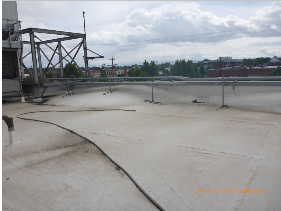
Photograph 32. View of the roof of the main production building. Milk powder residue and dust was observed on the roof in this location.
