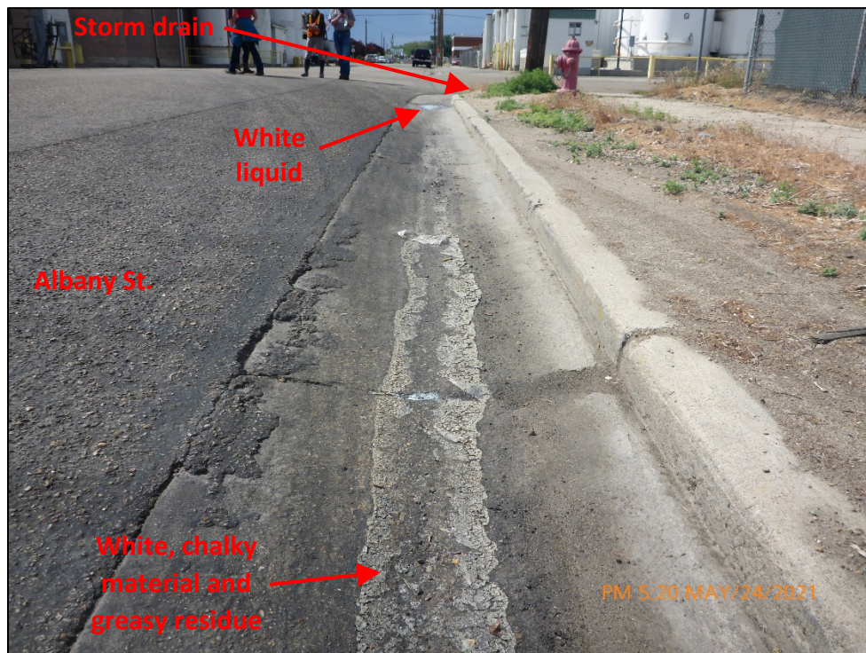
Photograph 20. View, facing northwest, of dried white, chalky material and greasy residue in gutter line of Albany St., upgradient of white liquid and storm drain shown in Photograph 19.
