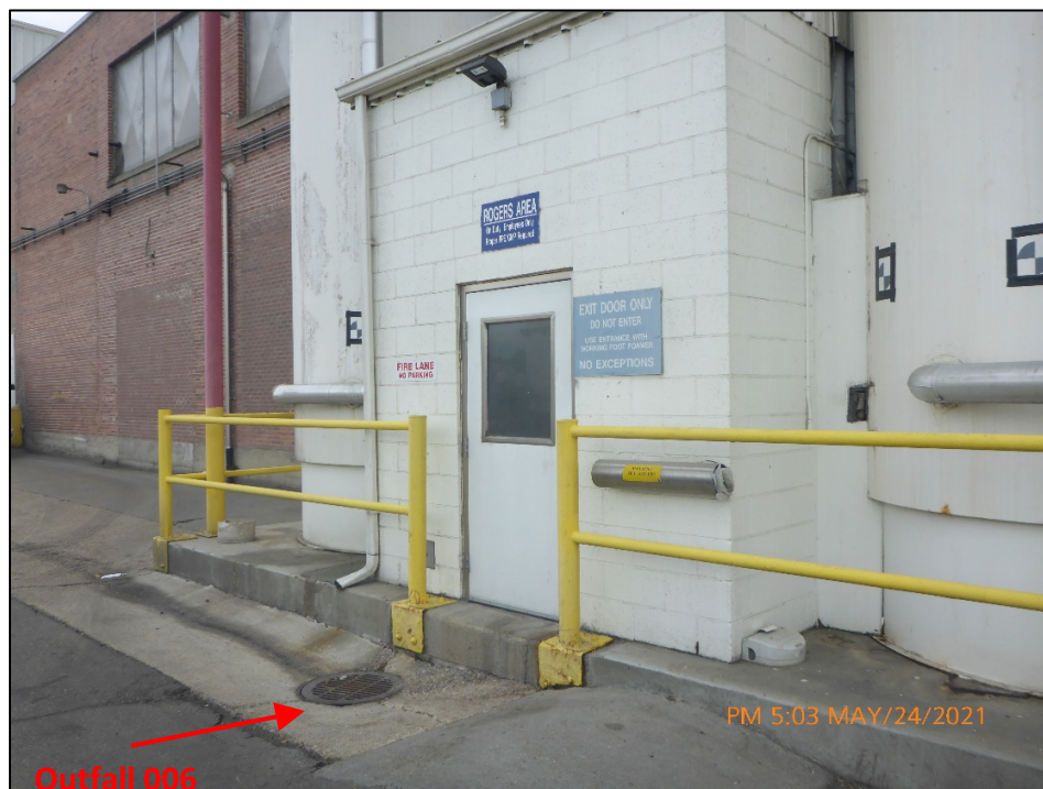
Photograph 12. View of the existing storm drain/outfall identified on the Facility's 2021 MSGP NOI as Outfall 006. Multiple inspection reports (starting with March 5, 2020 inspection) have identified a corrective action to berm this Facility entrance to prevent a spill of process water from inside the main production building from discharging to this storm drain; however, this corrective action had not been completed.
