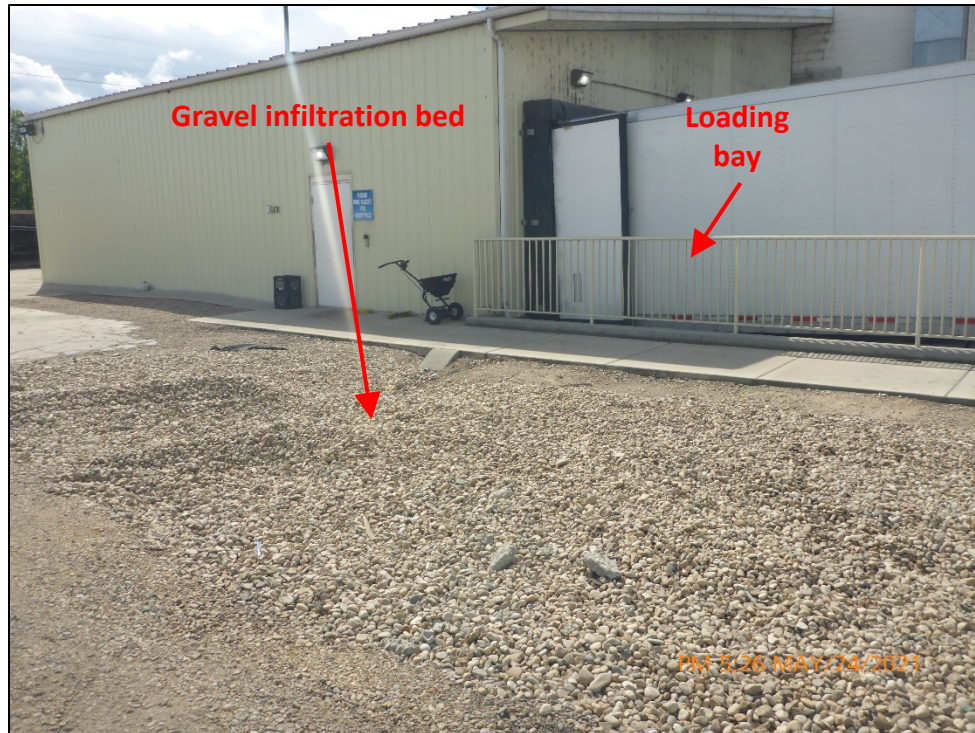
Photograph 15. View of the gravel infiltration bed which receives stormwater runoff from the adjacent loading bay storm drain (previously referred to by the Facility as Outfall 003).
