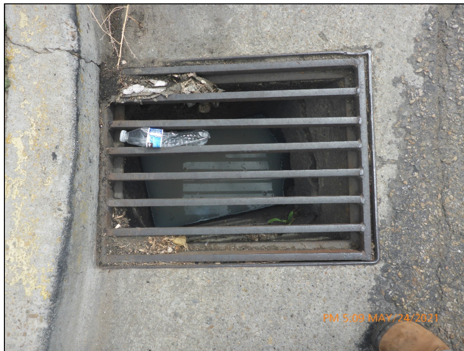
Photograph 24. Close-up view of the storm drain inlet at Albany St. and N. 6 th Ave. shown in Photographs 19, 20, 22, and 23. Note the trash in the grate inlet and the white liquid in the storm drain catch basin.
