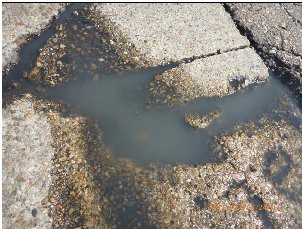
Photograph 28. Additional close-up view of the wash water in the gutter line of Albany St. as shown in Photographs 26 and 27.
