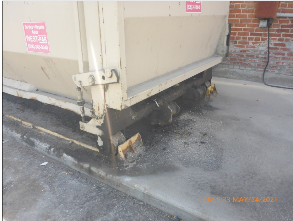
Photograph 38. View of dark staining on the impervious surface under the Facility's trash compactor located immediately upgradient of Outfall 005, as shown in Photograph 10 and 33. Note the absorbent material that had previously been applied to fluid underneath the compactor but which had not been cleaned up at the time of the inspection.
