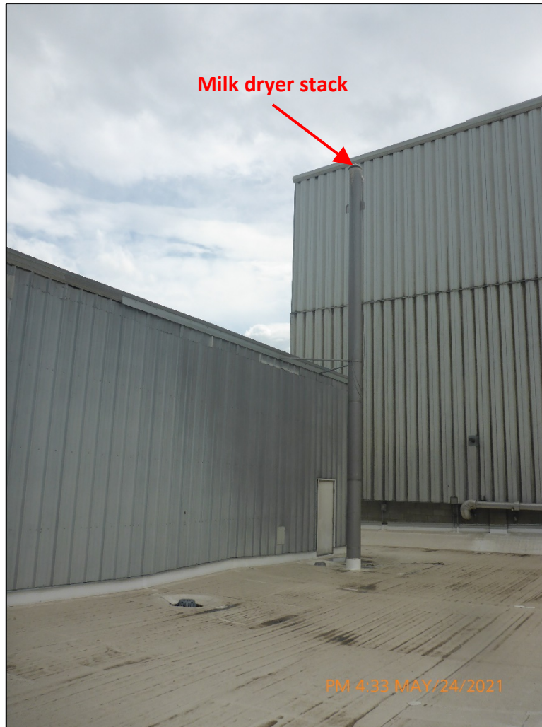
Photograph 29. View of a stack that services one of the Facility's two milk dryers. Powdery residue accumulated on the roof was attributed to milk powder released from this stack, as well as other stacks and receiving vents in this portion of the main production plant roof.
