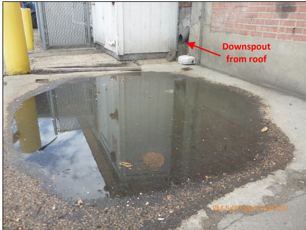
Photograph 13. View of a roof downspout that discharges to Outfall 006 shown in Photograph 12. Note the evidence of recent precipitation.
