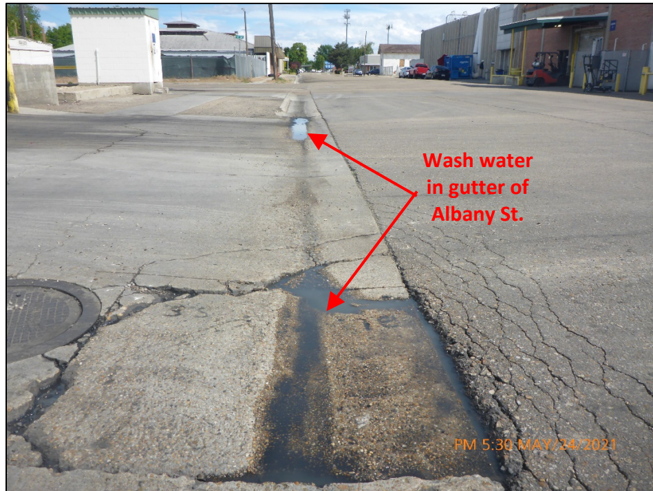
Photograph 27. Close-up view of the wash water in the gutter line of Albany St. as shown in Photograph 26.
