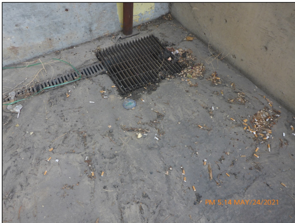
Photograph 8. Close-up view of sediment, grit, trash, and cigarette butts accumulated around the loading bay storm drain (Outfall 002 sample point) shown in Photograph 7. Note the drain was labeled with a storm drain placard.
