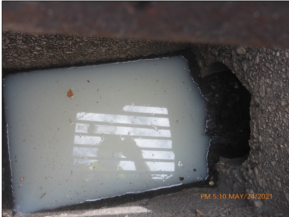
Photograph 25. Close-up view of white liquid in the catch basin of the storm drain at Albany St. and N. 6 th Ave. shown in Photographs 19, 20, 22, 23, and 24.
