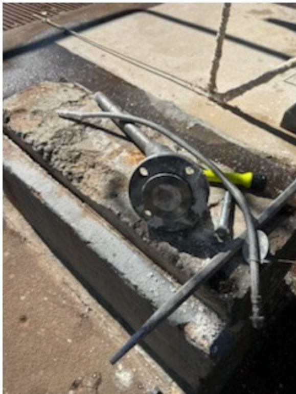
Photo 2: An approximately 2.5-foot piece of piping that is plugged with F002 hazardous waste on the pavement near the 55-gallon container in the PEKK Process Area SAA.
