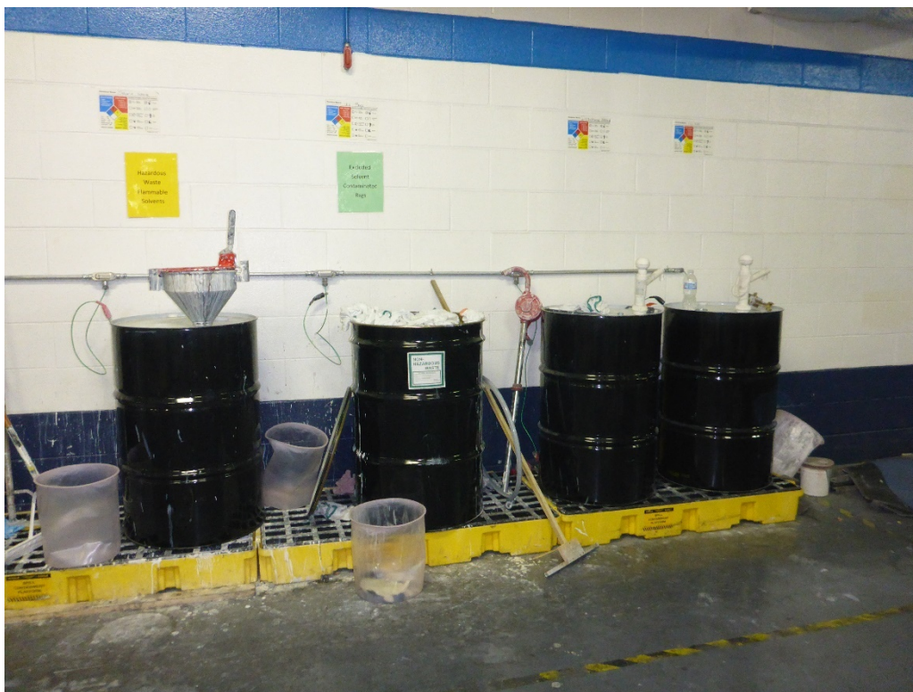
Photo 2: Four of five 55-gallon drums staged on portable secondary containment pallets in the UV Paint Coating Area along the wall just outside of the Paint Mixing Room. The drum on the left was identified for accumulating hazardous waste flammable solvents; second drum from the left was identified for accumulating excluded solvent contaminated disposable wipes; the second drum from the right was identified as denatured alcohol; and the drum on the right was identified as acetone.
