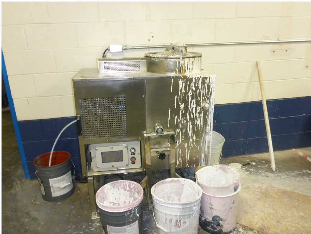
Photo 4: Solvent distillation unit found in the reclaim room. The bucket on the left is used to accumulate recovered solvent for reuse on-site. The three 5-gallon buckets in front of the machine contain an unknown material and may be used to load spent solvents into the machine and/or unload solvent sludge from the machine.
