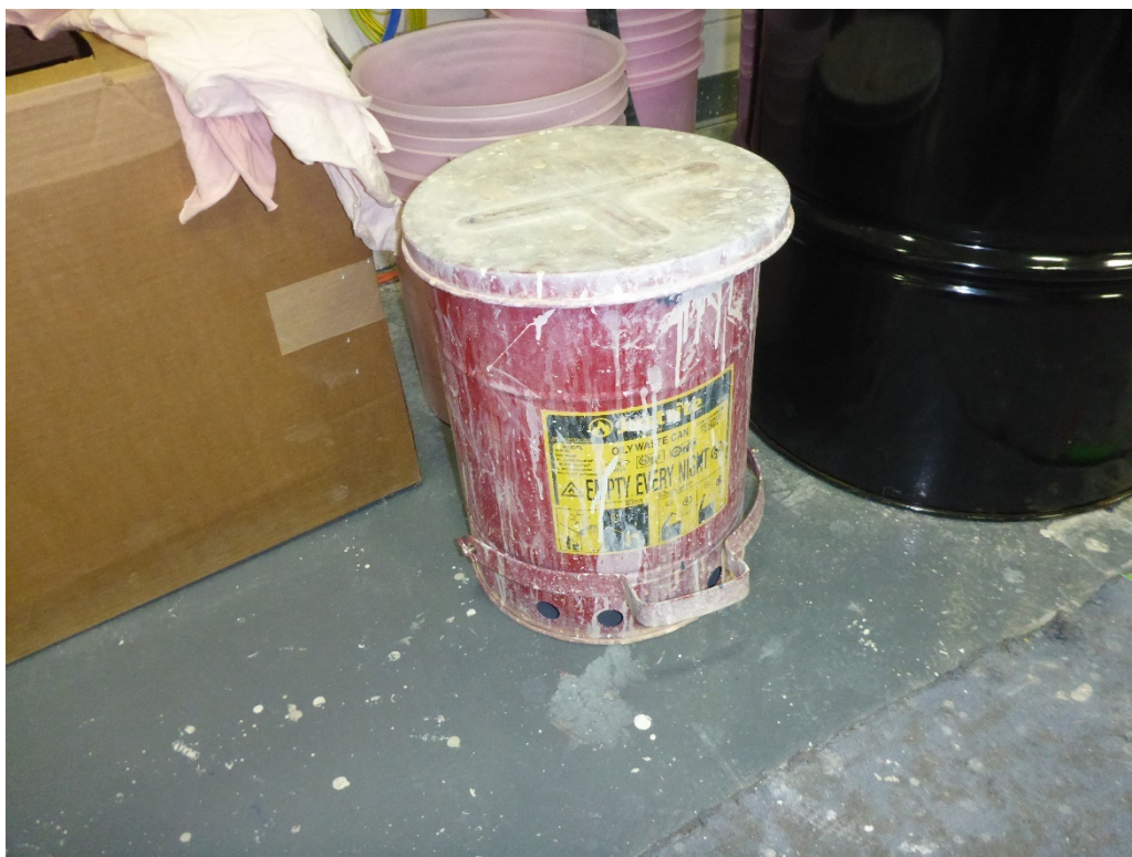
Photo 16: One 5-gallon step-open flammable can for accumulating excluded solvent contaminated disposable wipes at the first solvent paint spray line. The container is labeled as “oily waste” and “empty every night.” It is not labeled as excluded solvent contaminated wipes.
