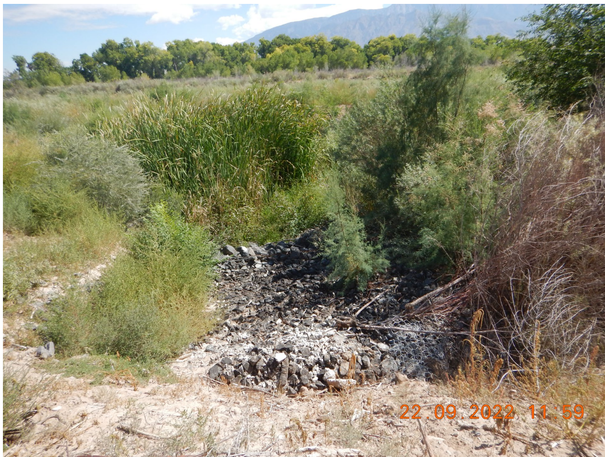
View of the original Outfall 001. Note: the riprap and extensive vegetative overgrowth. (DSCN2333). Photographed by D. Esparza
