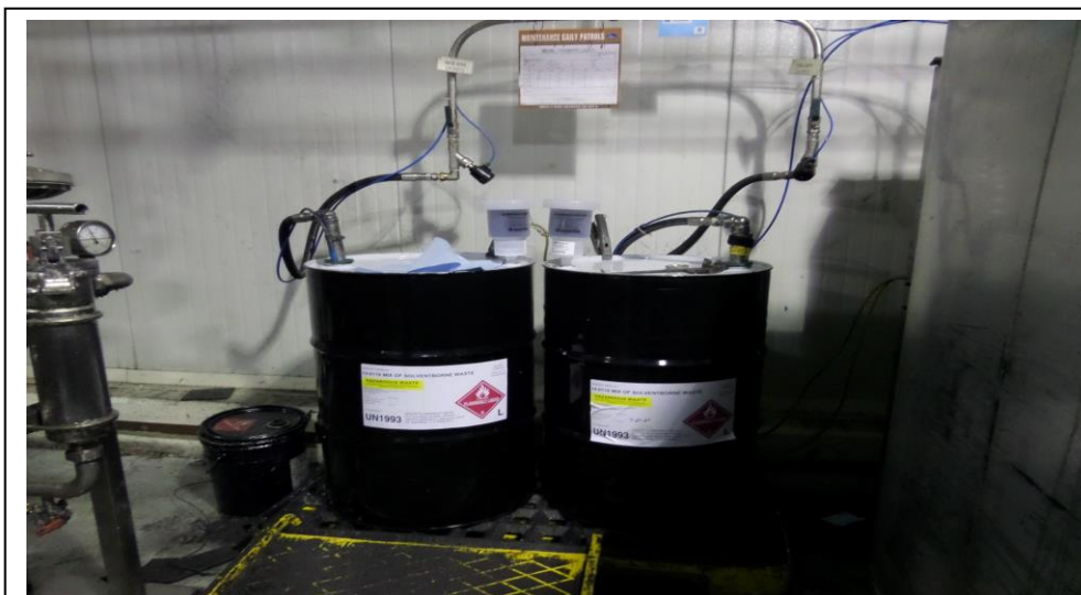
Hyundai. Purge Recovery 90-Day Area. Inspectors observed two 55-gallon containers accumulating solvent-borne waste from the two 35-gallon “Kettle” Purge Tanks. The containers were marked with dates in July 2021. Photograph 6 taken July 26, 2021 at 3:20 p.m.
