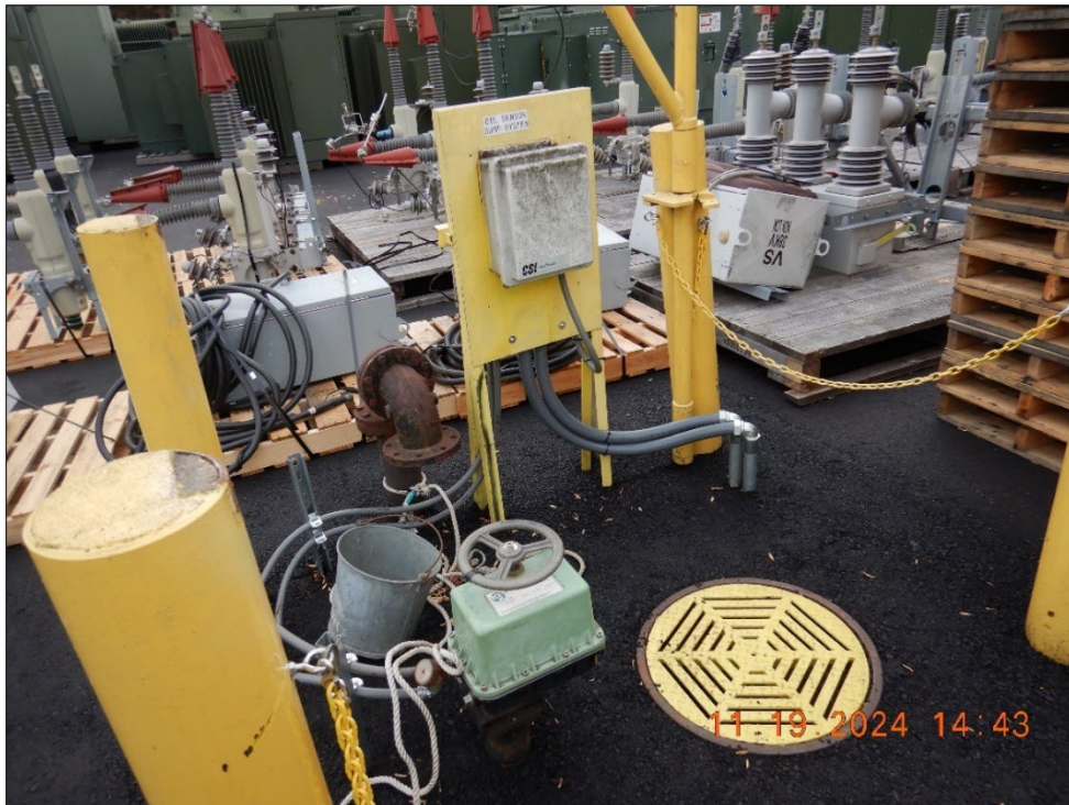
Photograph 14. DSCN0610.JPG View of the oil sensor sump system located upgradient of Outfall 001. The system is equipped with a conductivity sensor, automatic valve actuator, and spill containment vault to divert stormwater containing oil prior to discharge via Outfall 001.
