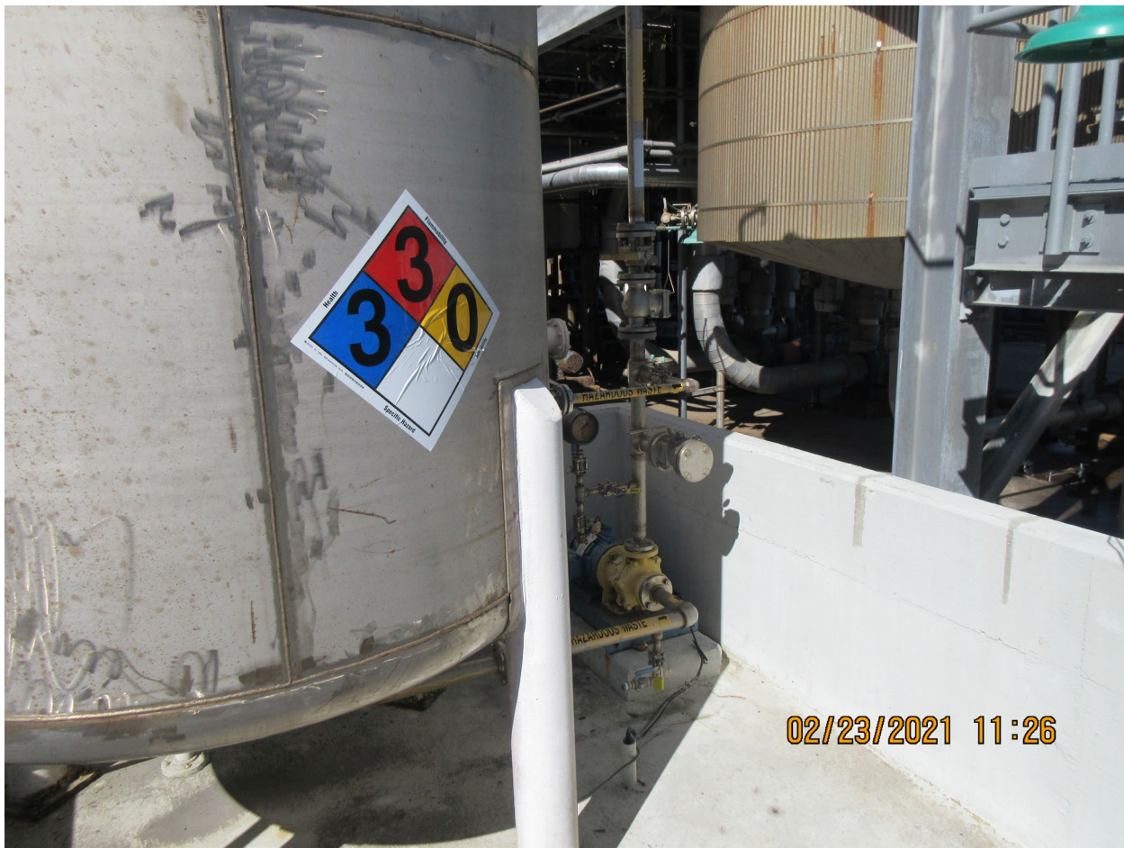
Photo 4 – Ancillary equipment for Tank-830
