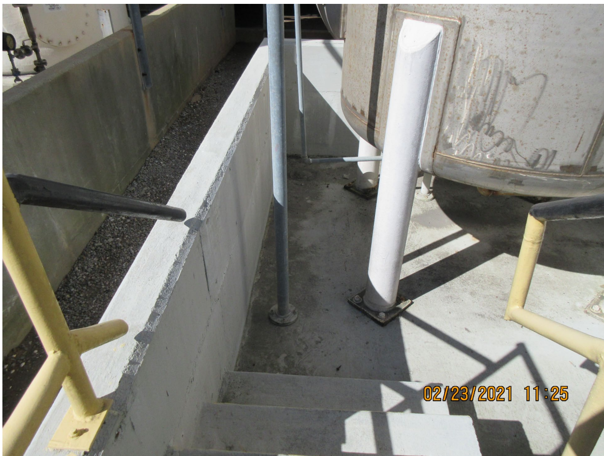
Photo 2 – Secondary Containment for Tank-830
