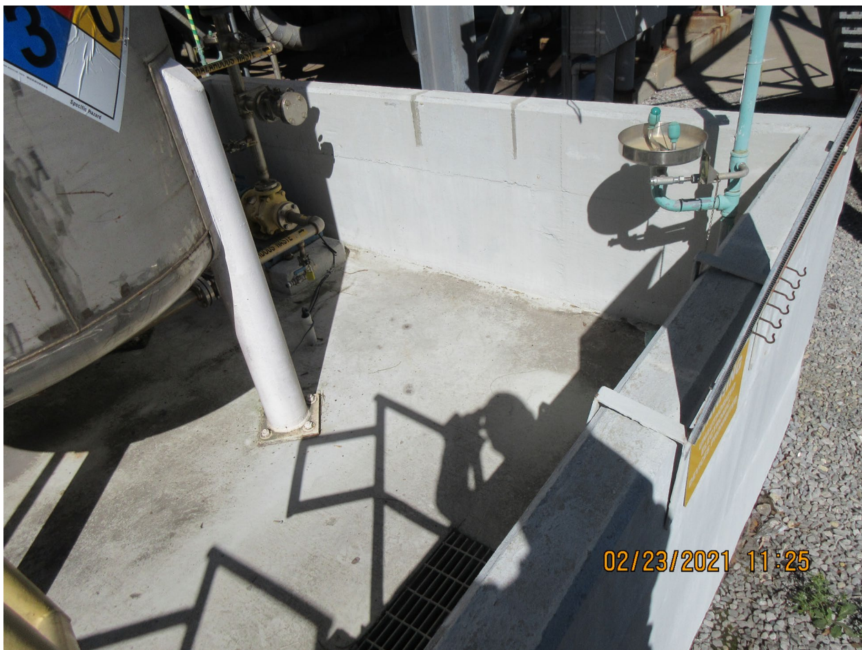
Photo 3 – Secondary containment for Tank-830
